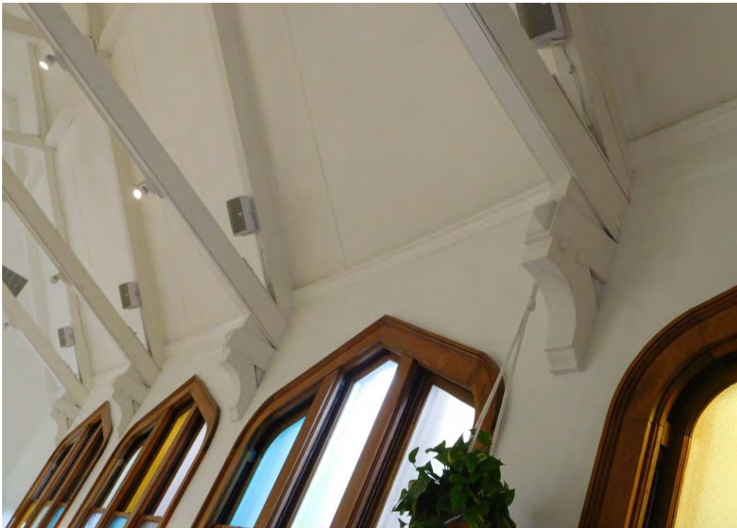
Figure 36. Corbels supporting the scissors trusses inside the former sanctuary; view toward southwest.
