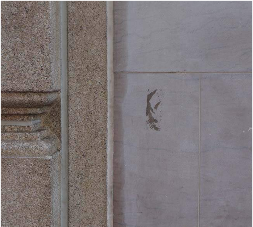
Hearst Building – Minor residue at marble podium
