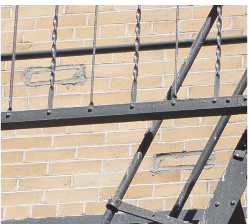
17-29 Third Street - Limited locations of mismatched mortar
