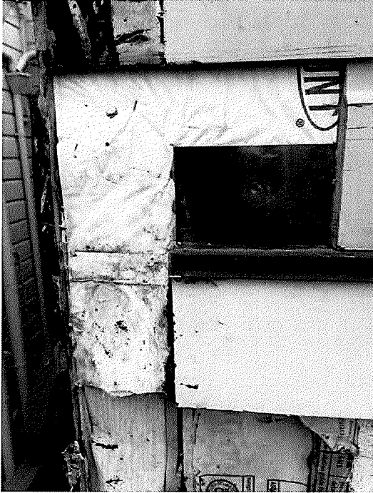
Photo A: Prior condition. Deteriorated sealing.
