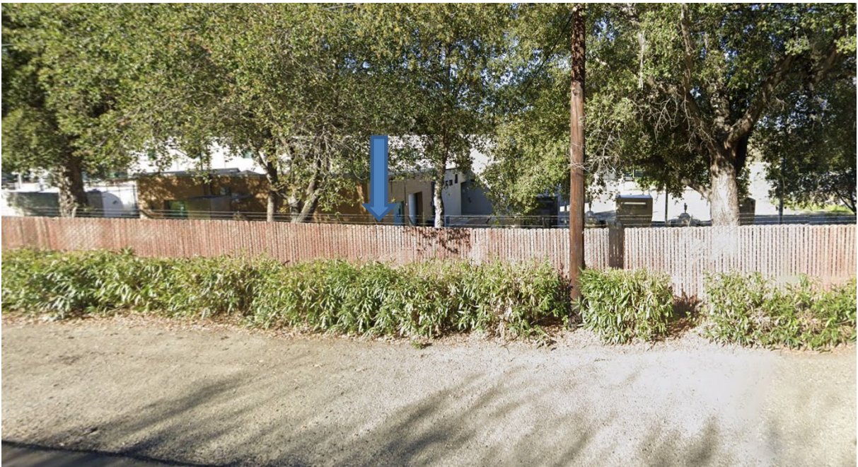
Figure 11: View from Calaveras Road Looking West Toward Approximate Location of the Power Factor Correction Capacitor Equipment Panel (Indicated by Blue Arrow) at the San Antonio Pump Station
