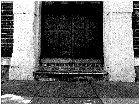
Figure 89 Detail view of entrance bay along Front Street. Note biological activity on brick coursework (photograph taken on 03/30/2017).
