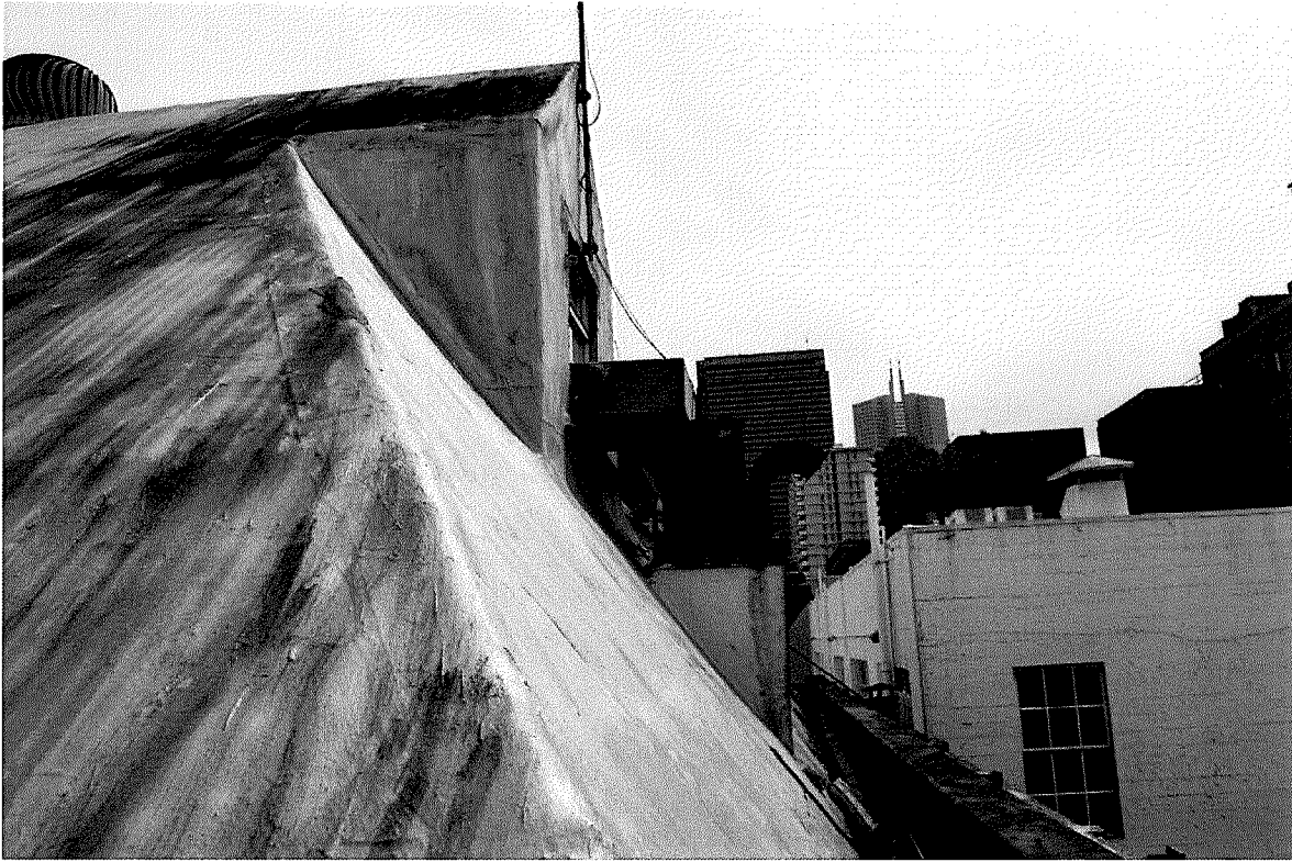
Figure 134 Photograph of western side of roof. Note mechanical equipment ran through the window opening (photograph taken on 04/05/2017).
