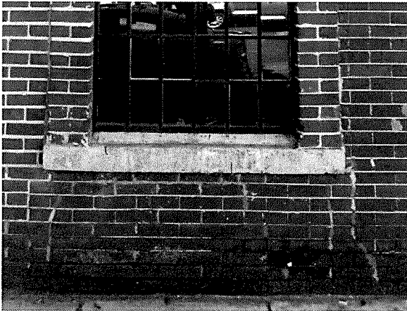
Figure 32 Detail of biological colonization plaguing mortar joints at the bottom courses along Vallejo Street (photography taken on 03/31/2017).
