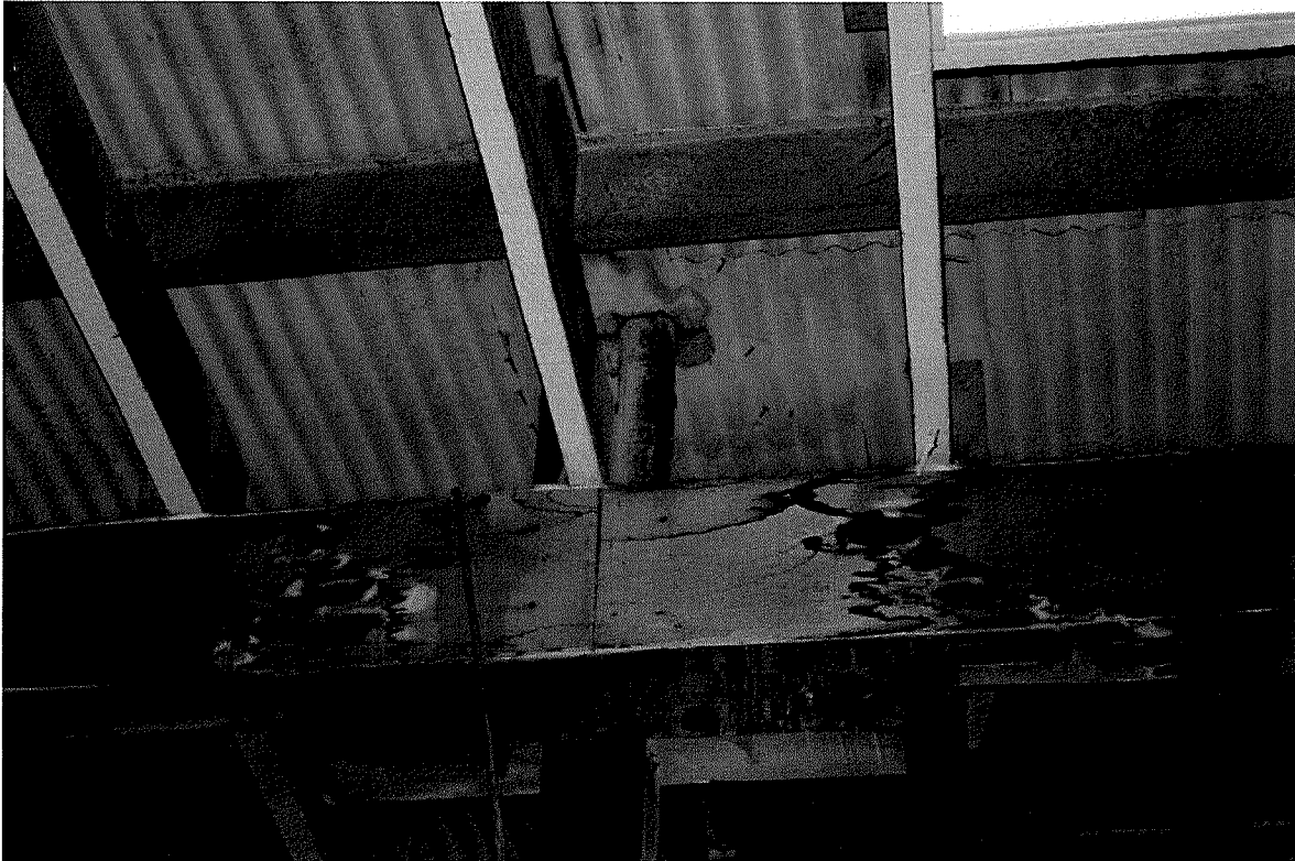
Figure 82 Detail of roof to beam construction. Note water staining and efflorescence on wooden members (photography taken on 04/04/2017).
