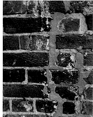
Figure 66 Detail of figure 64. Note cracking of brick adjacent to Portland cement repair (photography taken on 04/10/2017).
