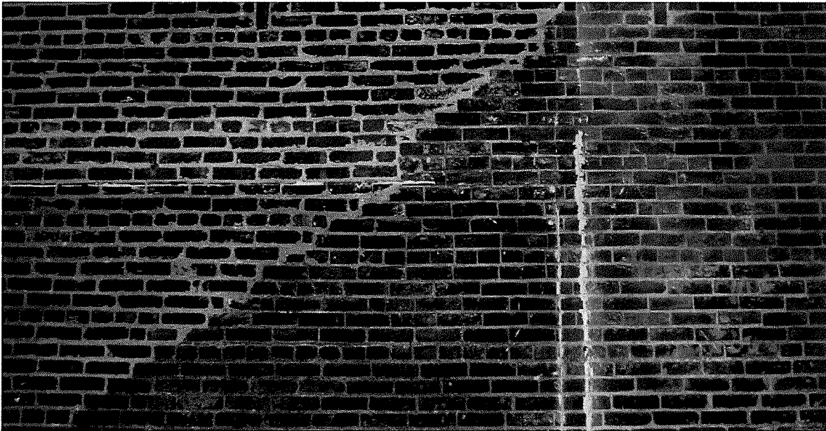
Figure 67 Photograph of south wall at the ground level. Note distinctively different eras of brick and mortar (photography taken on 04/04/2017).
