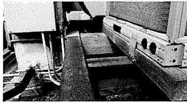
Figure 41 Detail photograph of structural support for HVAC and systems (photography taken on 04/05/2017).
