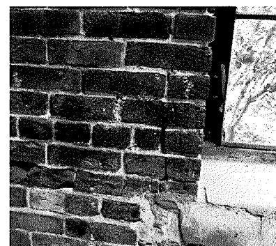
Figure 86 Detail of typical brick condition for deteriorated bricks around window openings (photography taken on 04/04/2017).
