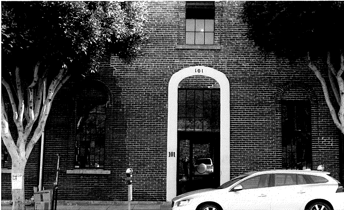
Figure 27 Photograph of 101 Vallejo Street. Note visual seam between historic brick (left) and the brick used in a later restoration campaign (right). Photography was taken on 03/30/2017.
