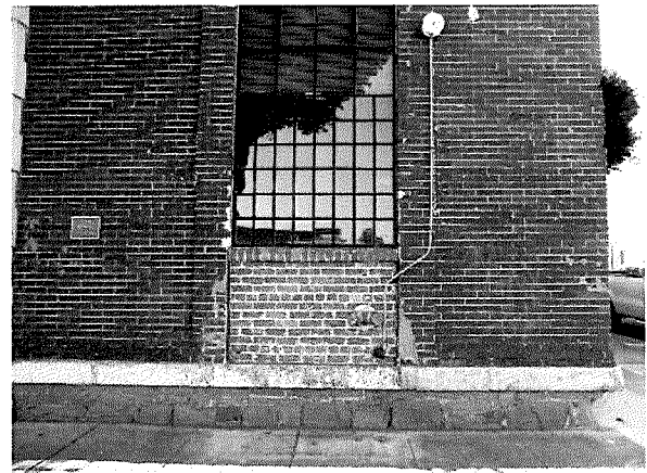
Figure 90 Photograph of the Front Street elevation. Note construction technique, paint remnants on watertable, and exposed foundation (photograph taken on 03/30/2017).
