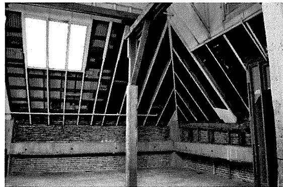
Figure 123 Interior photograph of structural system in the foreground and underside of the steep-pitched roof (photograph taken on 04/04/2017).
