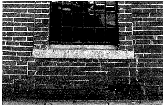
Figure 29 Detail of biological colonization at the bottom courses along Vallejo Street (photography taken on 03/31/2017).
