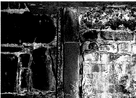
Figure 74 Detail of the intersection of the brick vault and foundation stone. Note iron staining and efflorescence (photography taken on 04/05/2017).
