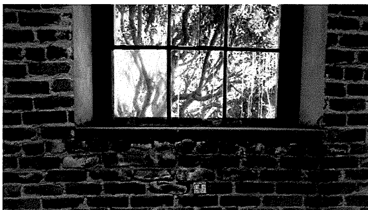
Figure 85 Detail photograph of southernmost window on the east wall. Note occurrence of efflorescence and eroded mortar (photography taken on 04/04/2017).
