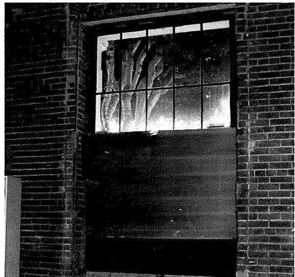
Figure 114 Interior photograph of entrance door along Front Street. Note extensive cracking of the brick and mortar surround the opening (photograph taken on 04/04/2017).
