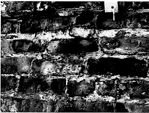
Photo 9: Deterioration in mortar joints of brick wall below gutter.
