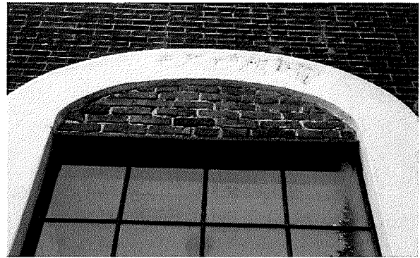
Figure 20 Detail of blind arch at westernmost entrance along Vallejo Street. Note the loss of concrete plaster and the raised metal rebar. Condition is also observed at the 101 Vallejo entrance (photography taken on 03/30/2017).
