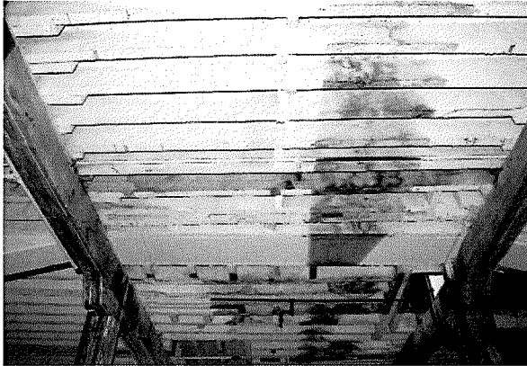
Figure 103 Photograph of ground floor ceiling joists. Note ghosts from old HVAC and water staining (photograph taken on 04/04/2017).
