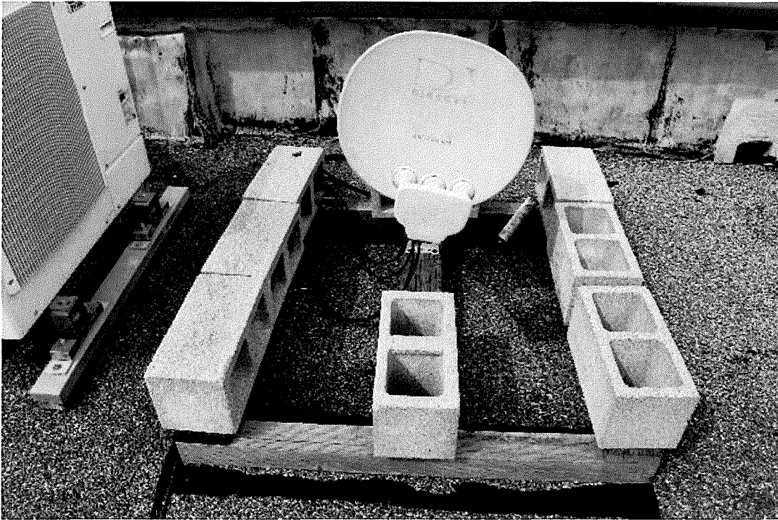
Figure 136 Detail of satellite dish installation. Note use of cinderblocks to weigh down nominally cut wood (cinderblocks are not anchored to the roof). Photograph was taken on 04/05/2017.
