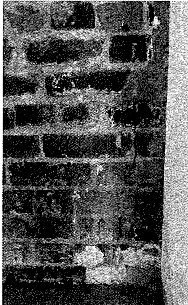
Figure 63 Detail of Portland cement patch and subsequent crack as a result (photography taken on 04/10/2017).
