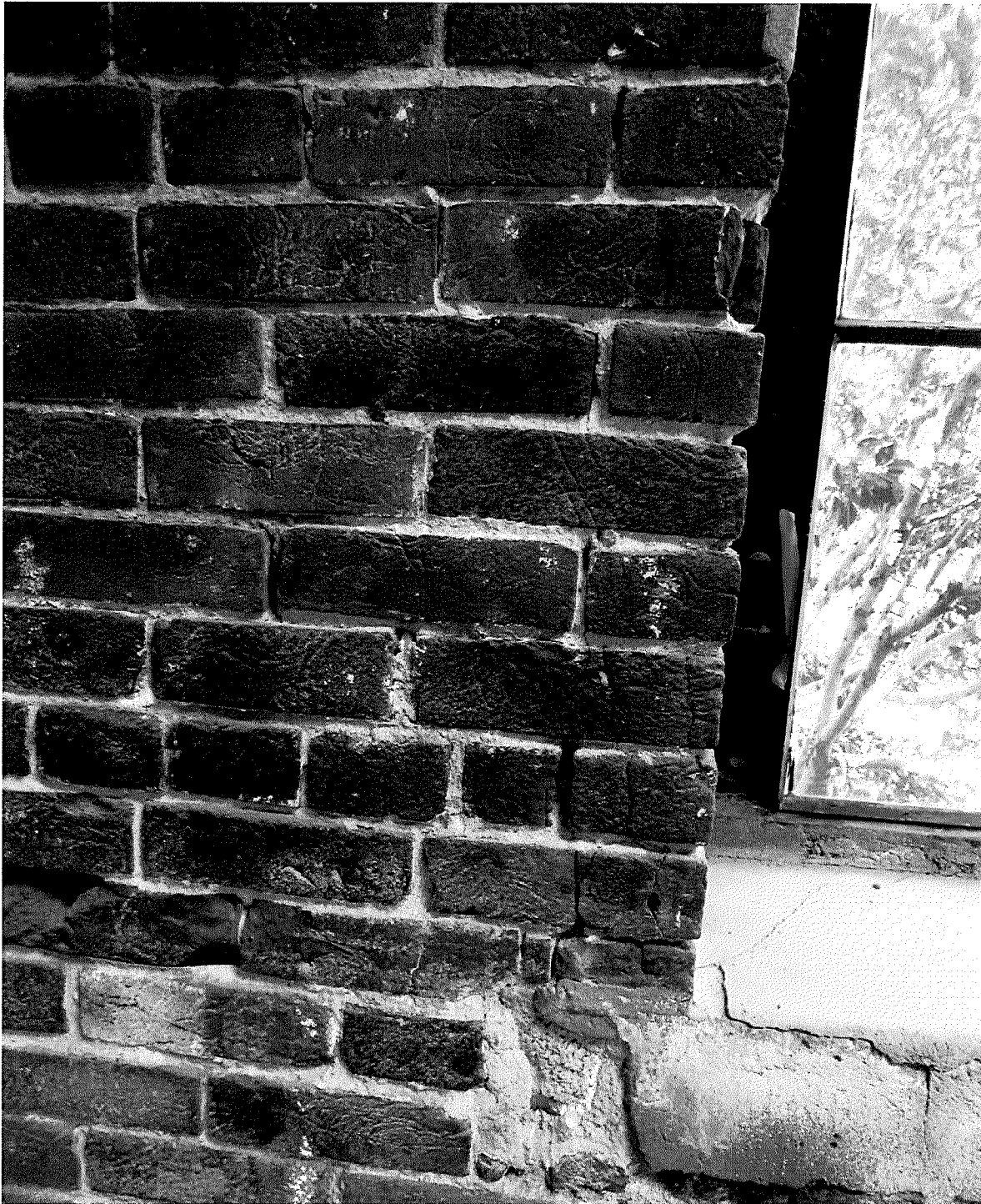
Figure 133 Typical condition of cracked bricks around window openings (photograph taken on 04/10/2017).
