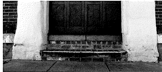
Figure 9 Detail view of entryway. Note brick stairs and biological growth (photography taken on 03/30/2017).
