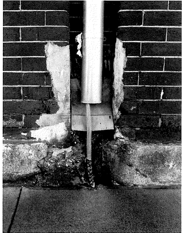
Figure 101 Detail of broken downspout along Vallejo Street. Note bio-colonization on stone, brick, and mortar (photograph taken on 04/04/2017).
