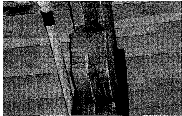
Figure 108 Interior detail of structural timber construction. Note split in capital (photograph taken on 04/10/2017).
