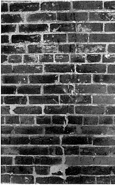
Figure 62 Detail of a crack propagated by a Portland cement repair. Crack originates at the Portland cement infill and runs the height of the wall (photography taken on 04/10/2017).
