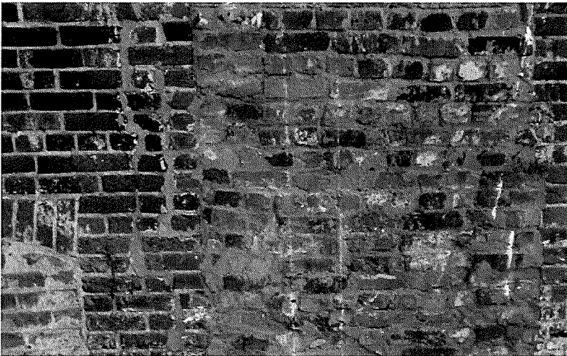
Figure 65 Detail photograph of historic window filled-in with brick on the east wall. There are 4 similar conditions on this elevation (photography taken on 04/10/2017).
