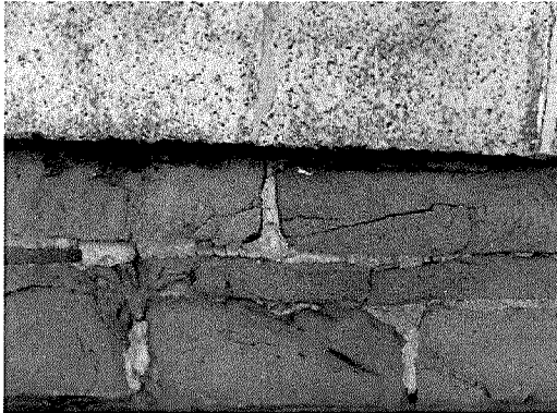
Figure 5 Detail view of foundation stone condition. Note cracking, fragmentation, insipient spalling, and failed mortar joints (photograph taken on 03/31/2017).
