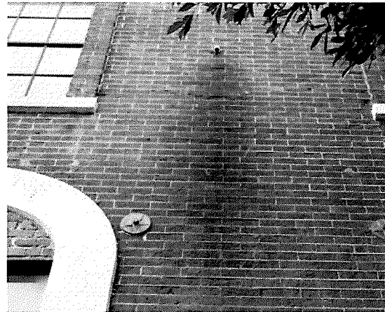
Figure 35 Non-functioning downspout along Vallejo Street. The inability to direct water away from the facade and foundation have resulted in heavy areas of bio-colonization. This will, in turn, accelerate the deterioration of the brick and mortar (photography taken on 03/31/2017).
