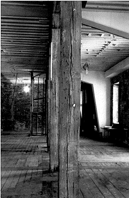
Figure 58 Interior photograph of vertical splitting present in several of the structural timber columns on the ground floor (photography taken on 04/10/2017).
