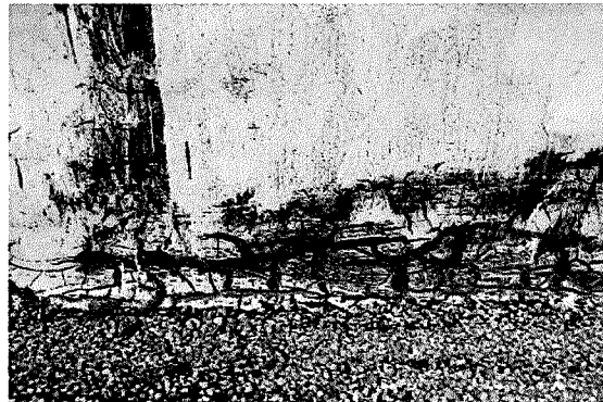
Figure 54 Detail at base of north parapet wall. Note cracking tar and paint (photography taken on 04/04/2017).
