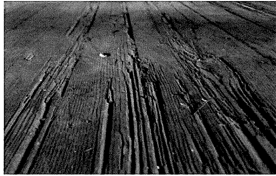
Figure 61 Detail photograph of floor condition on the ground floor level (photography taken on 04/05/2017).
