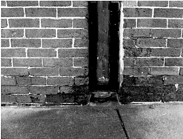
Figure 34 Non-functioning downspout along Vallejo Street. The inability to direct water away from the facade and foundation have resulted in heavy areas of bio-colonization. This will, in turn, accelerate the deterioration of the brick and mortar (photography taken on 03/31/2017).
