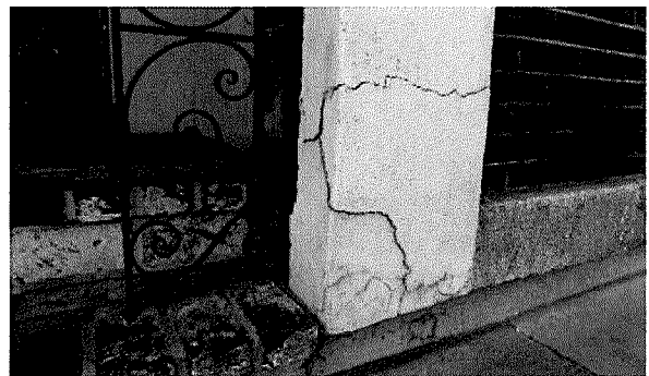
Figure 21 Detail photograph of cracked and spalling cement plaster (photography taken on 03/31/2017).
