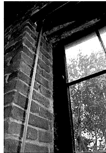
Figure 130 Detail photograph of window hardware on the second floor. Same window as previous two images. This is believed to be the earliest construction type found for the windows (photograph taken on 04/04/2017).
