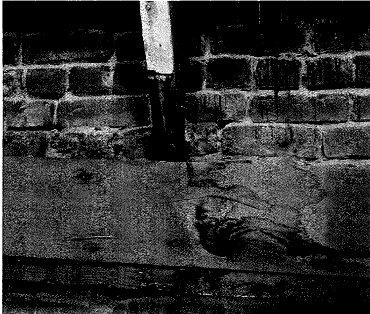
Figure 126 Detail view of rafter-to-masonry construction at the upper level. Note deteriorated mortar joints, efflorescence, and iron staining (photograph taken on 04/04/2017).
