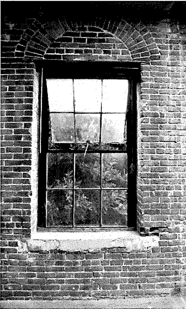
Figure 125 Interior photograph of typical deterioration around window opening (photograph taken on 04/04/2017).
