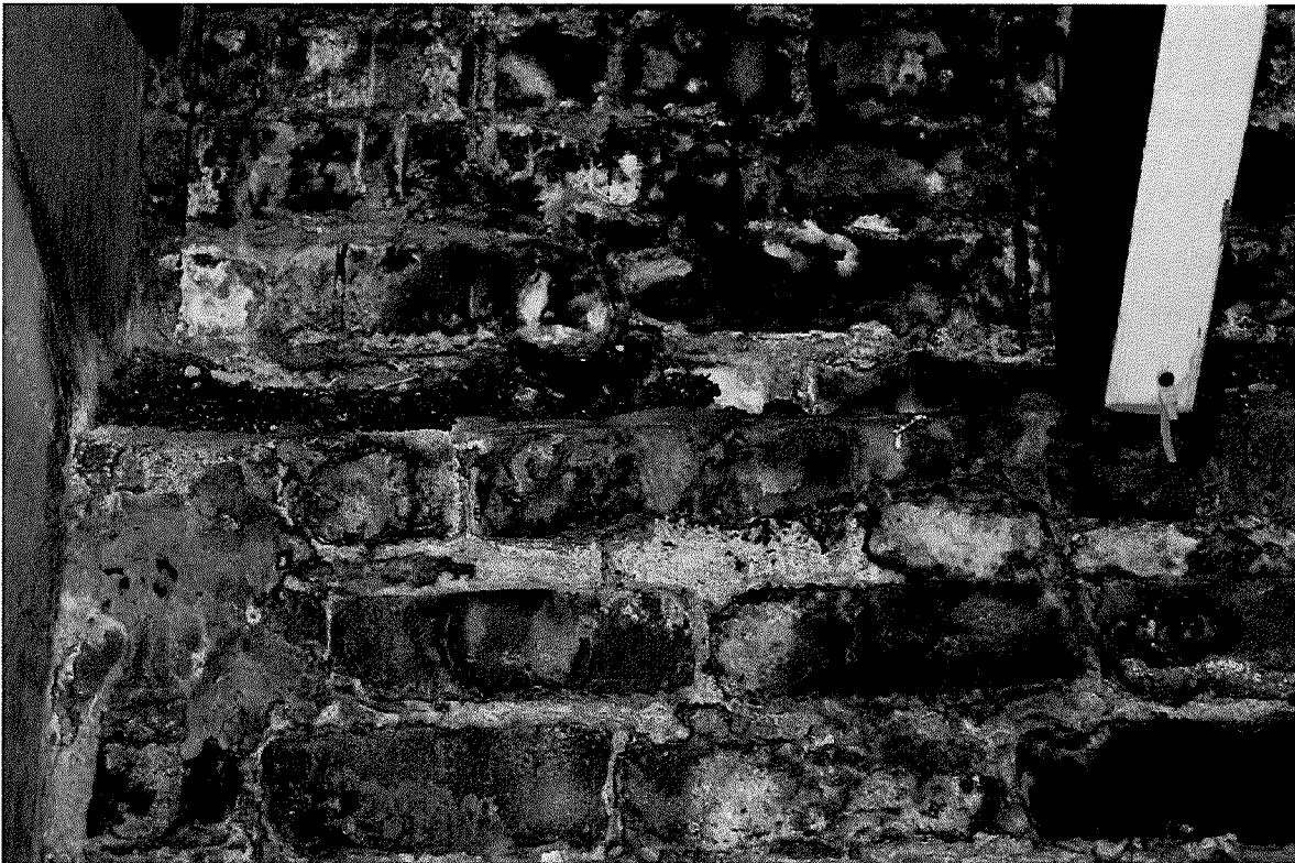
Figure 83 Detail photograph of interior upper brick courses, just below roofline. Note extensive efflorescence and discoloration. The corrosion colored staining is a leaching of ferruginous mineral inclusions innate in the brick and/or mortar (photography taken on 04/04/2017).
