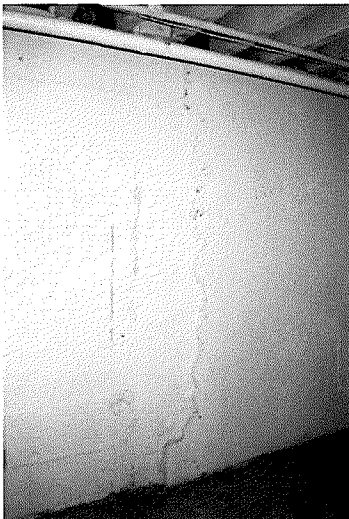
Figure 77 Photograph of north foundation. Note cement repairs over a masonry substrate (photography taken on 04/04/2017).
