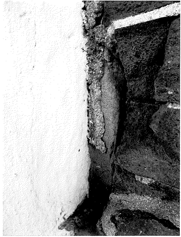
Figure 92 Photograph of entrance threshold at Front Street elevation. Note sandstone substrate (photograph taken on 03/31/2017).
