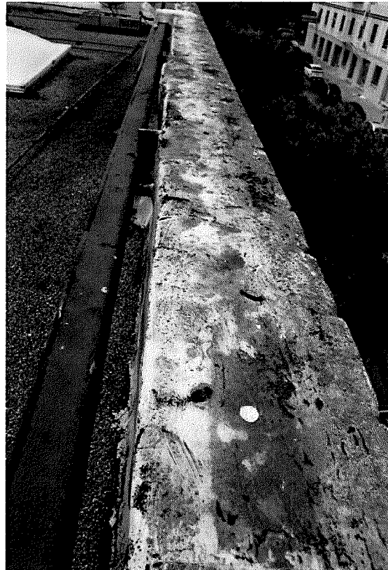
Figure 52 Photograph of horizontal surface on east parapet. Note biological-colonization, corrosion, atmospheric soiling, and minor animal deposits (photography taken on 04/04/2017).
