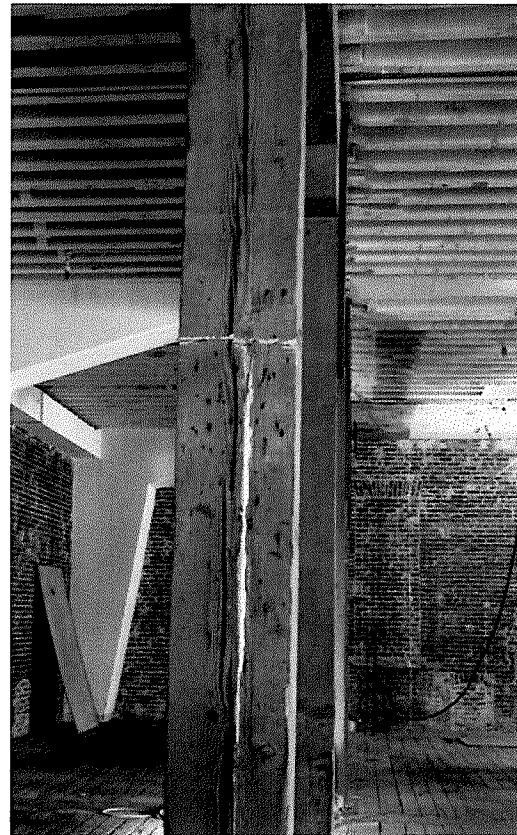
Figure 59 Interior photograph of vertical splitting present in several of the structural timber columns on the ground floor (photography taken on 04/05/2017).
