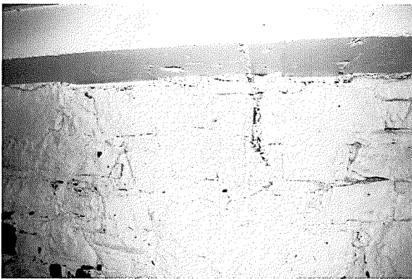
Figure 117 Detail view of south foundation wall. Note irregularly-cut and laid fieldstone (photograph taken on 04/04/2017).
