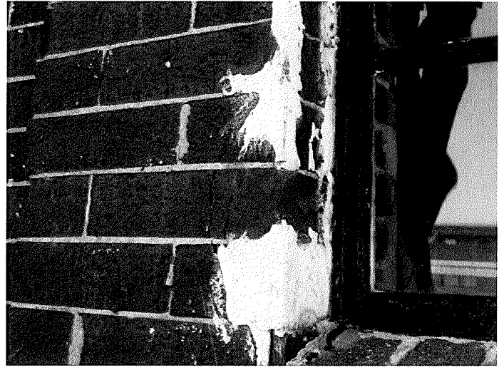
Figure 14 Detail of inappropriate repair material used on the brick façade (photography taken on 03/30/2017).
