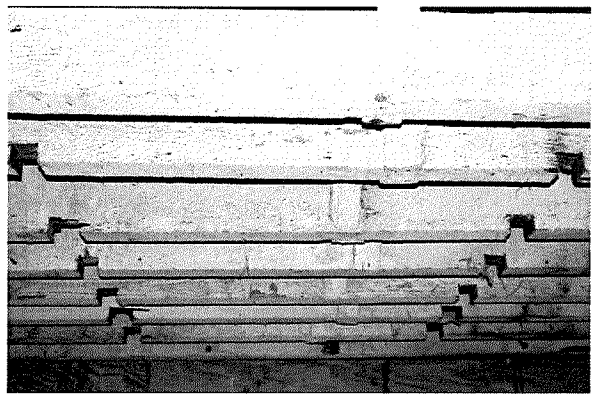
Figure 118 Interior photograph of the ceiling joists at the basement level (photograph taken on 04/04/2017).
