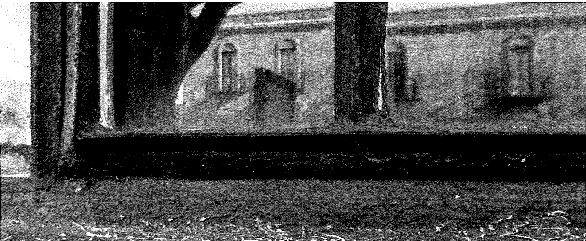
Figure 26 Detail of localized corrosion and window sash failure. Instances are few, however, need repair/rehabilitation (photography taken on 03/31/2017).
