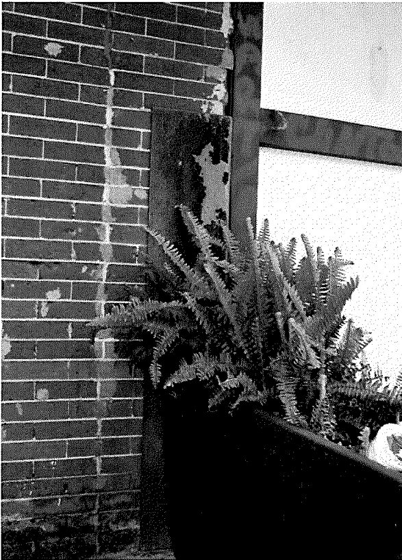
Figure 100 Photograph of steel reinforcement on the northwestern corner of the building (photograph taken on 04/04/2017).
