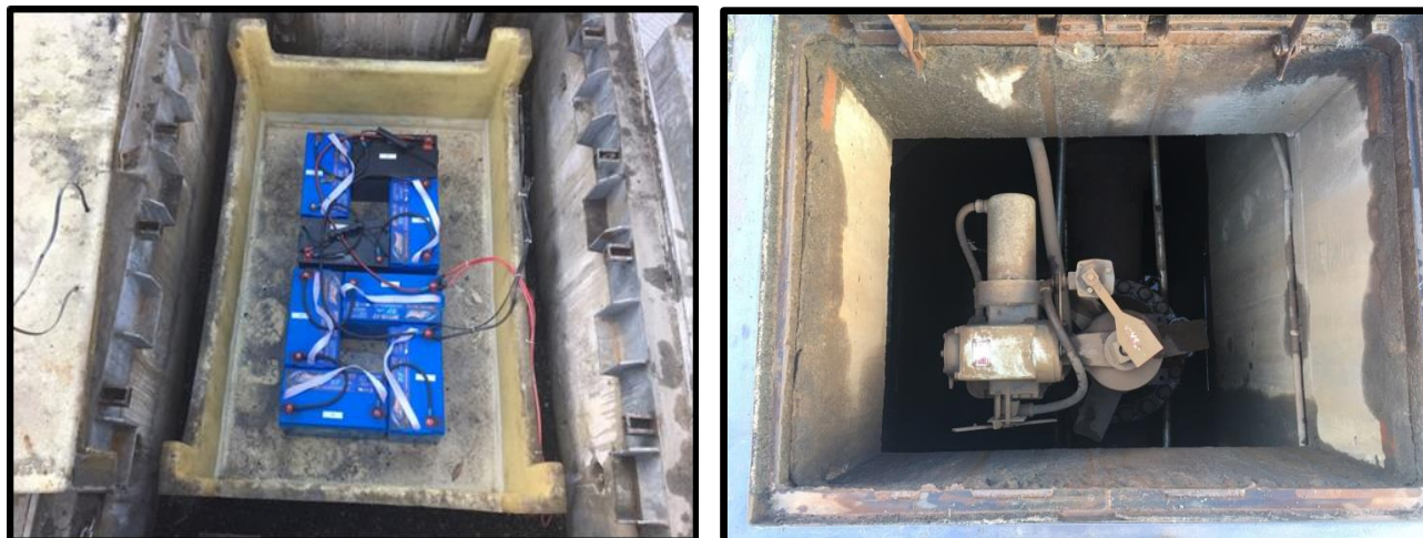
Figure 3 Seismic Actuated Valve and Battery System (Source: SFPUC)
