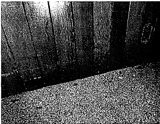
Figure 13: Abrasion marks and soiling at base of wainscoting from pedestrian traffic.
