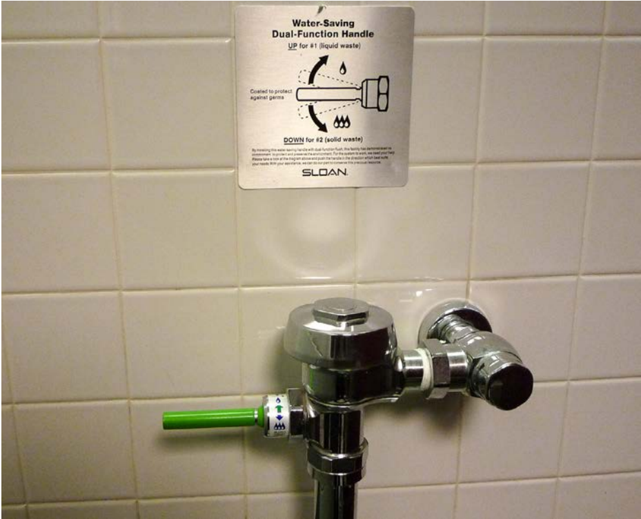
Dual flush toilets contribute to indoor water use reduction
