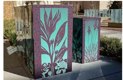
Utility infrastructure should be grouped, integrated with landscape, and can provide space for public art.
