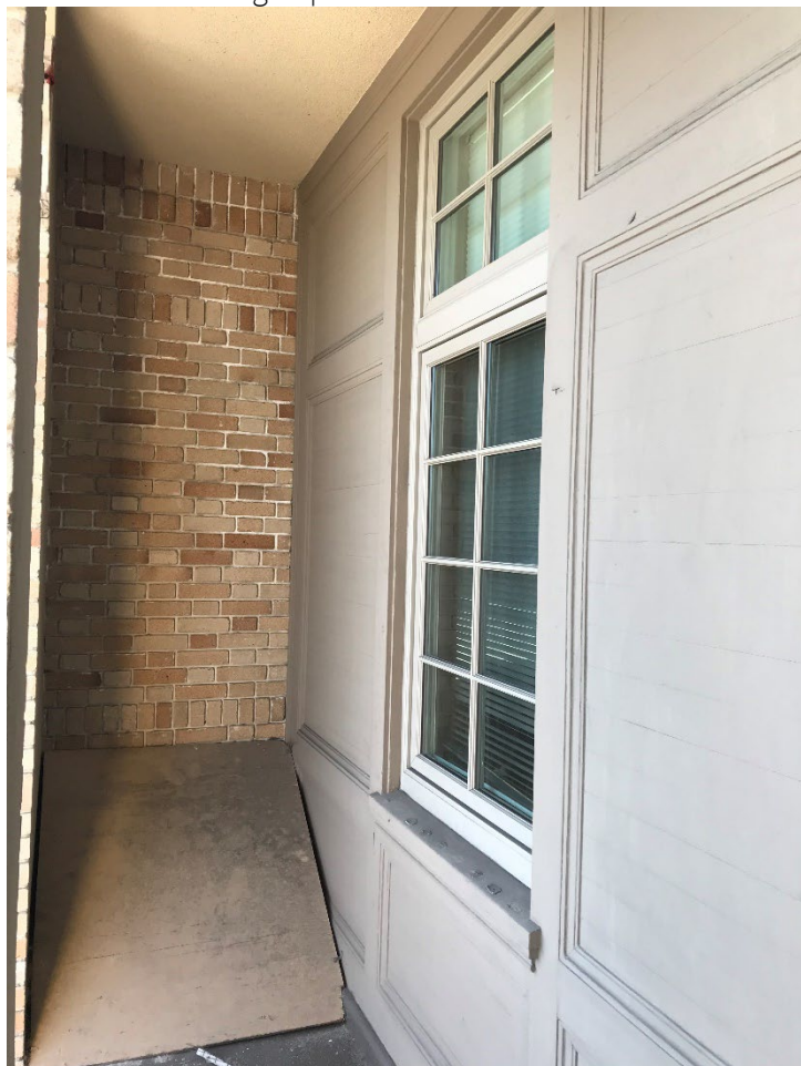
San Francisco Fire Station No. 44, detail of enclosed porch at Girard Street façade, view south, 2023. Source: SF Planning Department
