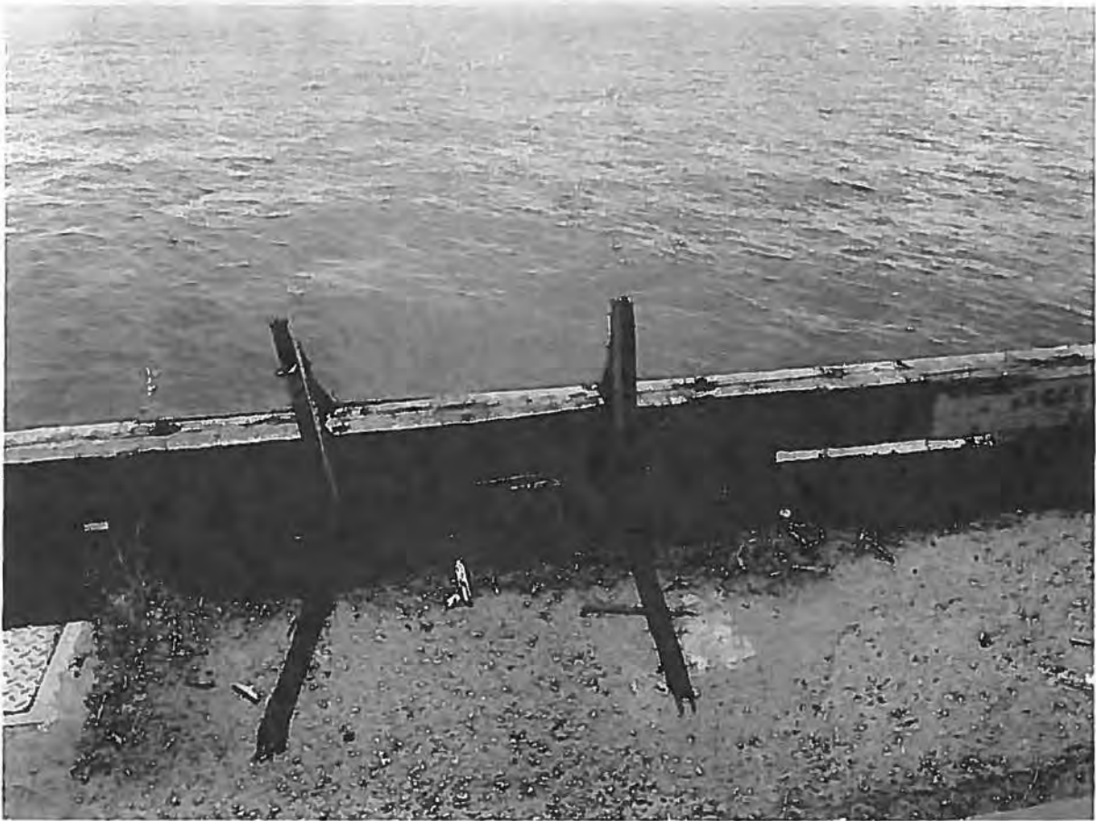
P80 C Face missing ships water service (Image #6)
