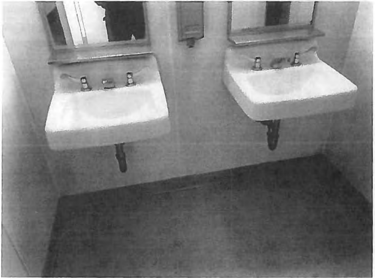
P80 C MRR sink faucets need rebuilding (Image #8)
