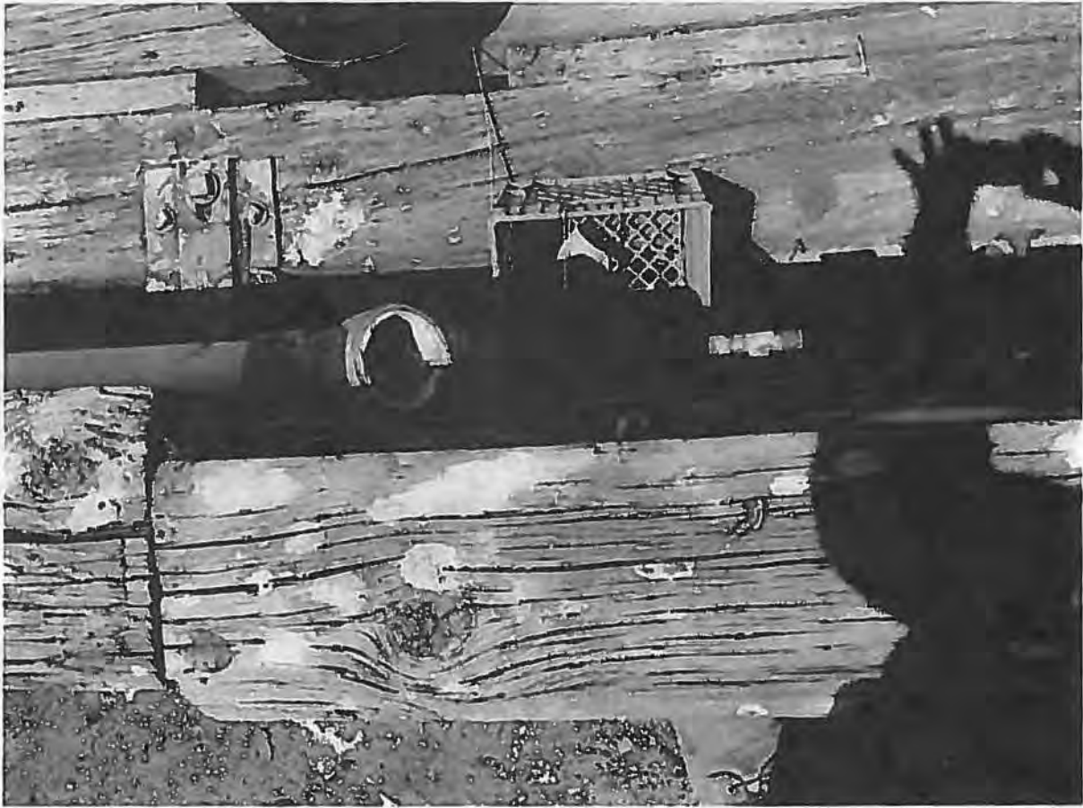
Forced Sewer Ship Connection on north side of P80, note that it is broken and unserviceable. (Image #4)
