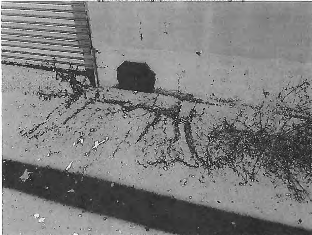
Photo 7. View of the ground settlement in the loading dock at the south side of the building
