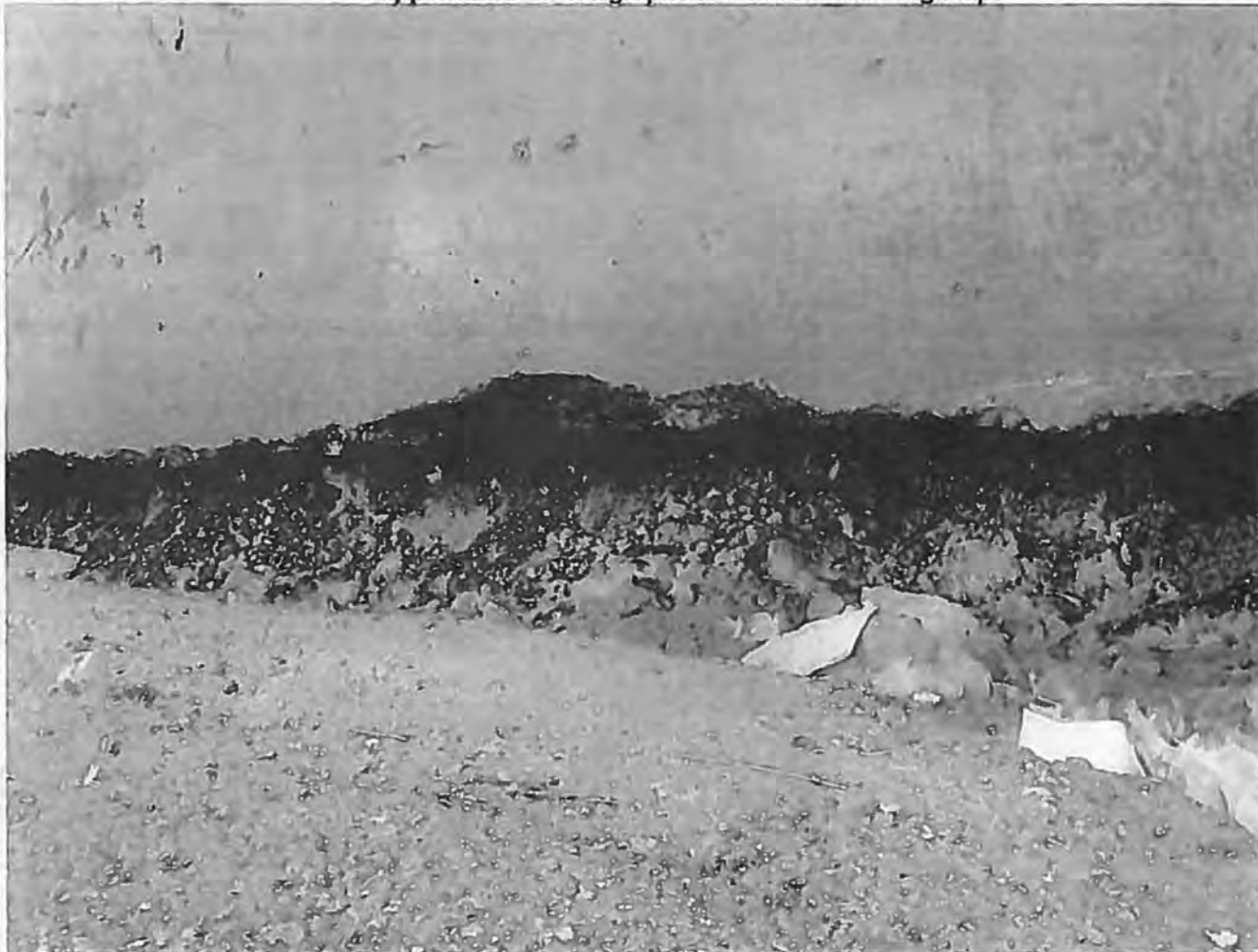
Photo 23. View of the settlement at the east side of the building
