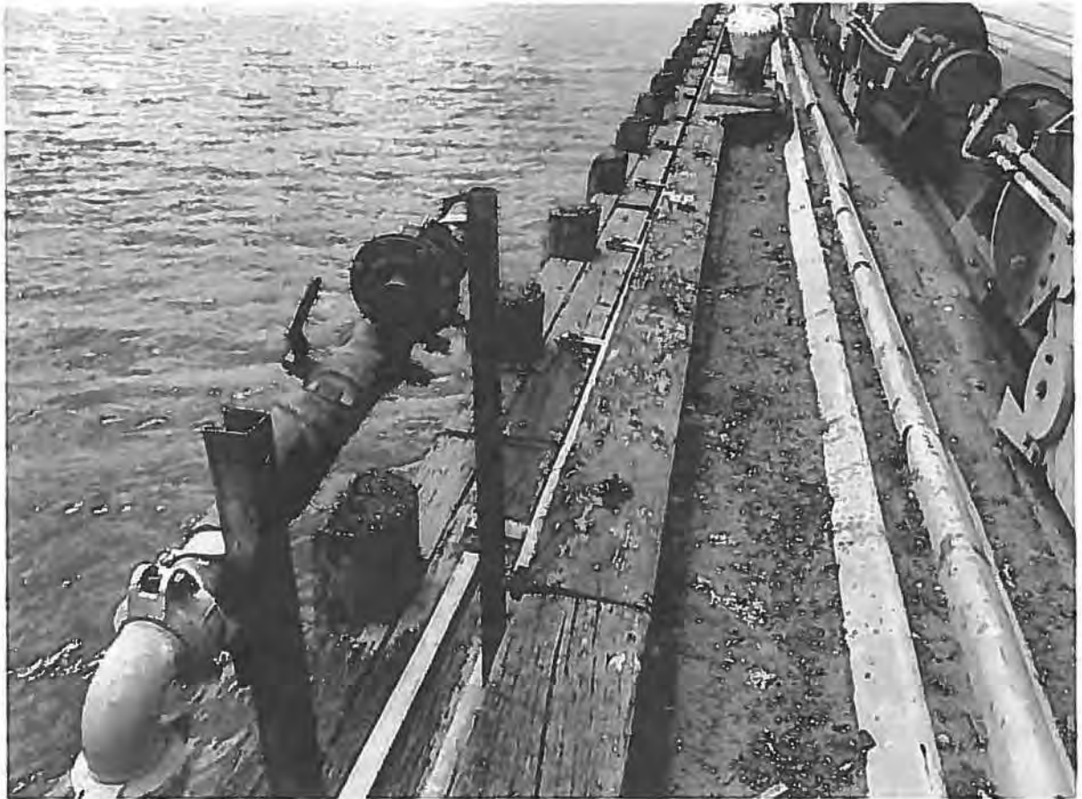
P80 B Face ships water service, note that it is upside down, and should not be operated this way.
