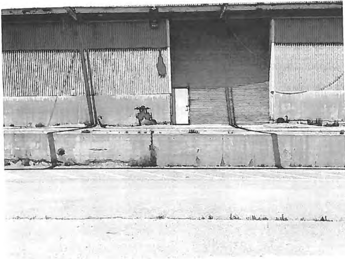
P80 A Shed Rain water liter dumping on loading dock, and fire department connection. (Image #1)
