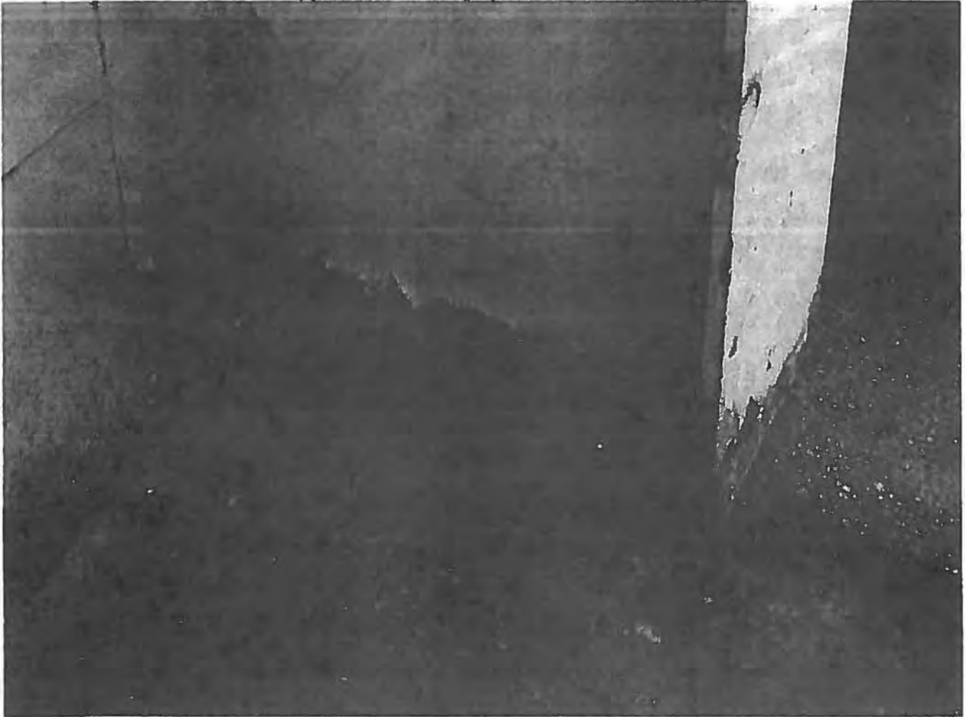
Photo 16. View of the steel column bases with corrosion and paint peeling
