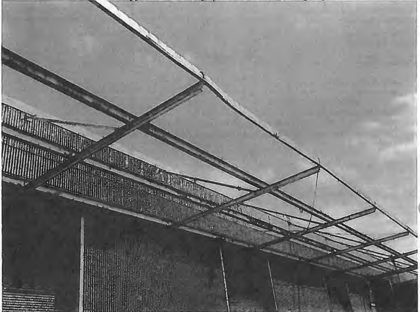
Photo 1. View of the south canopy structure with bent steel members and missing roof deck
