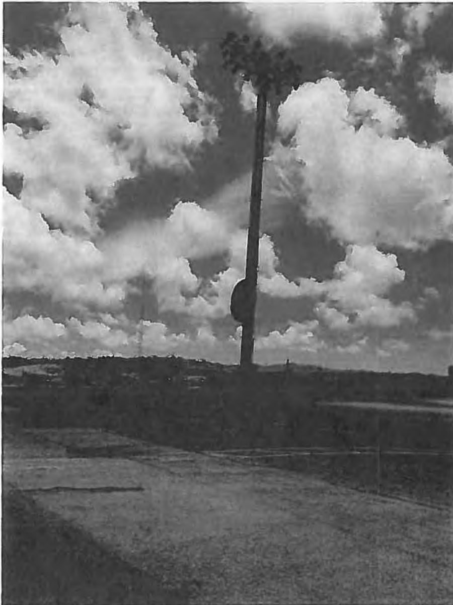
P80 C Face Main Yard light pole stand with sewer outfall vent pipe attached. Also there is a round sign saying that there is a submerged sewer outfall. The PUC is planning to paint these in the near future. (Image #12)
