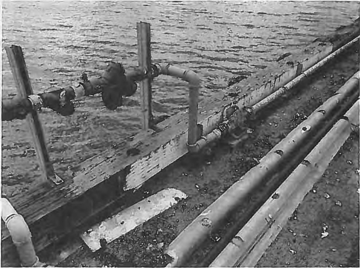
P80 B Face (west) backflow and SFWD maritime meter that feeds hose connection to the west. This was installed by America's Cup and should probably be shortened. (Image #14)
