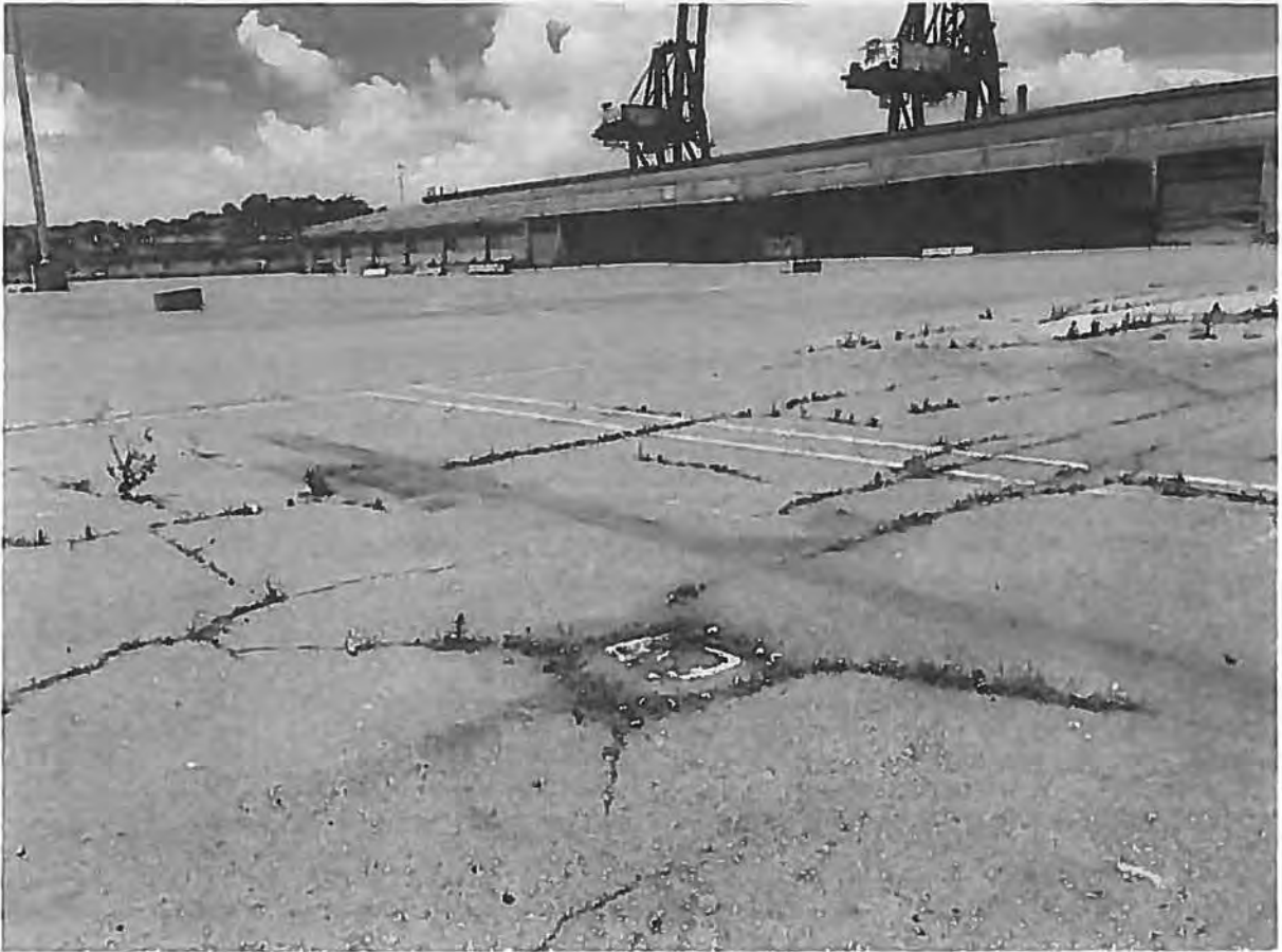
P80 Main Yard Center East: Yard valve to ships water services (Image #18)
