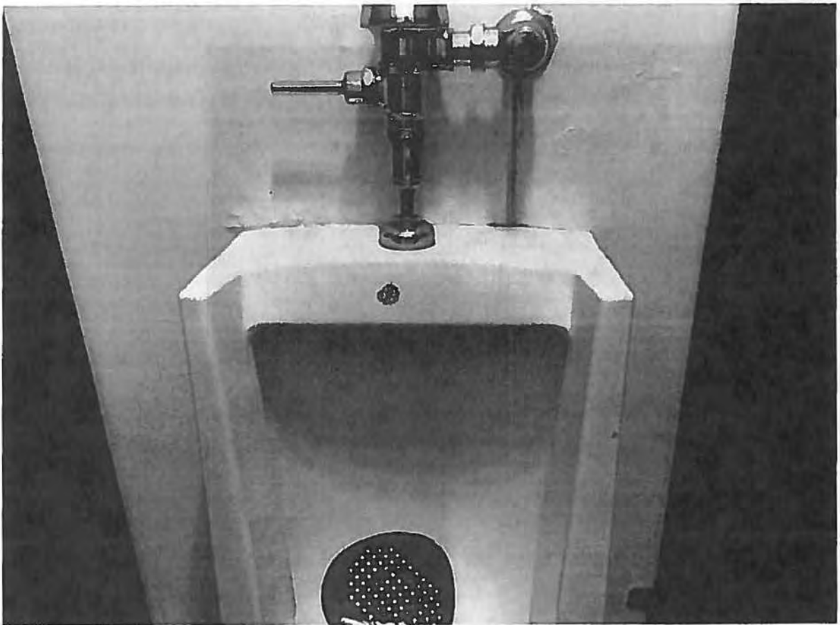
P80 M&R Building urinal leak behind wall (Image #22)
