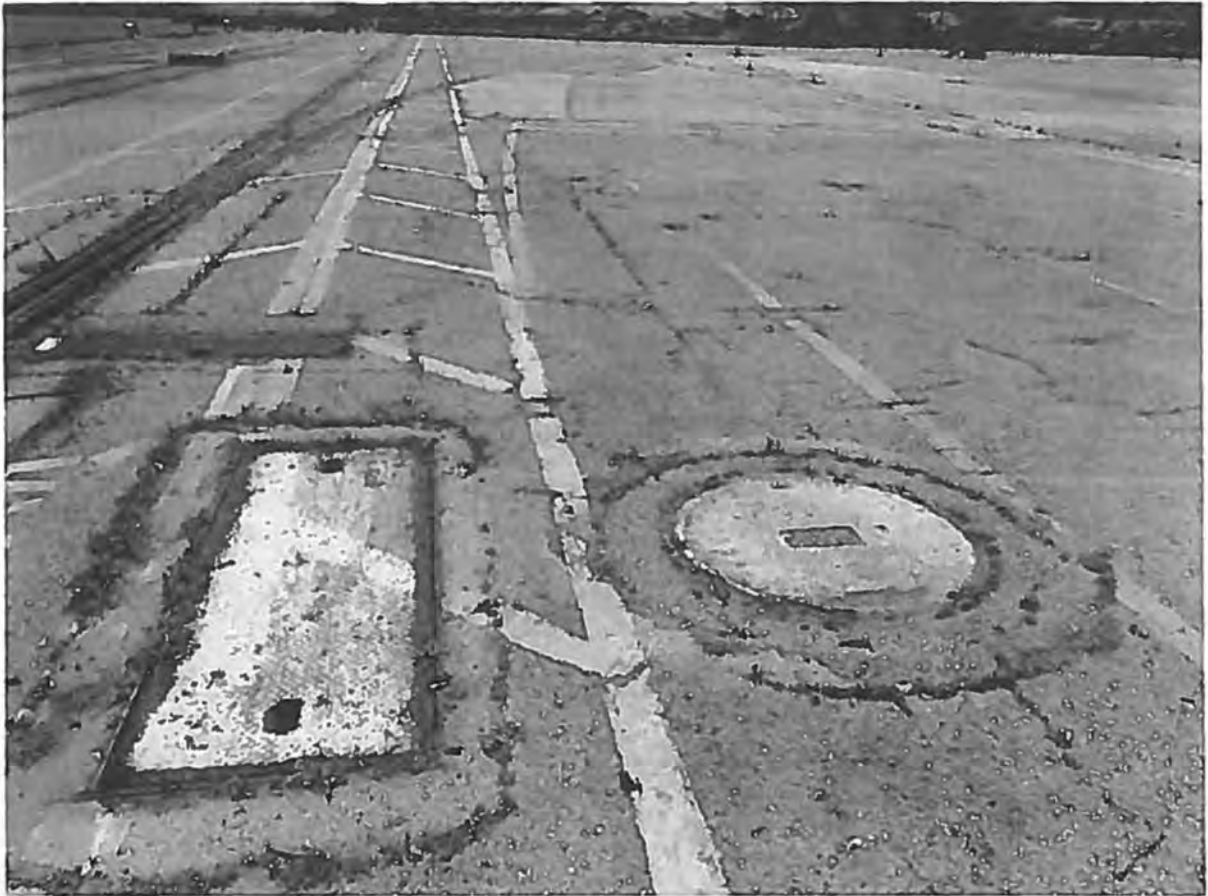
P80 C Face; PUC outfall from sewer treatment plant access manhole and gate valve (Image #11)
