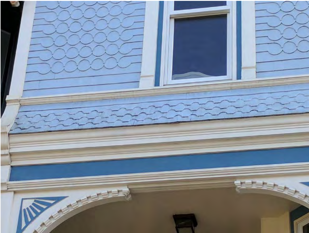
Cracked shingles to left of window near circular details:
