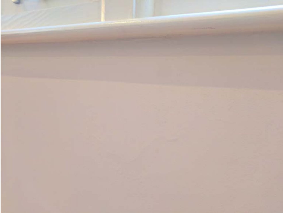
Photo B: Water damage adjacent to 2F kitchen
