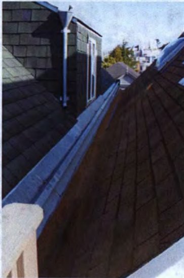
Figure 13: West roof gutter. Note water ponding locations
