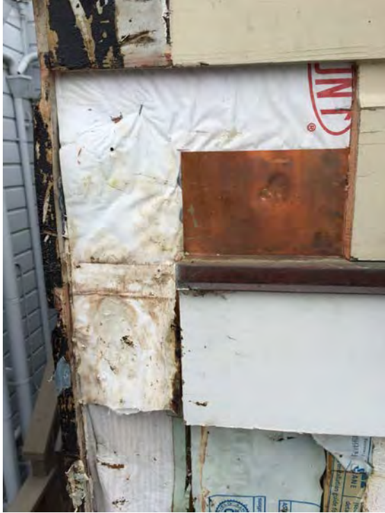
Photo A: Prior condition. Deteriorated sealing.
