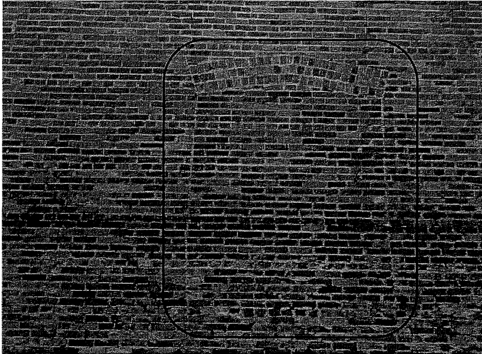
Figure 11: Segmental arch and mortar joints of former window openings along west façade remain visible. Looking east.
