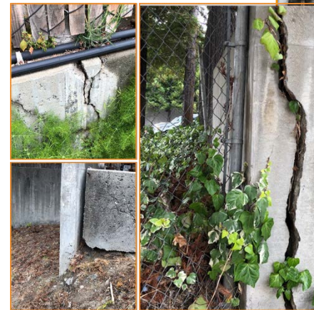
Cooling Tower foundation (above) structurally unstable.
