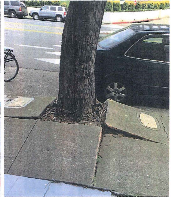
Sidewalk repair needs
