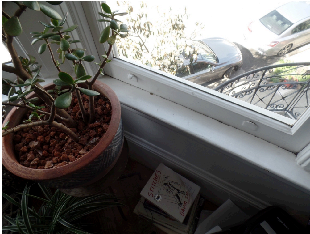
Figure 17: Interior view of front bay window in Unit 152A. Note deterioration at interior sill (Garavaglia Architecture, 2023).
