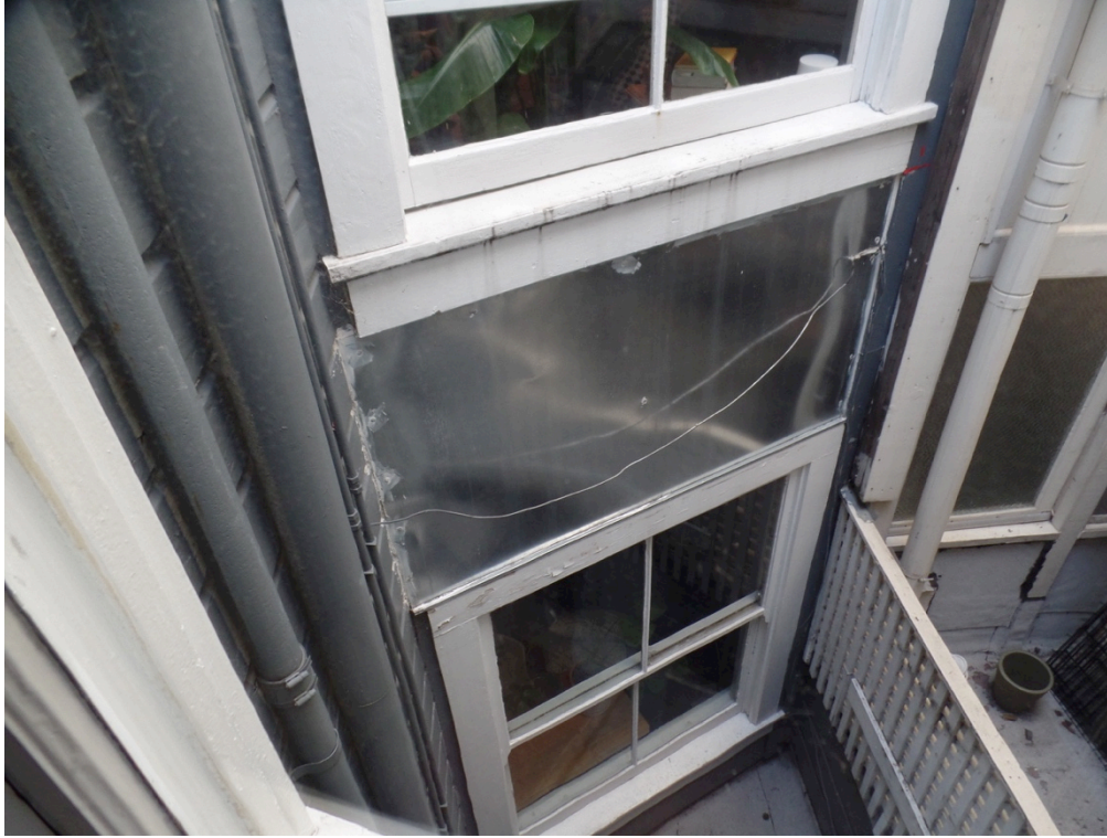
Figure 19: Interior view from Unit 152A looking down into south elevation window alcove. Note gap between sash and sill at upper window (Garavaglia Architecture, 2023).
