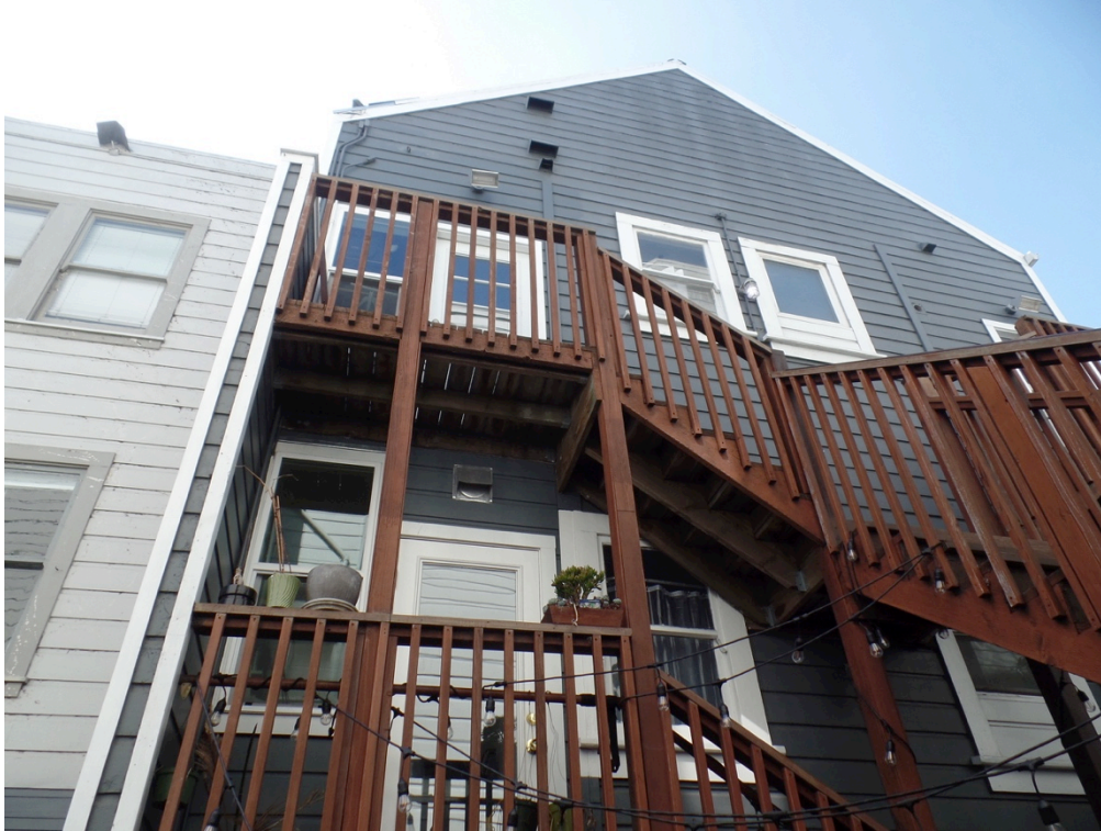
Figure 4: East elevation view of second and third levels and rear stairs (Garavaglia Architecture, 2022).
