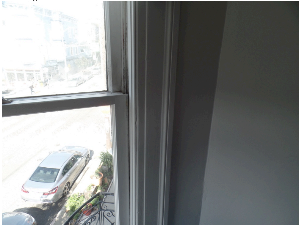
Figure 18: Interior view of front bay window in Unit 152A. Note damage at jamb and lower stile (Garavaglia Architecture, 2023).
