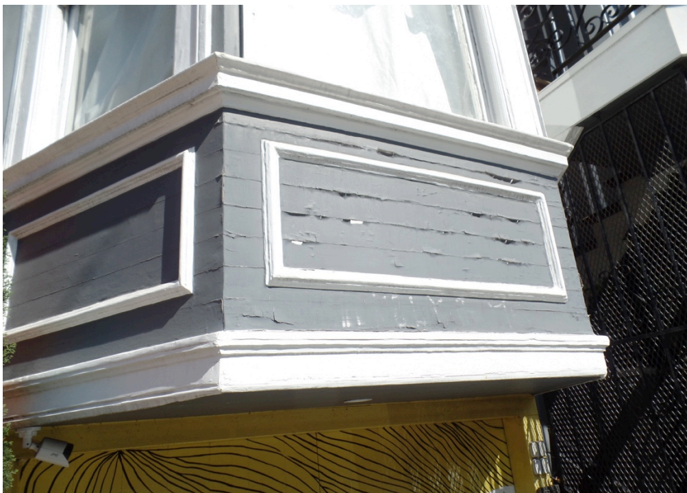
Figure 12: Front elevation view of peeling paint on bay window at second level (Garavaglia Architecture, 2022).
