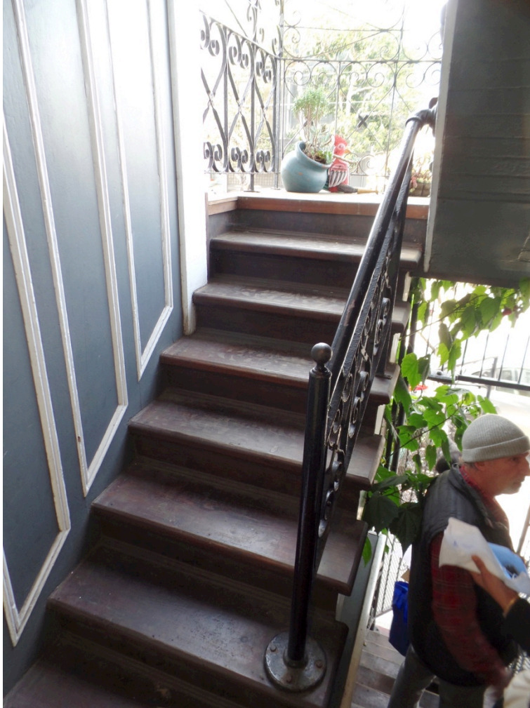
Figure 15: View of front entry stairs to third level. Note gap in baluster near landing (Garavaglia Architecture, 2023).
