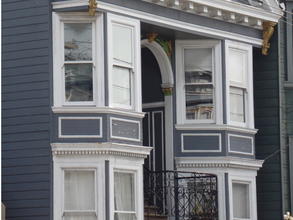
Figure 11: Front elevation view of peeling paint, worn wood elements at bay windows on third level (Garavaglia Architecture, 2023).
