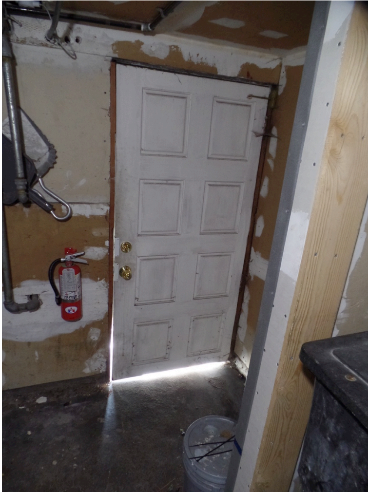
Figure 25: Interior view of 8-panel door to ground level on front elevation (Garavaglia Architecture, 2022).
