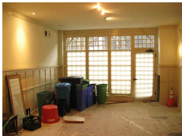
View north of the reception area, formerly used as a store at 2172 Market Street.
