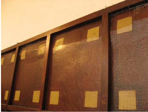
Detail of leather paper wall cladding. Note damage.
