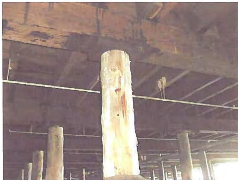
Photo 2: Fungus at Top Pile Section
