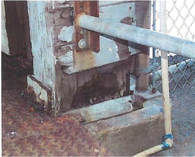
Photo 3: Damaged end wall column base
