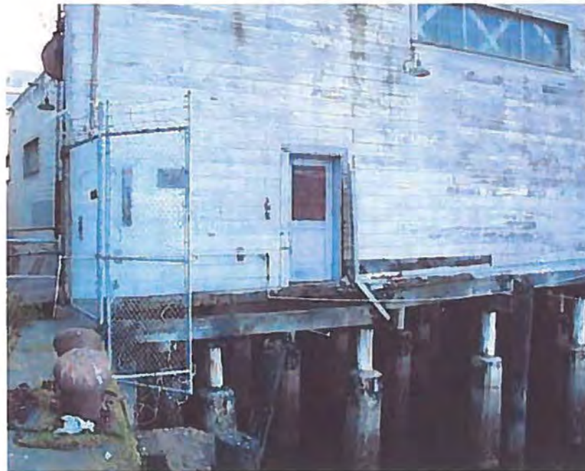
Photo 4: Mandoor exit with no exterior access
