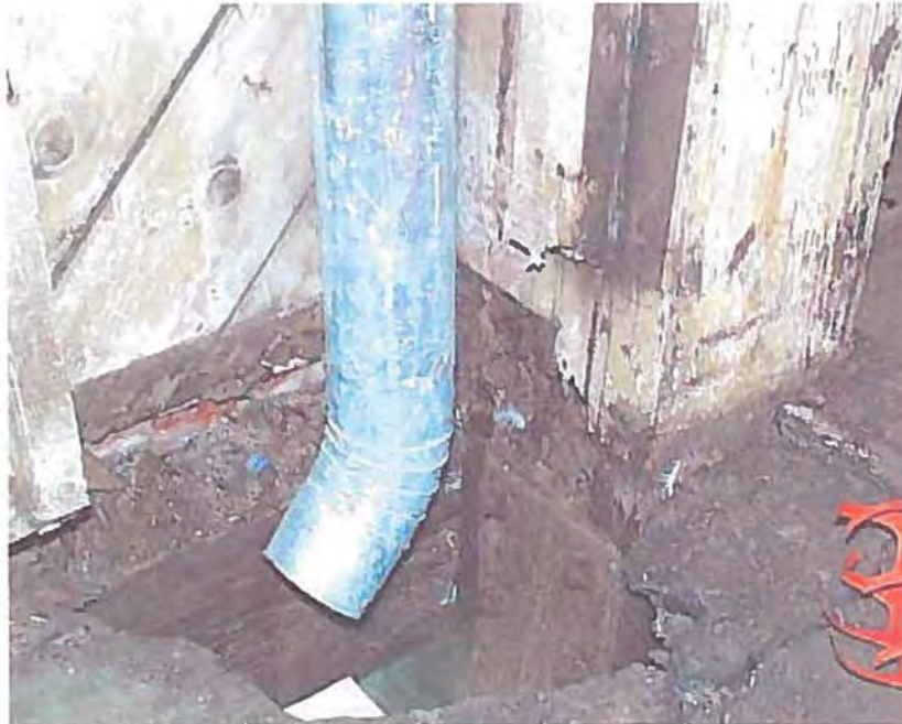
Photo 2: Damaged column base
