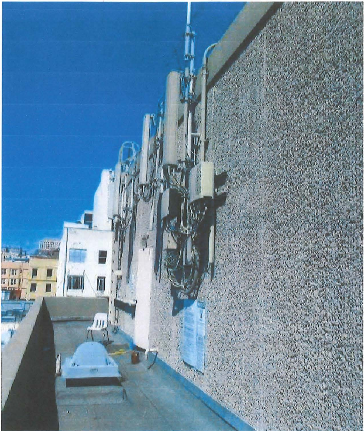
Exhibit A (cont.): Sector B – Antenna Area and Wall Equipment Area
