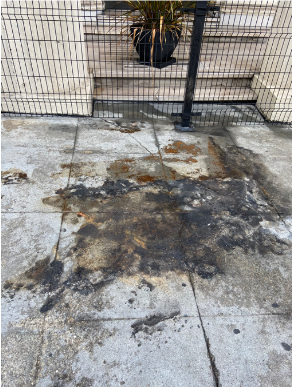
site of fire source AFTER cleaning
