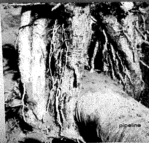
Example of the impact tree roots can have on a pipeline.
