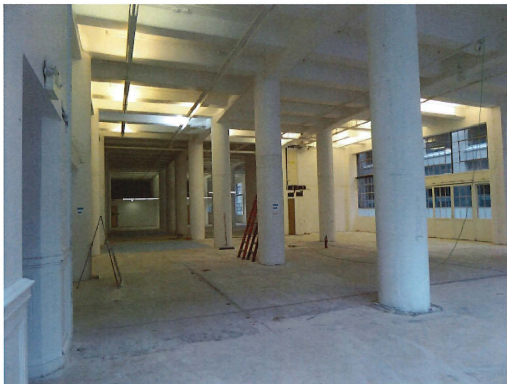
A15. Interior view of first floor, looking west towards the rear of the building (ARG, February 2017).
