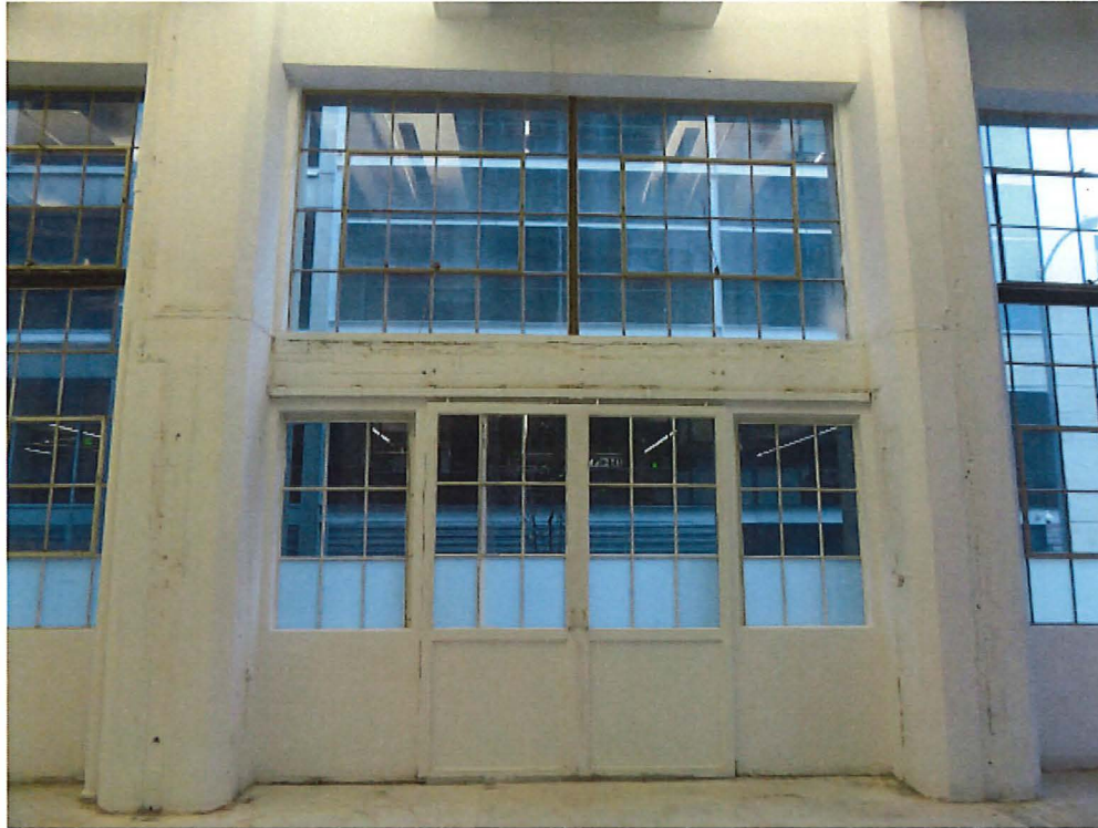
A16. View of sliding doors in the north wall of the building (ARG, February 2017). There is a matching set of sliding doors three bays to the west.
