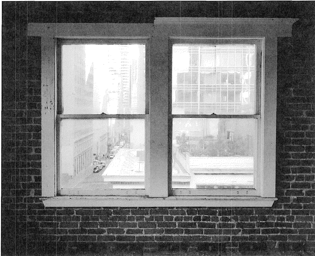
Figure 38: Detail photograph of typical double-hung windows at north and east walls (photograph taken on 02/27/2018).
