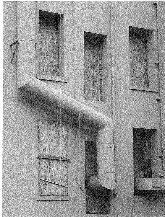
Figure 22: Detail photograph of ventilation ducts projecting through second floor openings. Note size difference between window and door openings (photograph taken on 01/26/2018).
