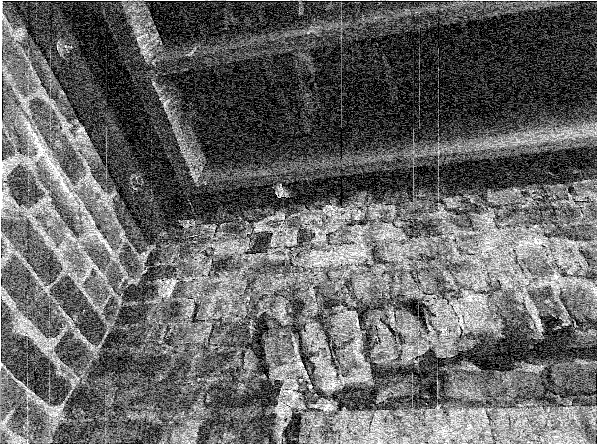
Figure 35: Detail photograph of deteriorated brick mortar joints and efflorescence above southernmost window opening at fifth level. Note rust stains surrounding metal embedments and water stains at underside of roof sheathing (photograph taken on 02/27/2018).
