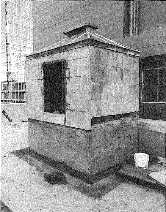
Figure 48: Photograph of elevator penthouse clad in metal panels over wood sheathing. Note surface corrosion on metal panels and missing access door (photograph taken on 02/27/2018)
