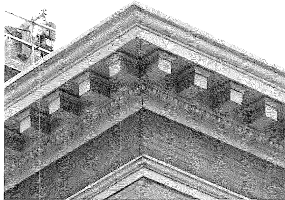
Figure 19: Detail photography of denticulated sheet metal cornice and brick frieze. Note localized paint peeling at cornice (photograph taken on 01/26/2018).
