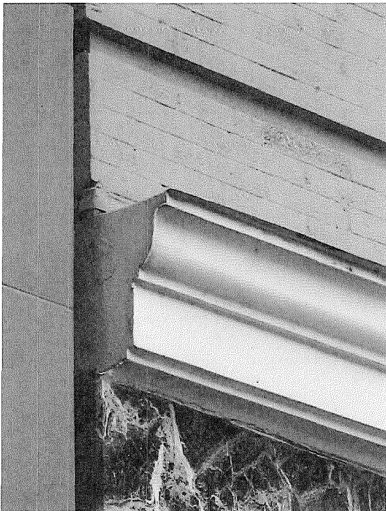
Figure 16: Detail photography of sheet metal water table banding at second floor. Note brick erosion beneath the paint on the brick substrate (photograph taken on 01/26/2018).
