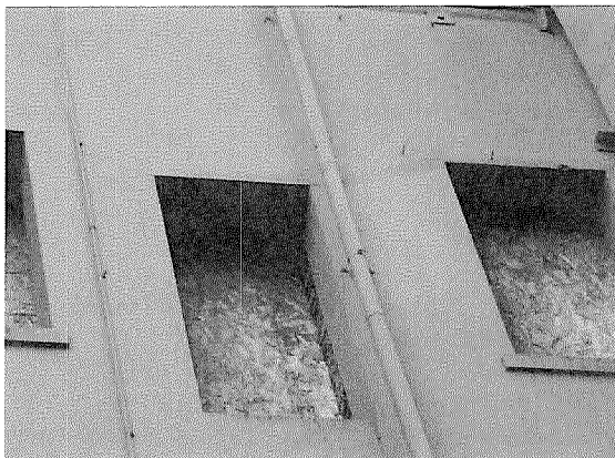
Figure 23: Detail view of punched openings. Note cracked cement plaster between window lintels (photograph taken on 01/26/2018).
