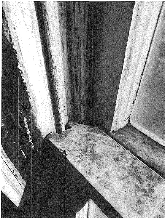
Figure 43: Detail photograph of top edge of lower sash, and sash cord. Note typical paint chipping and missing sash stop (photograph taken on 02/27/2018).
