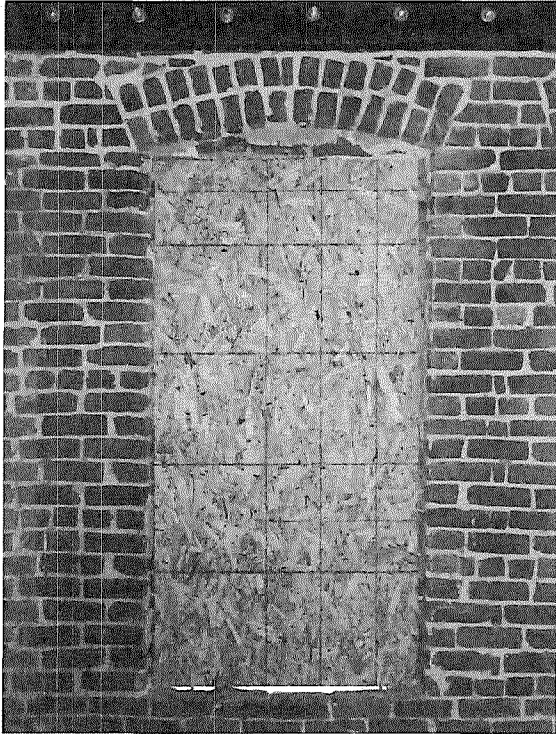
Figure 33: Detail view of typical punched window opening at western wall. Note arched brick lintel (photograph taken on 02/27/2018).
