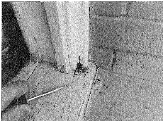
Figure 39: Detail photograph of typical deterioration at window trim (Photograph was taken on 02/27/2018).
