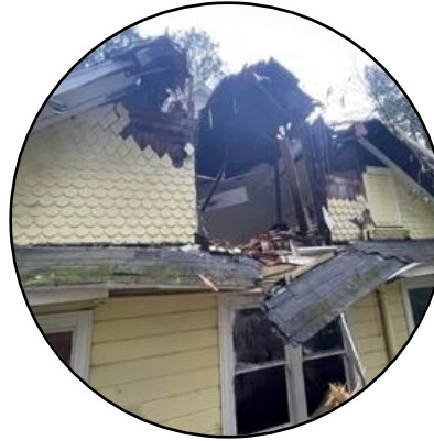
Winter Storm Damage
