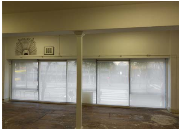
Figure 11. Interior view northwest on mezzanine floor toward windows facing Market Street. [No. 16.25.16] January 2014.
