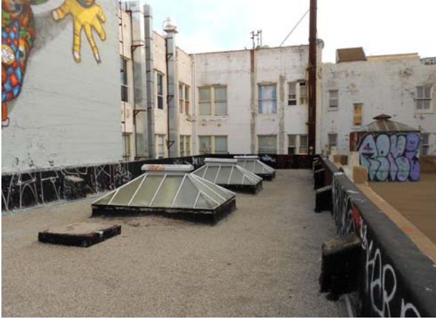
Figure 21. View southeast of rooftop showing hatch, now covered, skylights, tops of columns, and parapet wall. [No. 16.33.45] January 2014.
