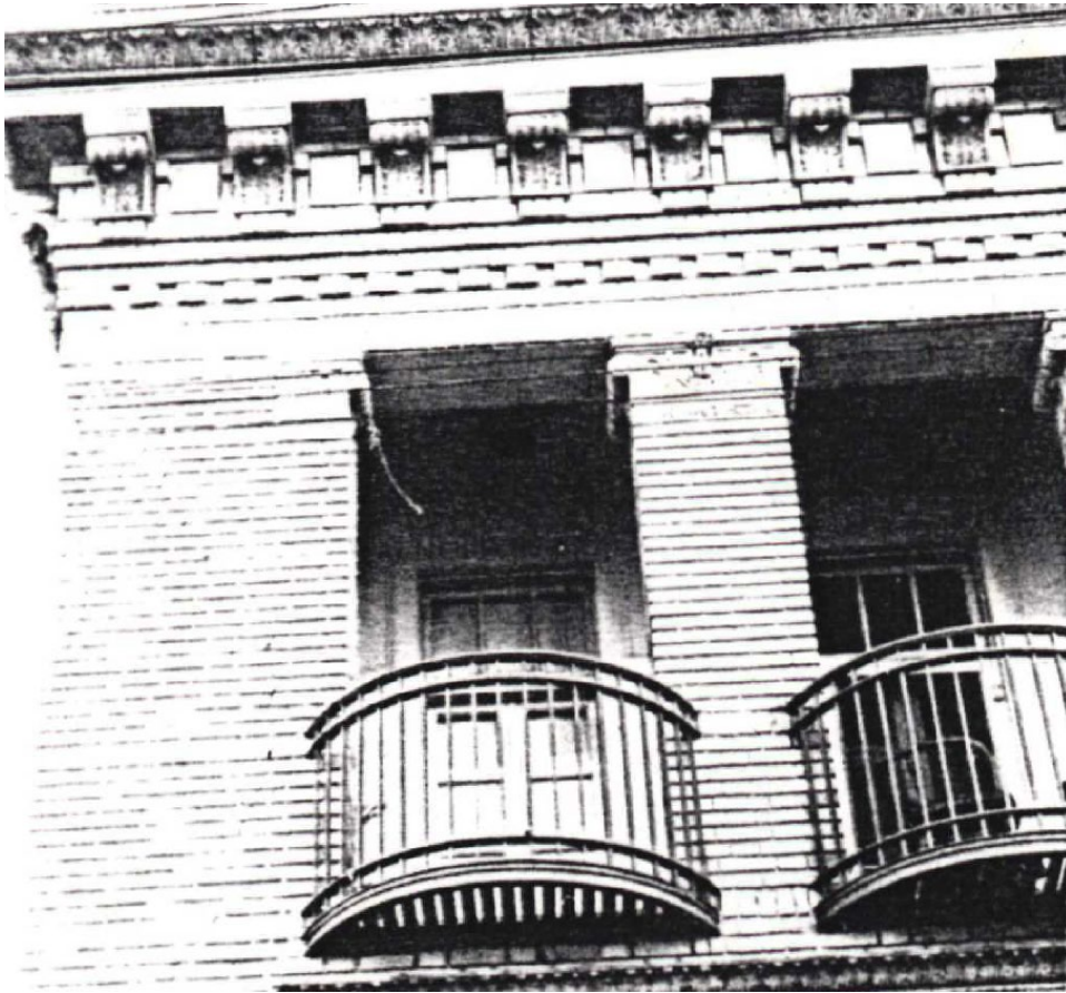
San Francisco Fire Station No. 44, Girard Street façade details, circa 1995. Source: SF Planning Department
