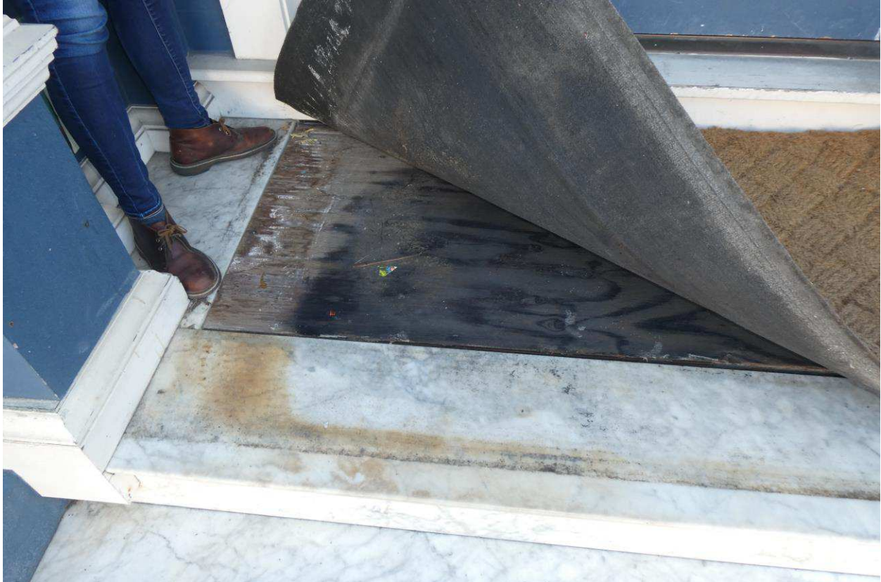
Figure 34: Detail of top entry landing showing plywood infill and ferrous staining of the marble.
