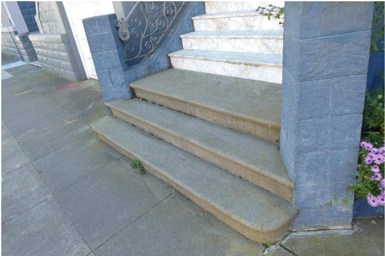
Figure 32: Detail showing plants and biological growth at joints in the concrete and marble stairs as well as beneath some of the bullnose marble stair treads.
