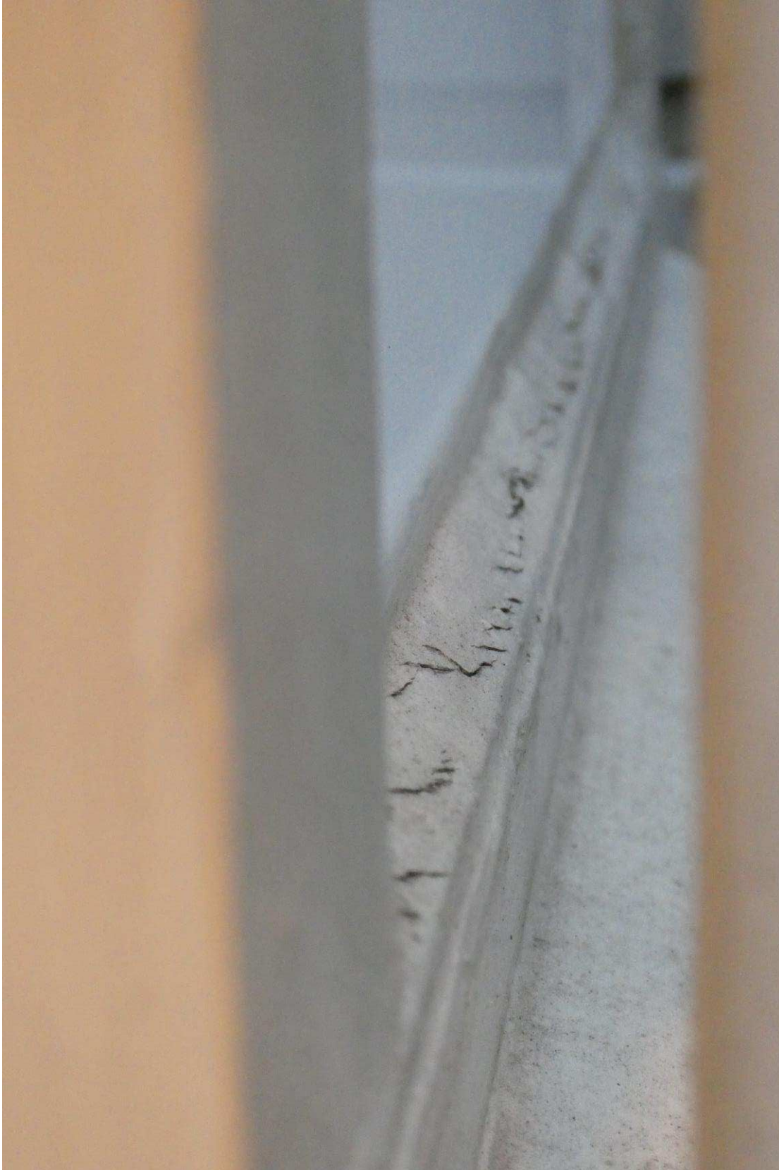
Figure 50: Detail showing deteriorated glazing sealant at the Plexiglas, second floor non-historic casement sash, northeast lightwell.
