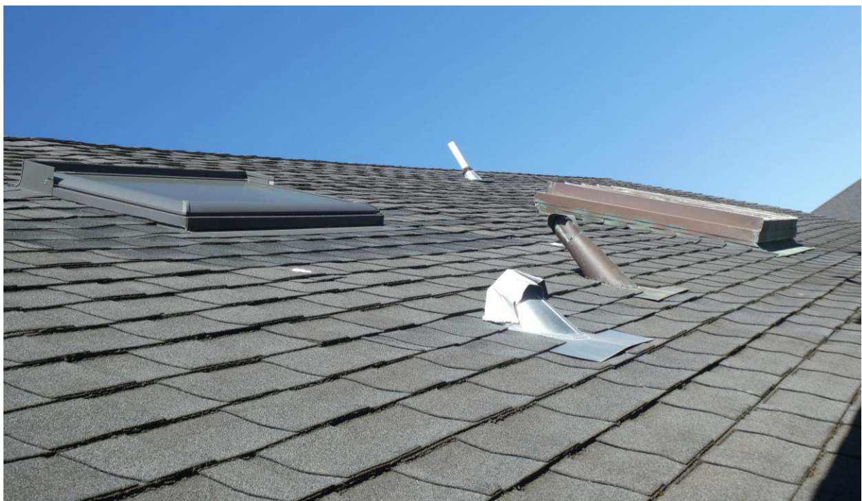
Figure 53: Detail of the asphalt shingle roofing on the main roof and two skylights. The original copper skylight over the interior stair is to the right in the photo.
