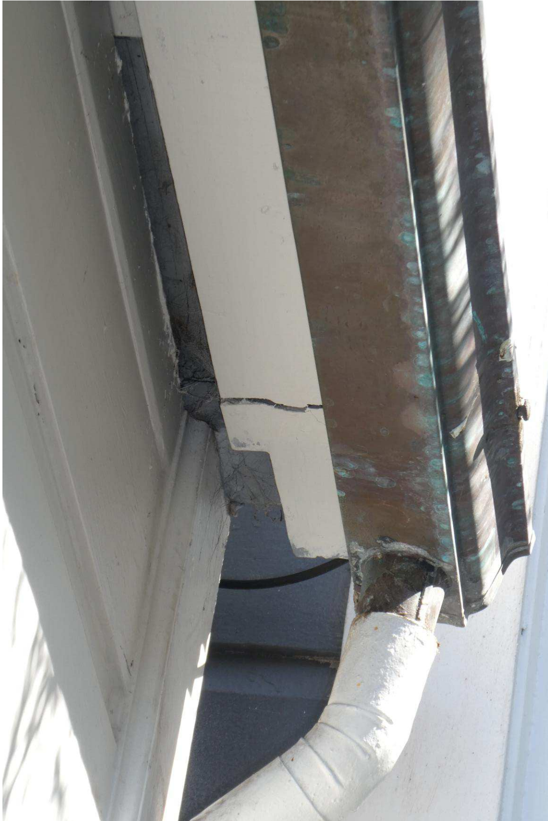
Figure 42: Detail showing the split/damaged wood at the southeast side of the first floor kitchen.
