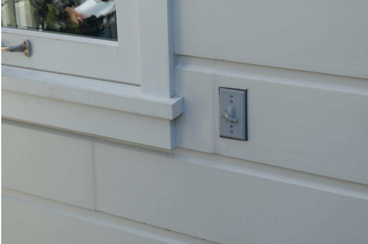
Figure 45: Detail of bulging siding at the lower corner of the window, southwest side of the first floor kitchen.
