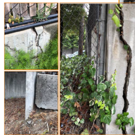
Cooling Tower foundation (above) structurally unstable.
