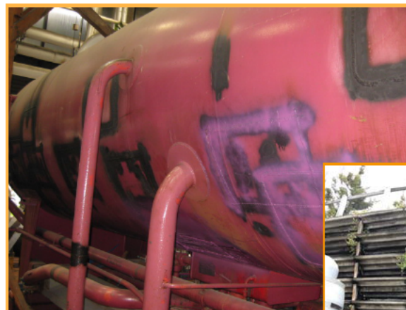
Chiller scarred from multiple repairs (right). Shell interior has delaminated
