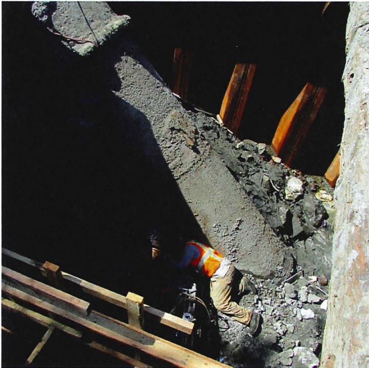
Poor soil conditions and debris encountered during construction, adjacent to aging pipeline
