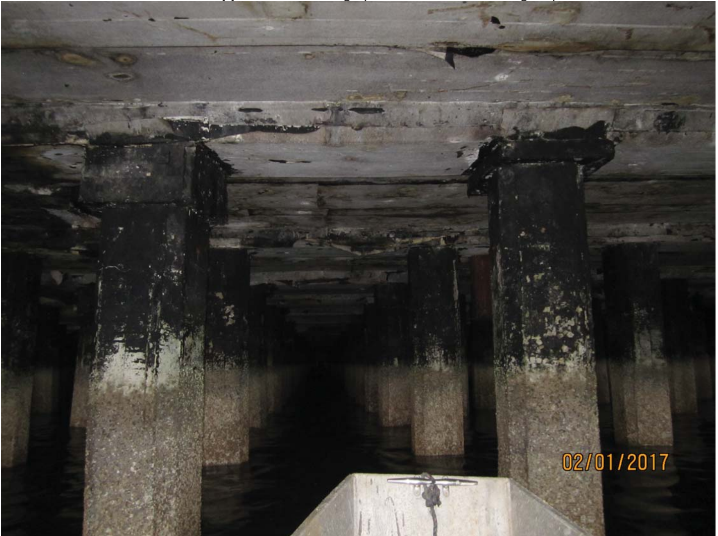
Photo 12. Typical conditions of concrete deck and concrete pile jackets along centerline of pier.
