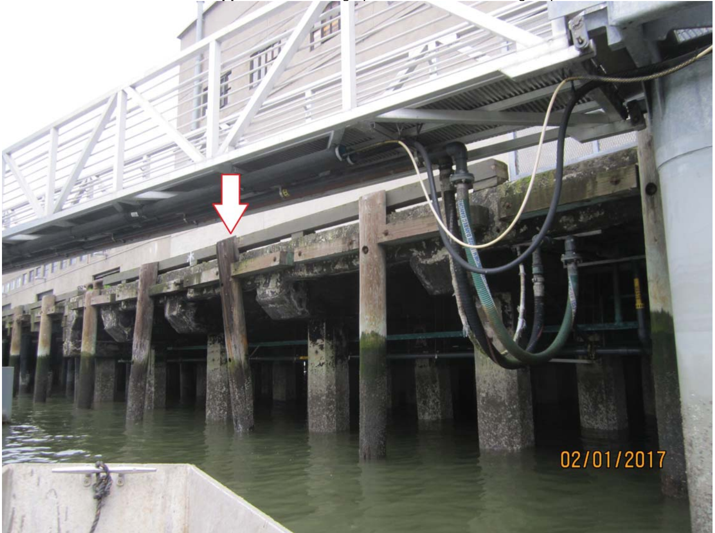
Photo 9. One broken fender pile on northern edge of pier near bulkhead building.
