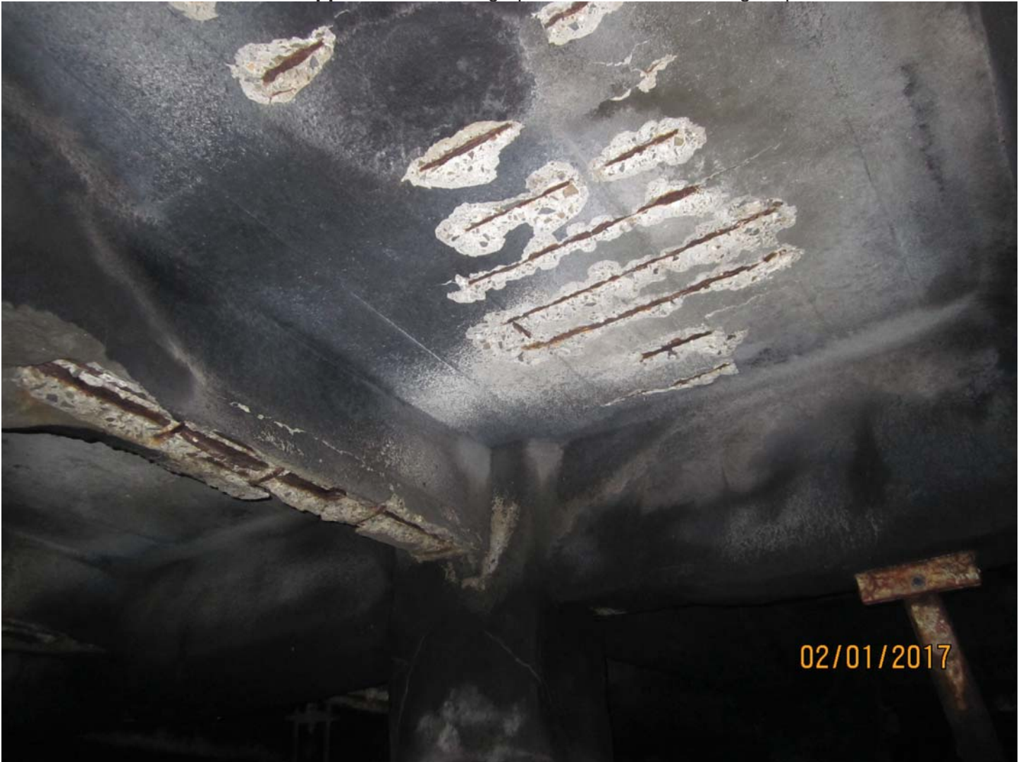
Photo 5. Deck under north end of bulkhead building has more spalls in shotcrete repair due to rebar corrosion
