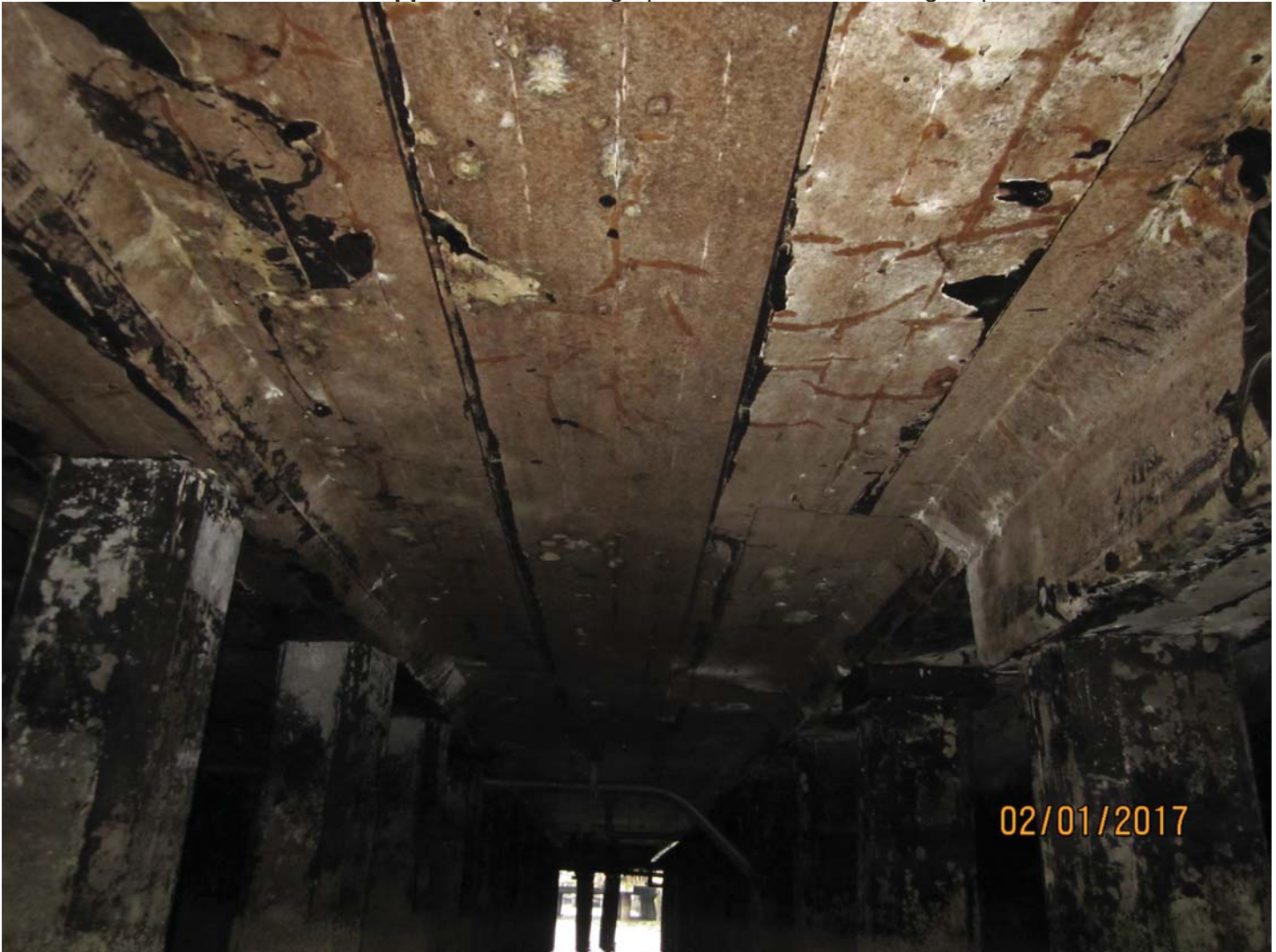
Photo 8. Typical condition of concrete deck. Old waterproofing paper is in varied condition, but appears to have protected the concrete.
