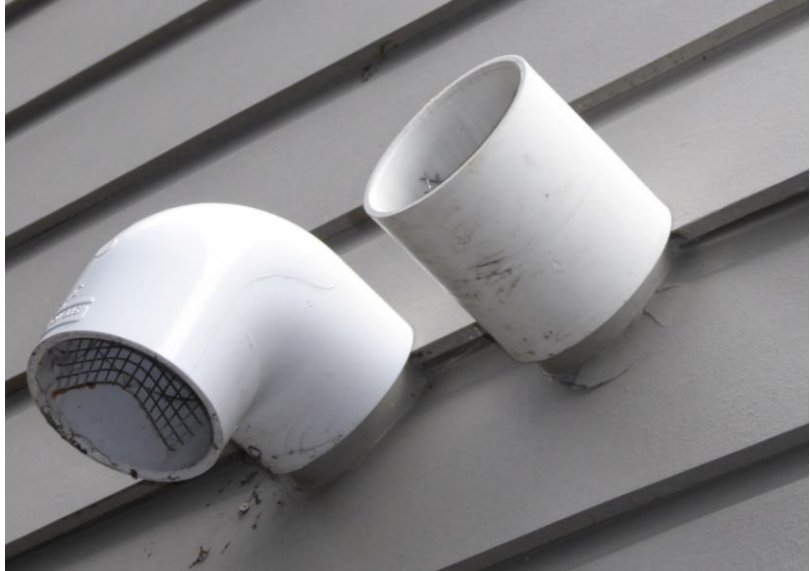
Figure 33: Detail of damaged siding beneath vent.
