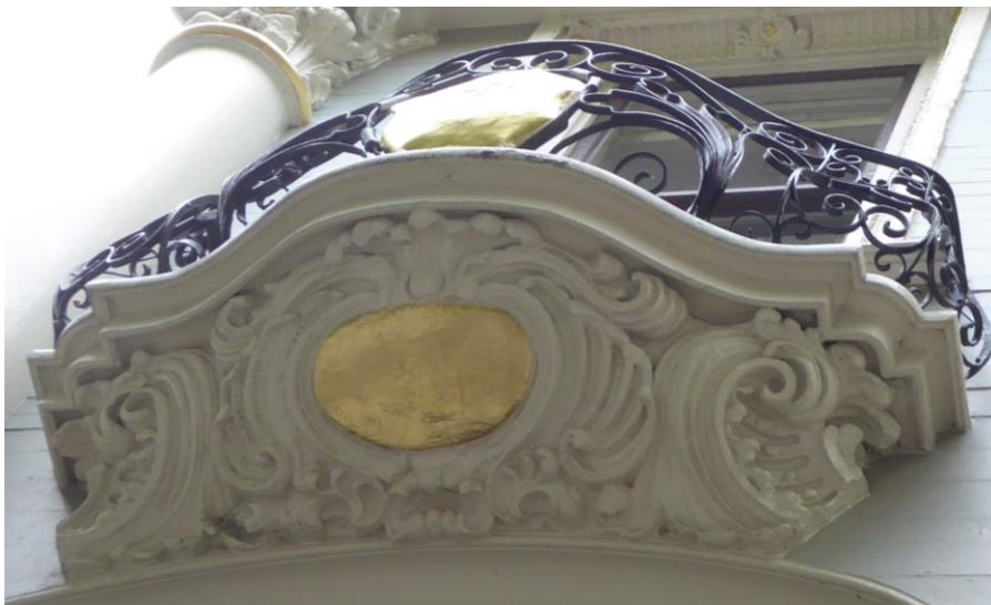
Figure 23: Detail of the molded balcony showing peeling paint at the front edge.
