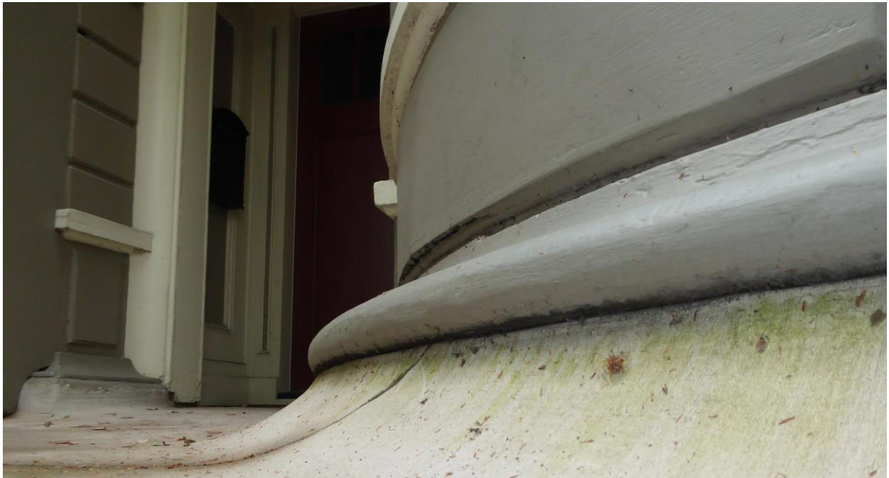
Figure 29: Detail of curb termination at wood trim (beneath area of soft deteriorated wood).
