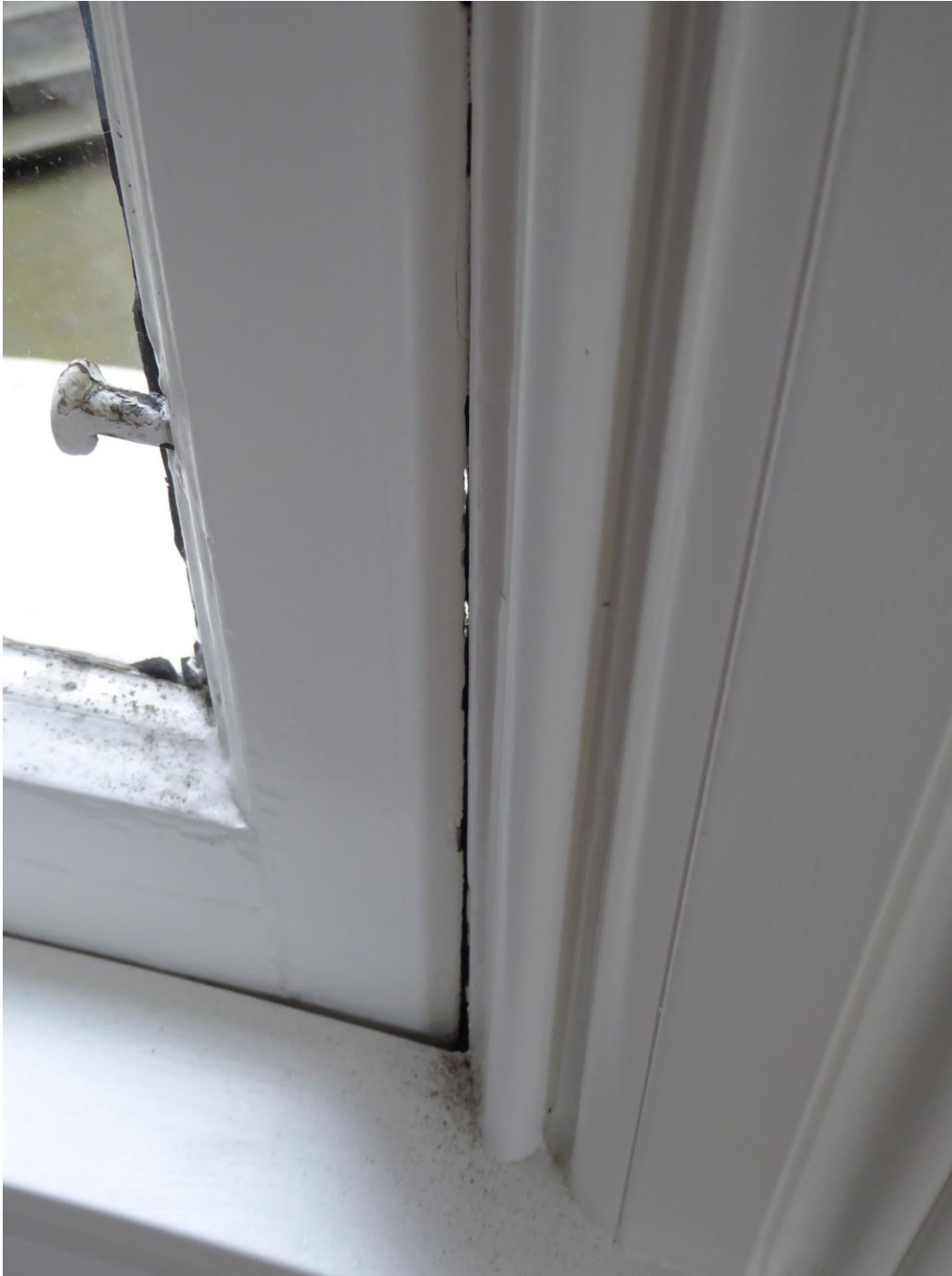
Figure 30: Detail of first floor window from interior showing gap at edge of sash where light is coming through.
