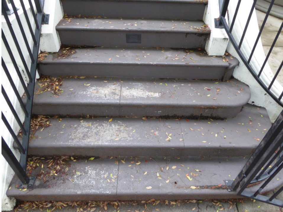
Figure 24: Detail of wear at concrete and wood stairs.
