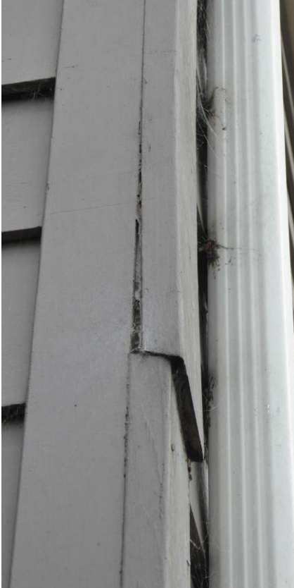
Figure 32: Example of displaced corner trim
