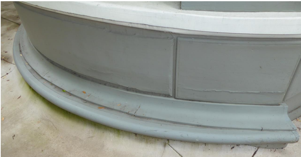
Figure 27: Detail of split wood at rusticated "block" panel and several splits at curved base trim.
