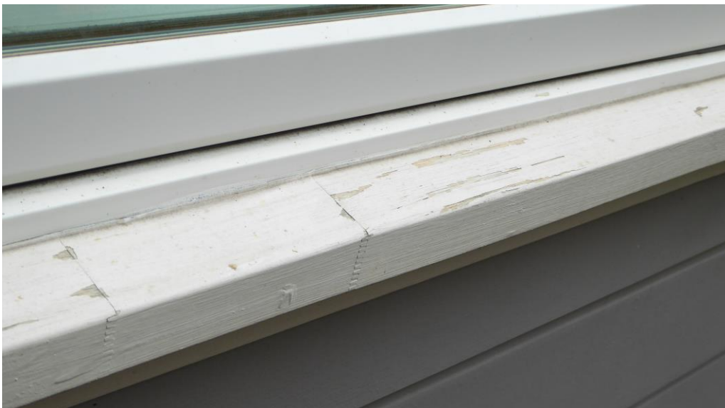
Figure 34: Detail of finger-jointed sill separation and paint degradation.
