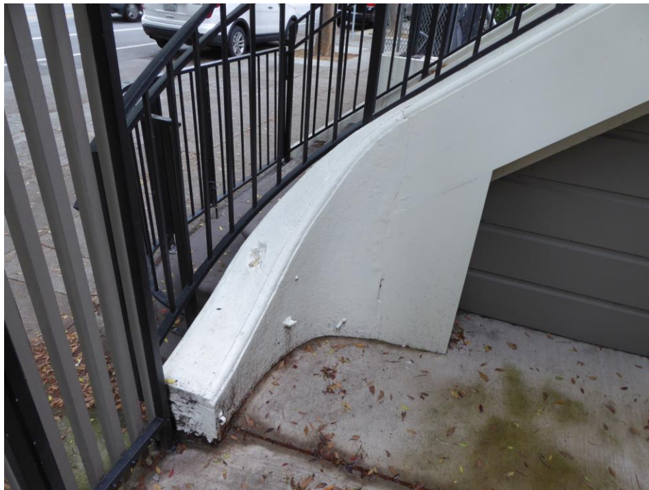
Figure 25: Detail of concrete stair curb with spall.
