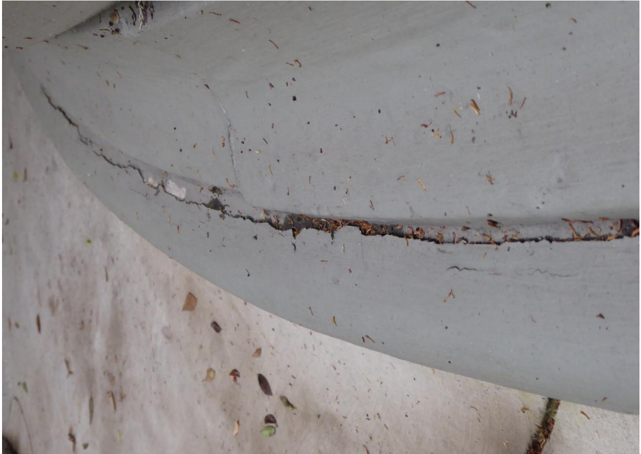
Figure 28: Detail of area where soft deteriorated wood was noted with moisture at the wood.
