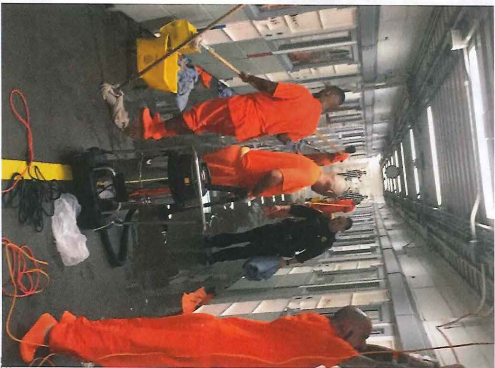
County Jail #4 – Plumbing Overflow January 27, 2017
