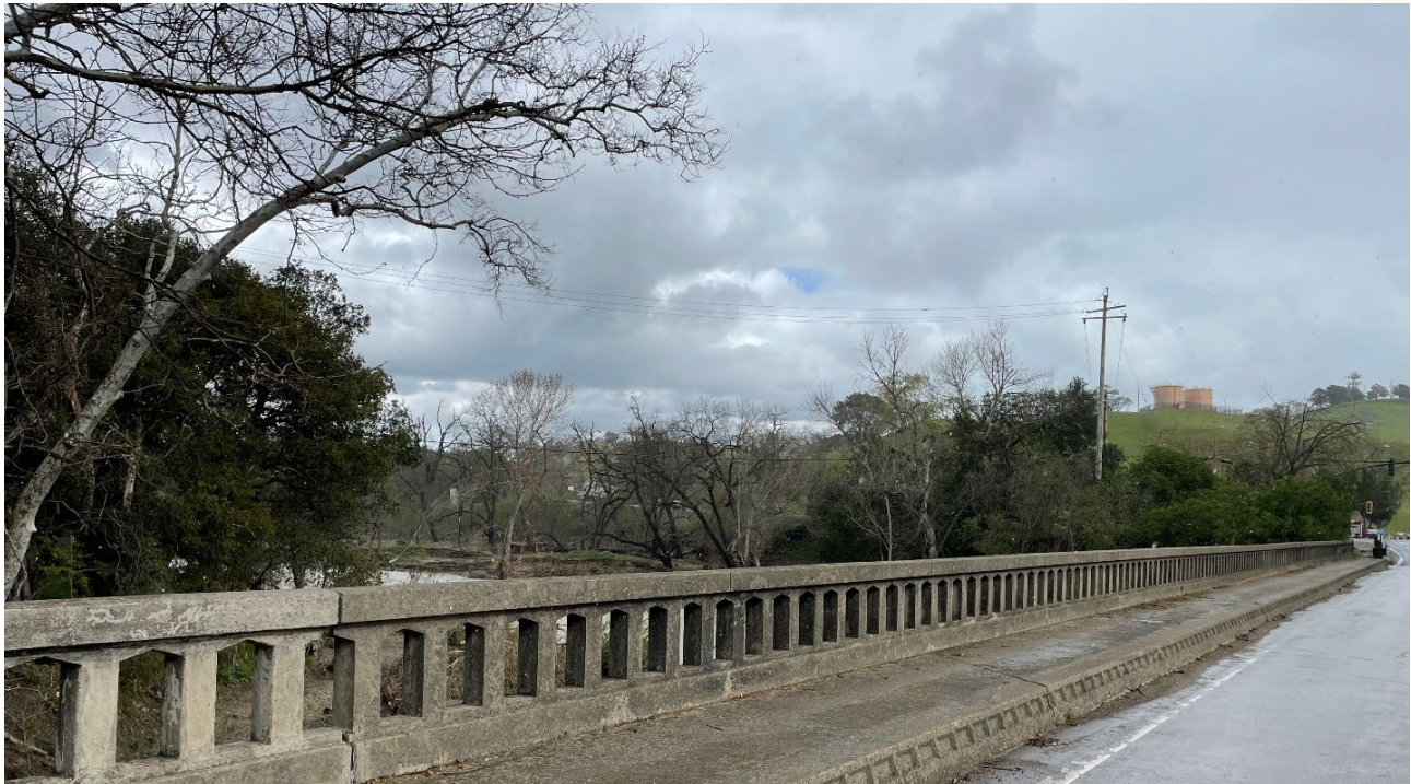
Figure 6: View of the Creek Crossing Work Area Traveling Eastbound on Niles Canyon Road
