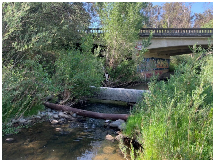
Figure 3: Exposed Concrete-Encased Section of Existing Pipeline Crossing Arroyo de la Laguna with Abandoned 1941 Pipeline in the Foreground
