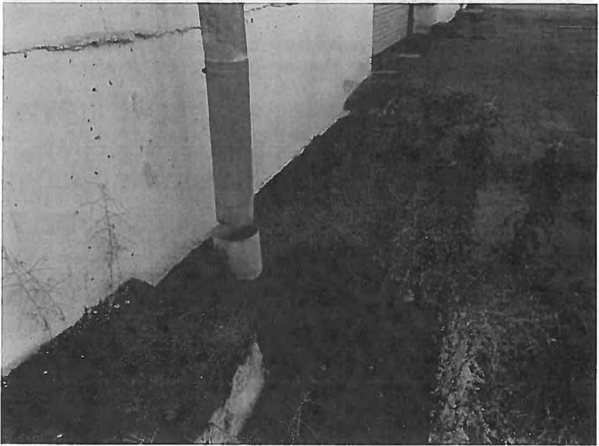
P80 A Shed disconnected rain water liter (Image #30)
