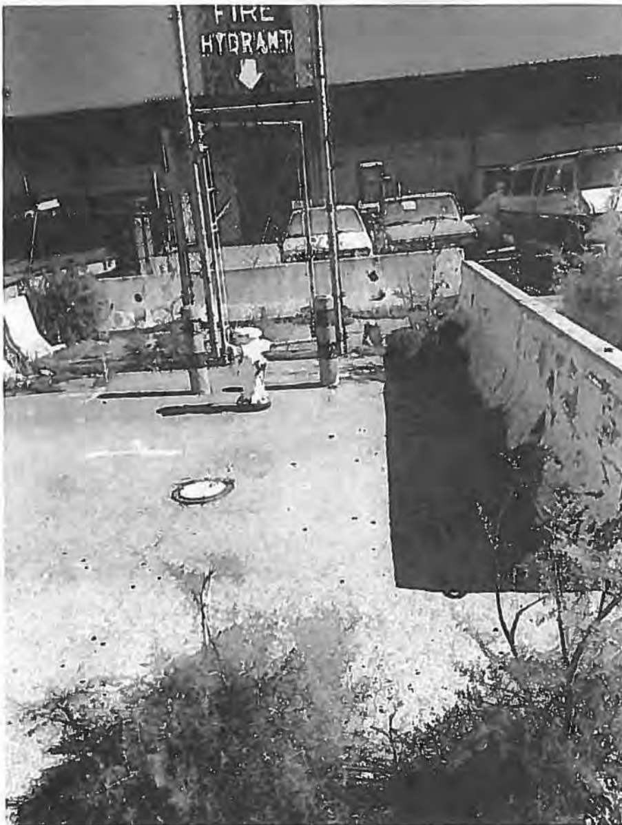
P80 East of Marin Street Gate, private fire hydrant on the master water meter account (Image #23)
