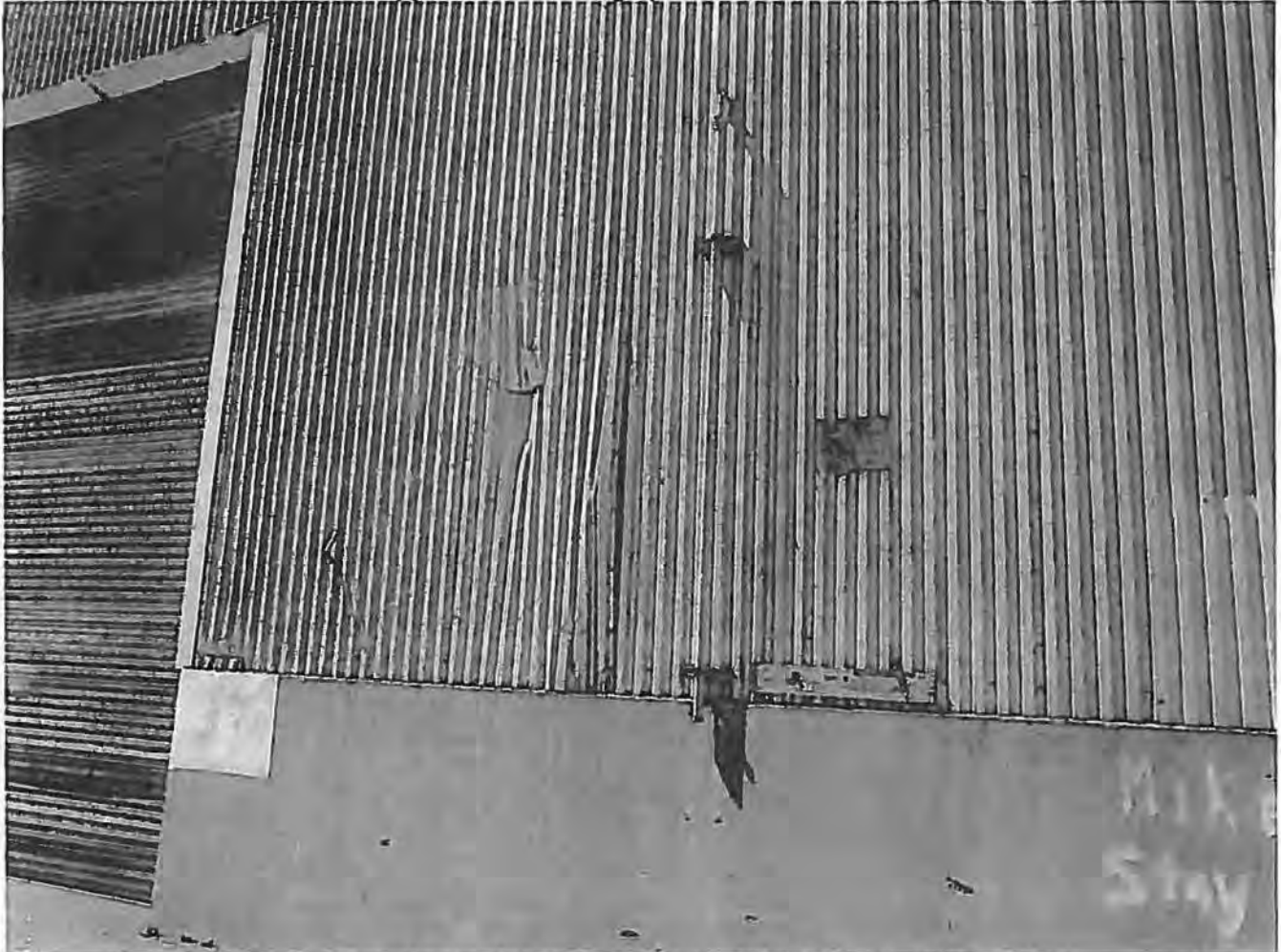
Photo 11. View of the damaged metal siding at the south side of the building
