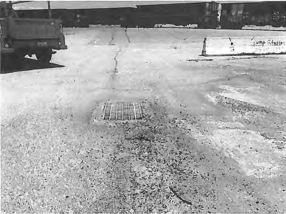
P80 Center East Main Yard; Catch basin with back water valve (Image #17)
