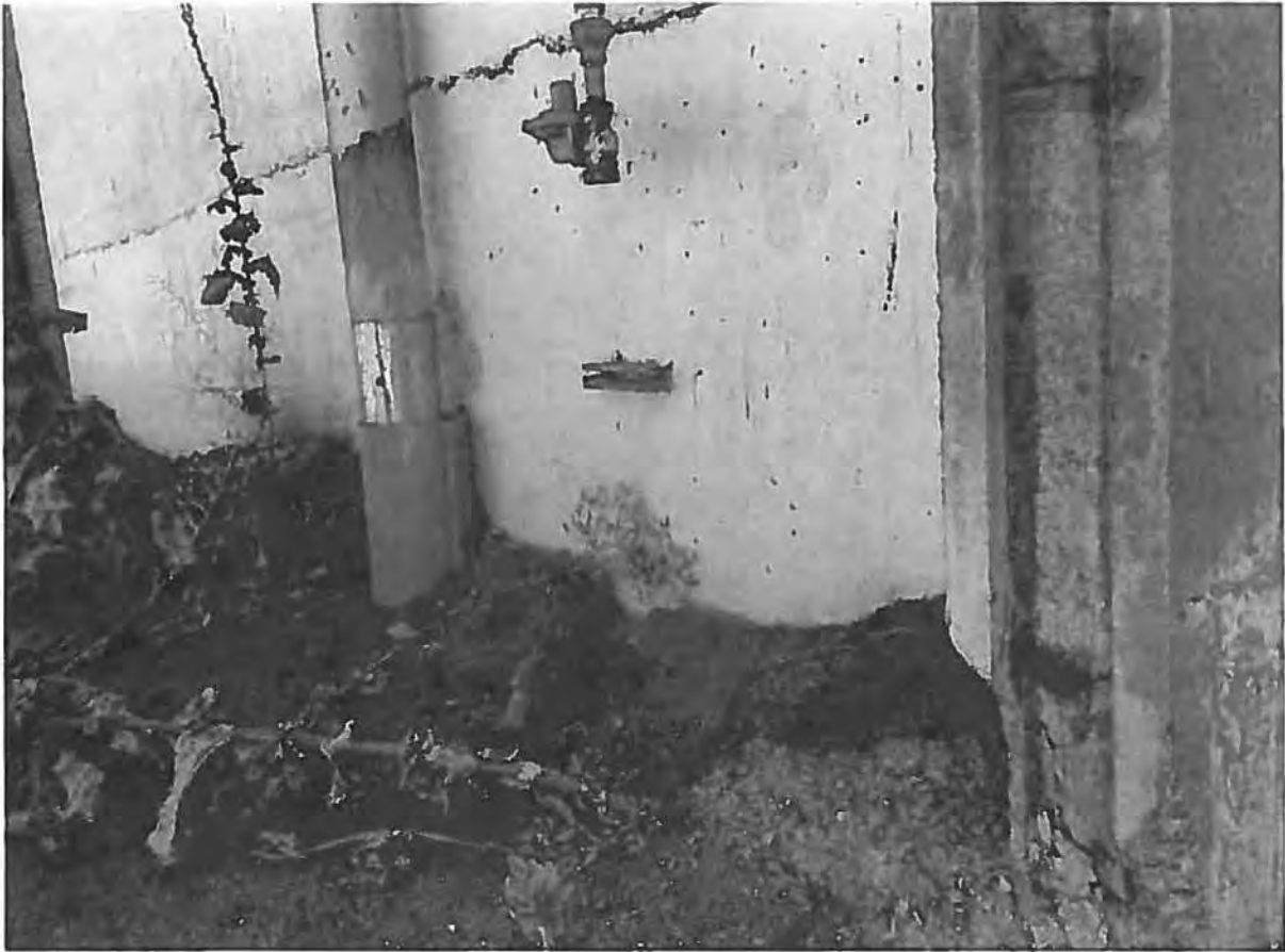
P80 A Shed capped off gas piping, PG&E gas meter exists, just left of image. Replacement line needs flex connector due to ground settlement. (Image #31)
