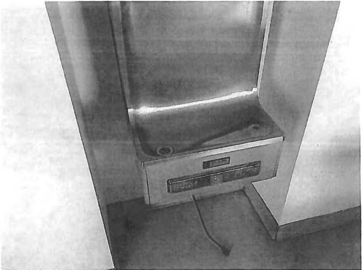
C Stevedore's Building: drinking fountain missing parts (Image #7)
