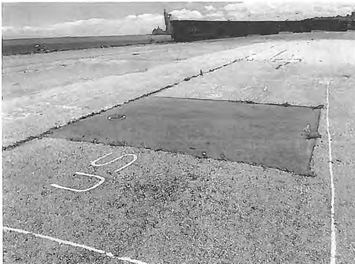
P80 C face underground valve and recent repair for ships water service (Note piping and valve under deck and on face are missing). (Image #19)
