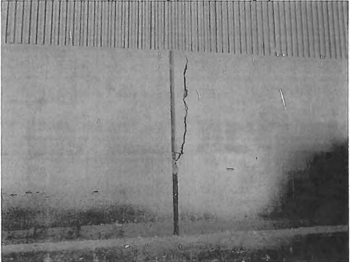
Photo 15. View of the cracking in the concrete walls, looking west
