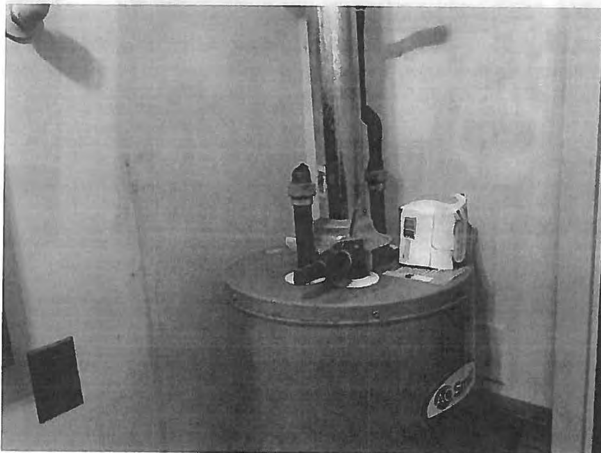
P80 A shed 2 story offices building vandalized water heater (Image #24)
