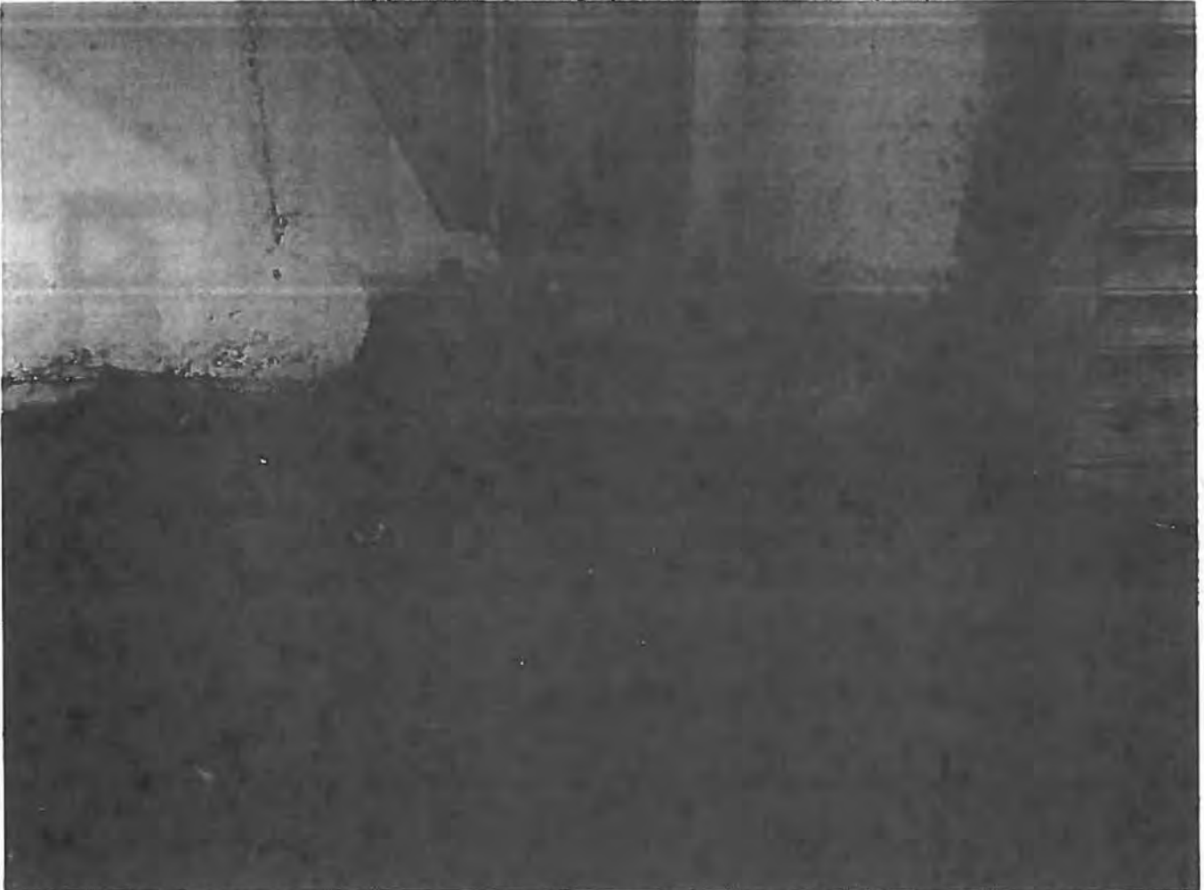
Photo 18. View of the interior steel column with settlement around the column at the south side of the building
