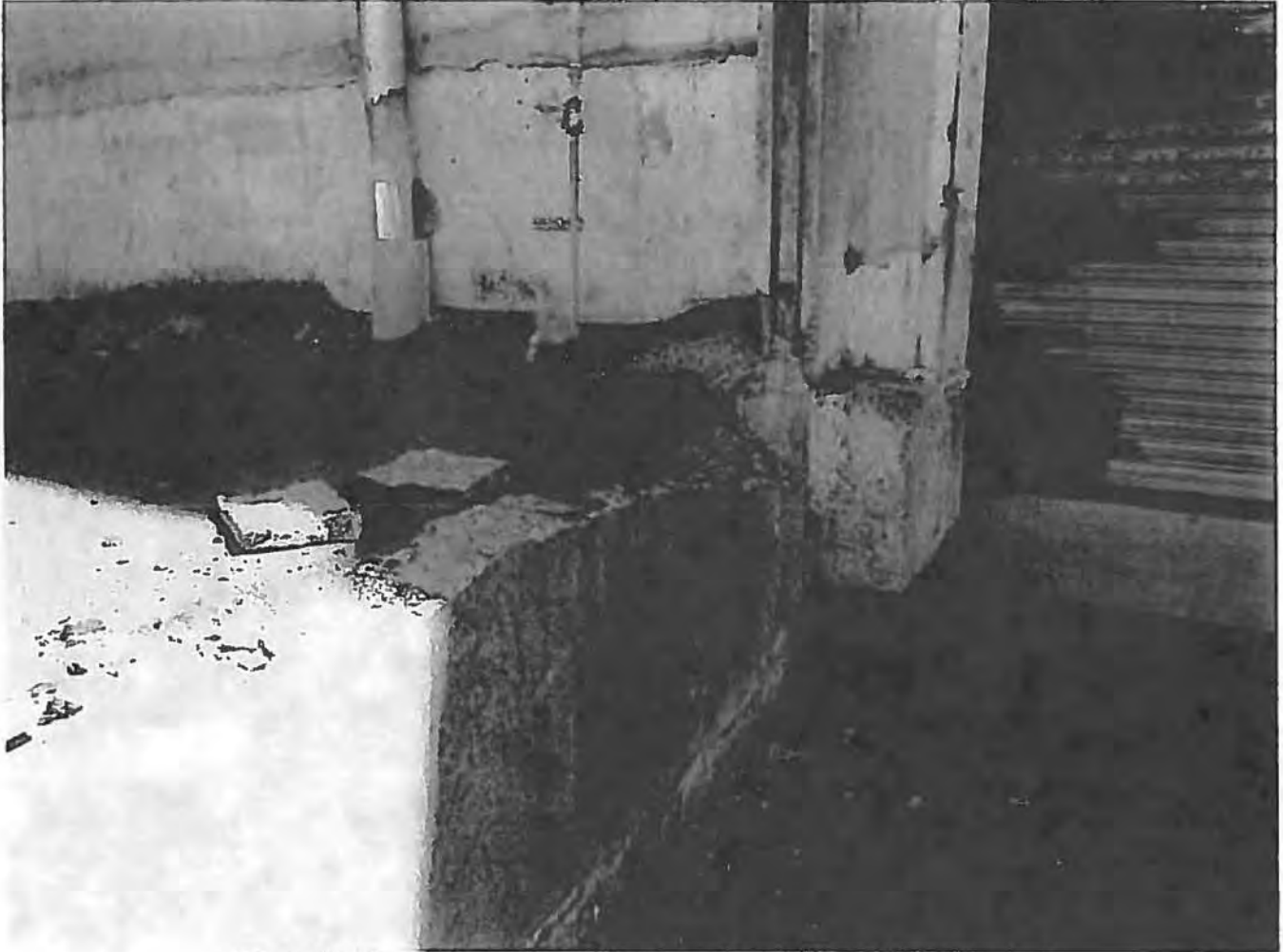
Photo 22. View of the settlement and cracking in the north loading dock
