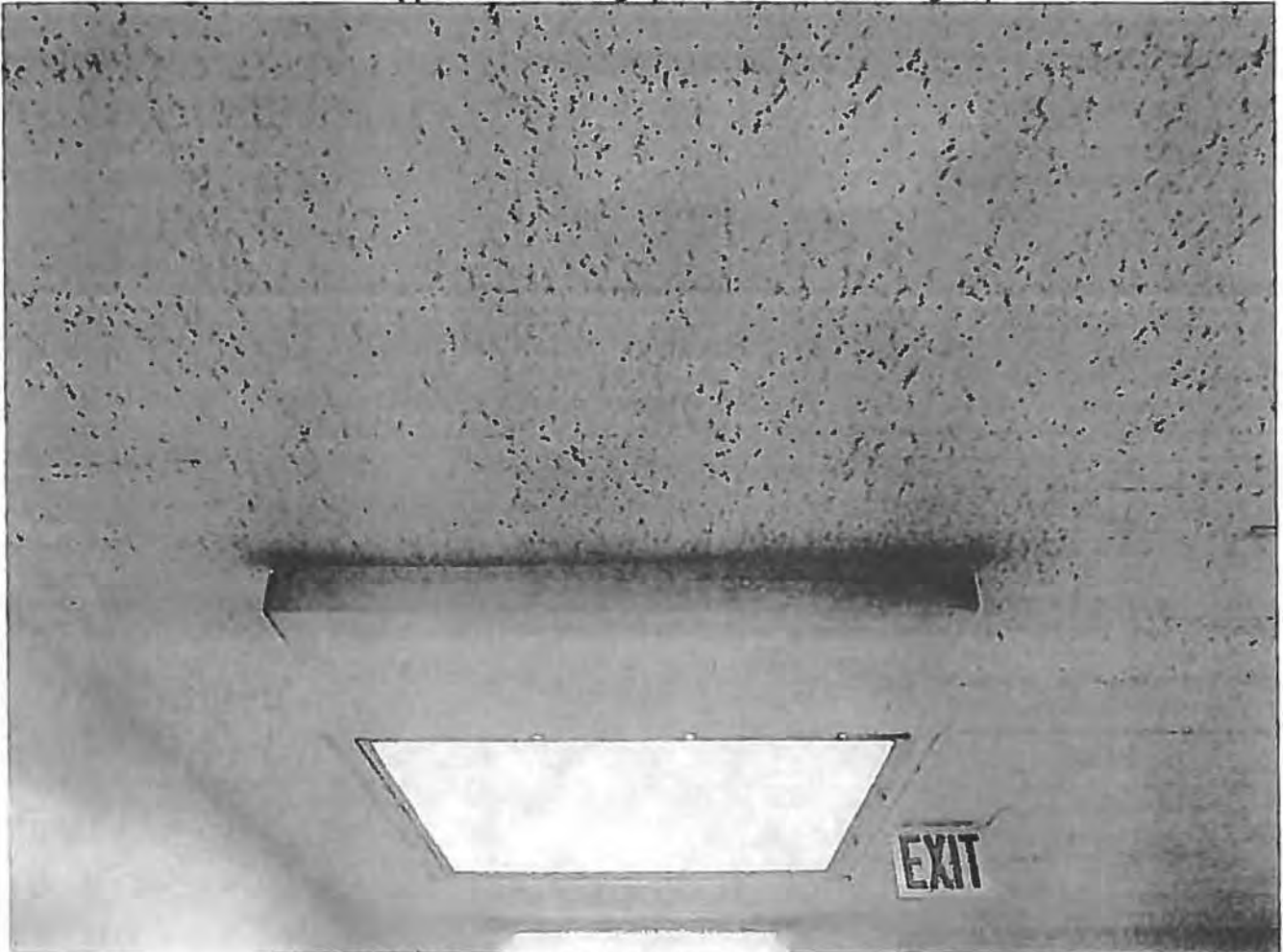
Photo 7. View of the water penetration in the second floor ceiling
