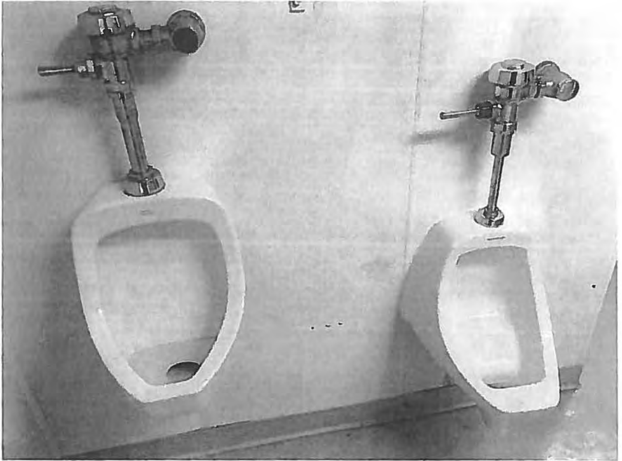
P80 C MRR angle stop cover missing, partition missing (Image #9)
