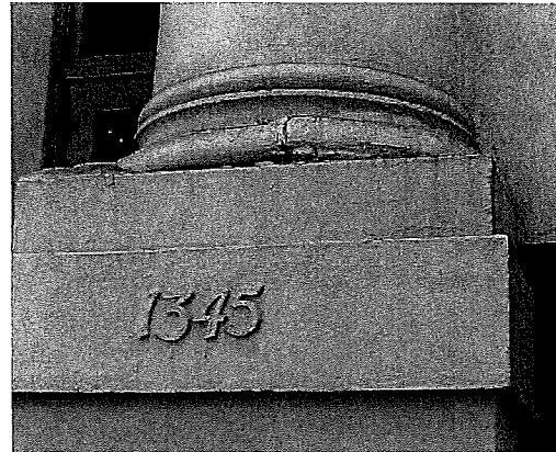
Figure 2: Cracking of concrete column at base.
