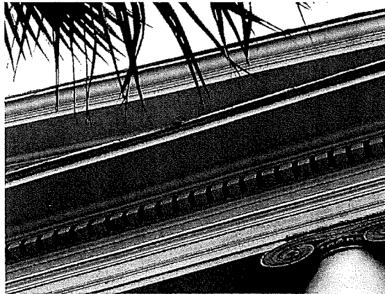
Figure 3: Staining and cracking at roofline suggest roofing issues.
