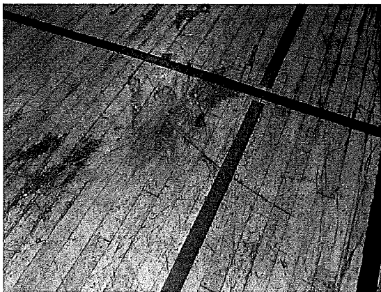
Figure 19: General wear and tear of wood floors from pedestrian traffic.
