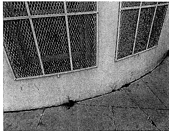
Figure 4: Biogrowth at base indicates possible inadequate drainage.
