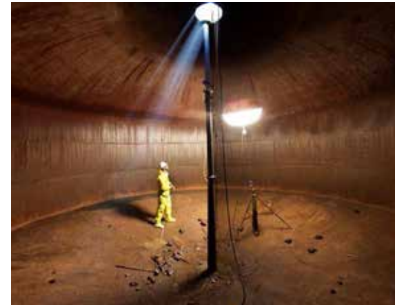
Emergency Firefighting Water System Cistern
