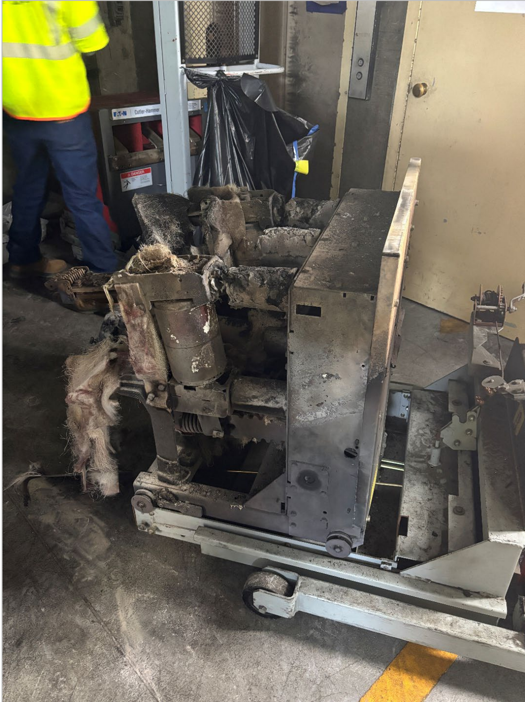
Figure 5. Damaged Circuit Breaker from Cell No. 5 (Incident Breaker No. 52). 23
