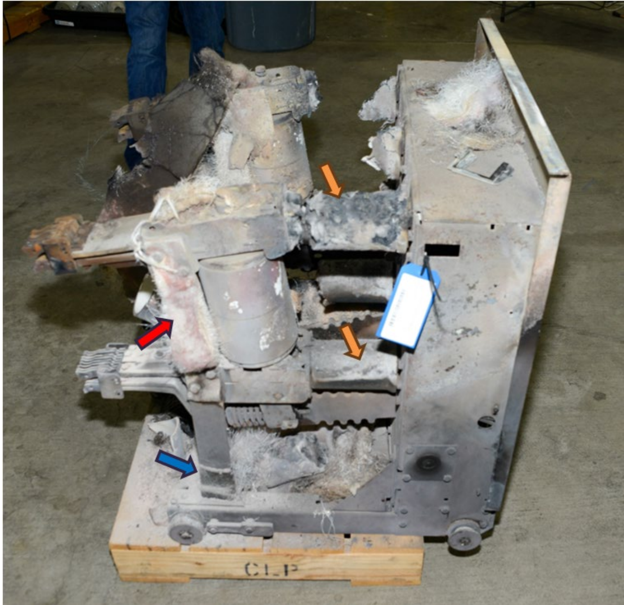
Figure 15. Thermally damaged electrical insulators for electrically isolating the vacuum bottles (orange arrows), damaged vertical insulating bars at each phase (red arrow), and rubber insulators at the bottom (blue arrow).
