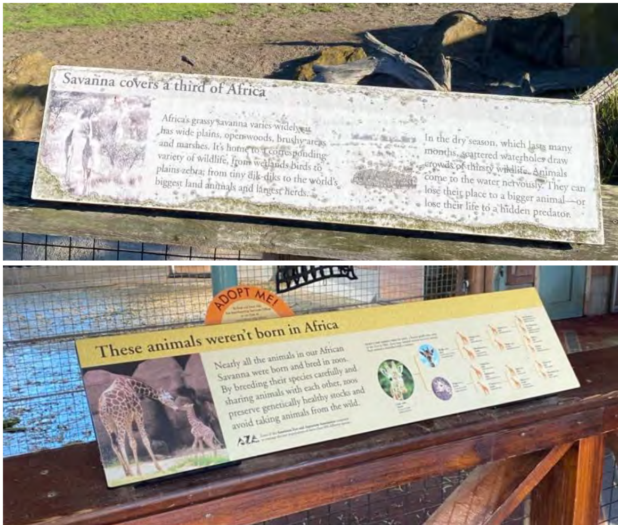
The top photo shows an educational sign within the African Savanna region that has been corroded by salt and sun, largely rendering the text illegible. The signage inventory from 2019, more than five years before this photo was taken, records that this exact sign is faded to the point of needing replacement. The second photo below is a sign located indoors in the giraffe barn for comparison purposes. Source: BLA site visit observations (October 2025).
