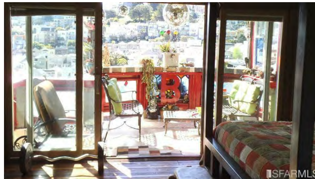
VIEW OF THE TOP FLOR REAR BALCONY NOTE THE APPROX. 36" HIGH RAILING AND THE DISCO BALLS HANGING FROM THE ILLEGEL REAR ROOF ANWING THAT WAS REMOVED
