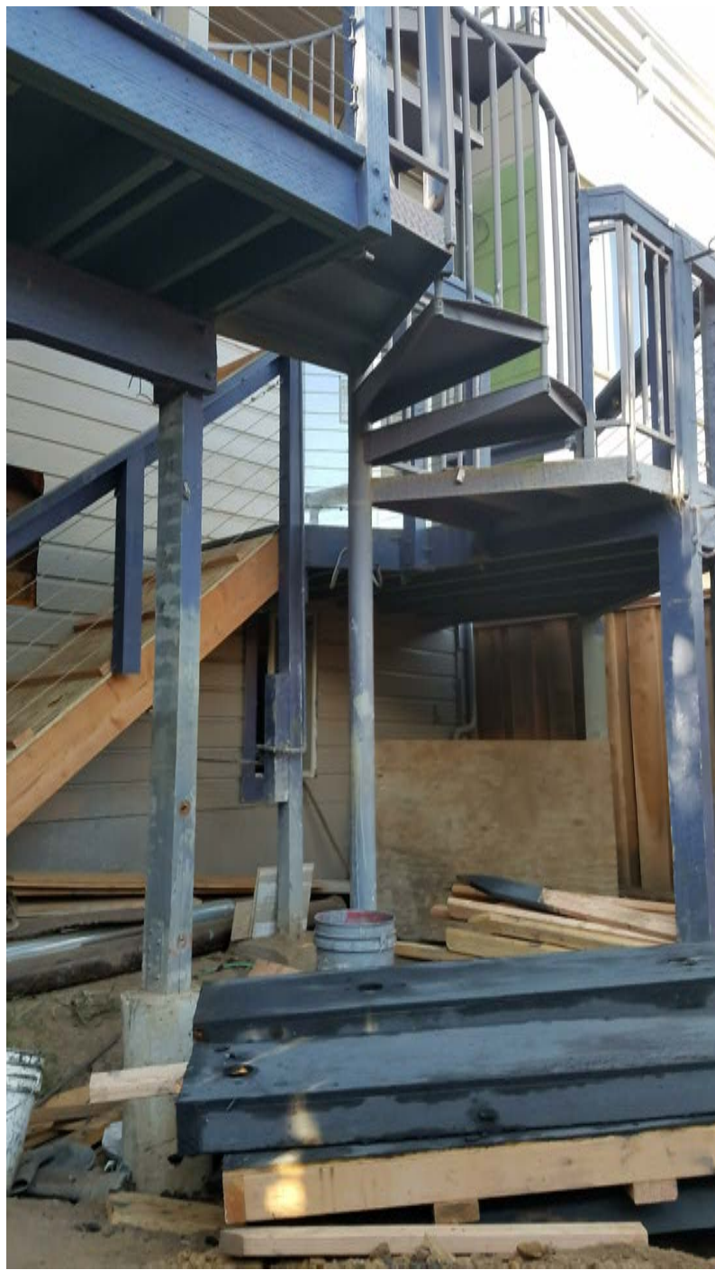
PHOTO OF AWKWARD SPLIT DECK
