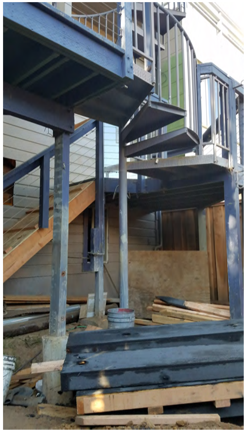
PHOTO OF AWKWARD SPLIT DECK
