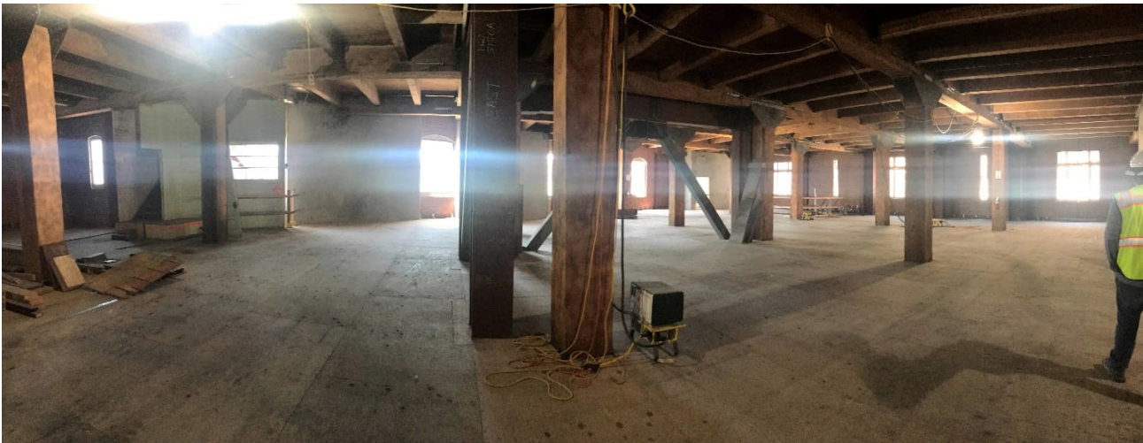
Above: Southeast addition interior, second story. Planning Department Staff, August 2021 Middle: Northeast addition interior, second story. Planning Department Staff, August 2021 Below: Main building interior, second story. Planning Department Staff, August 2021
