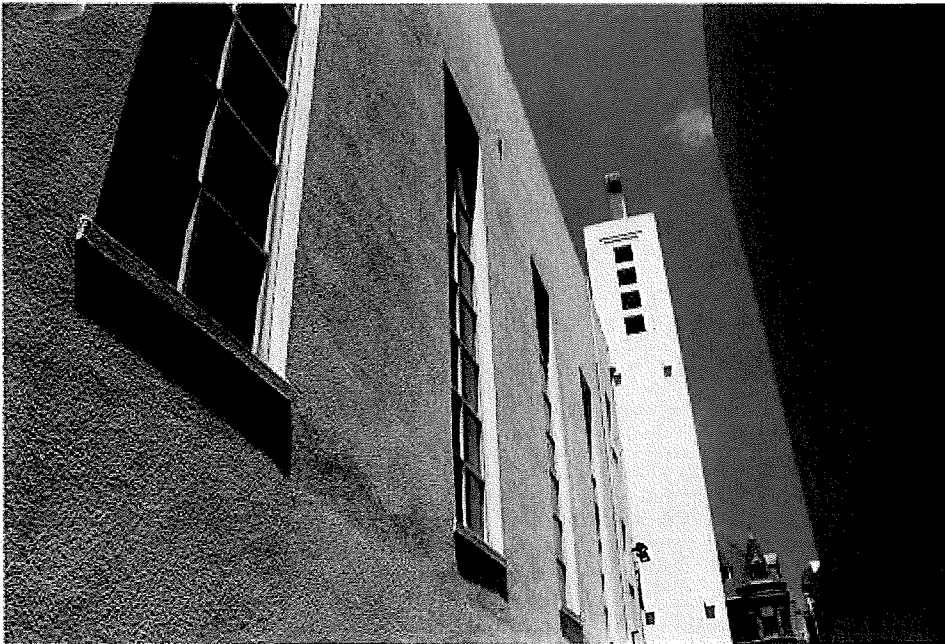
East elevation of church building, vertical wood ribbon windows with divided lites and yellow glass, and south elevation of bell tower. View northwest.
