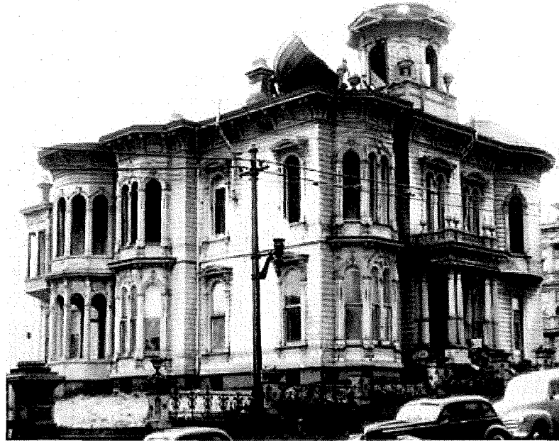
Above: Workers remove the turret on the observatory in the cupola of the former mansion of Captain Charles Goodall at Pierce and McAllister Streets, which was demolished and replaced with Third Baptist Church in 1952 (Courtesy San Francisco Public Library Photo Collection)
