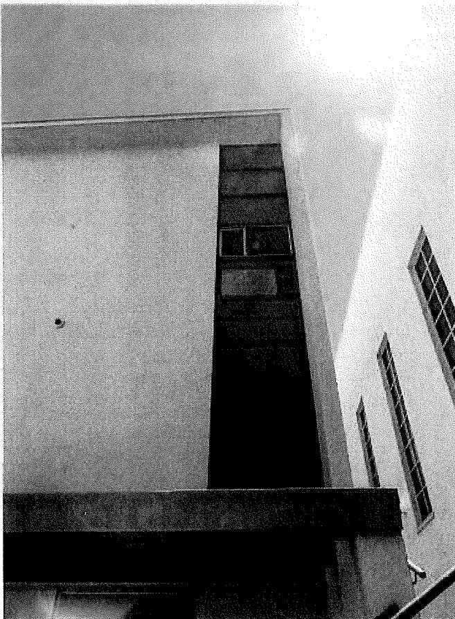
Vertical wood ribbon windows with textured yellow glass on north elevation of youth center and fellowship building, view south.
