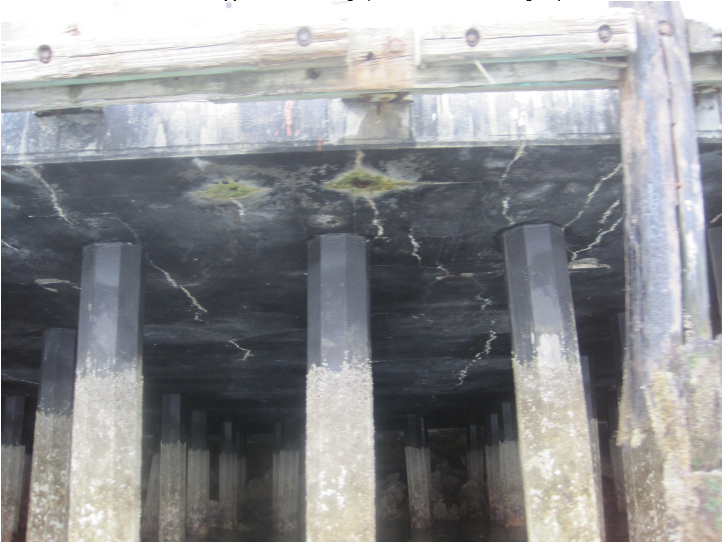
Photo 4. Cracks in concrete deck
