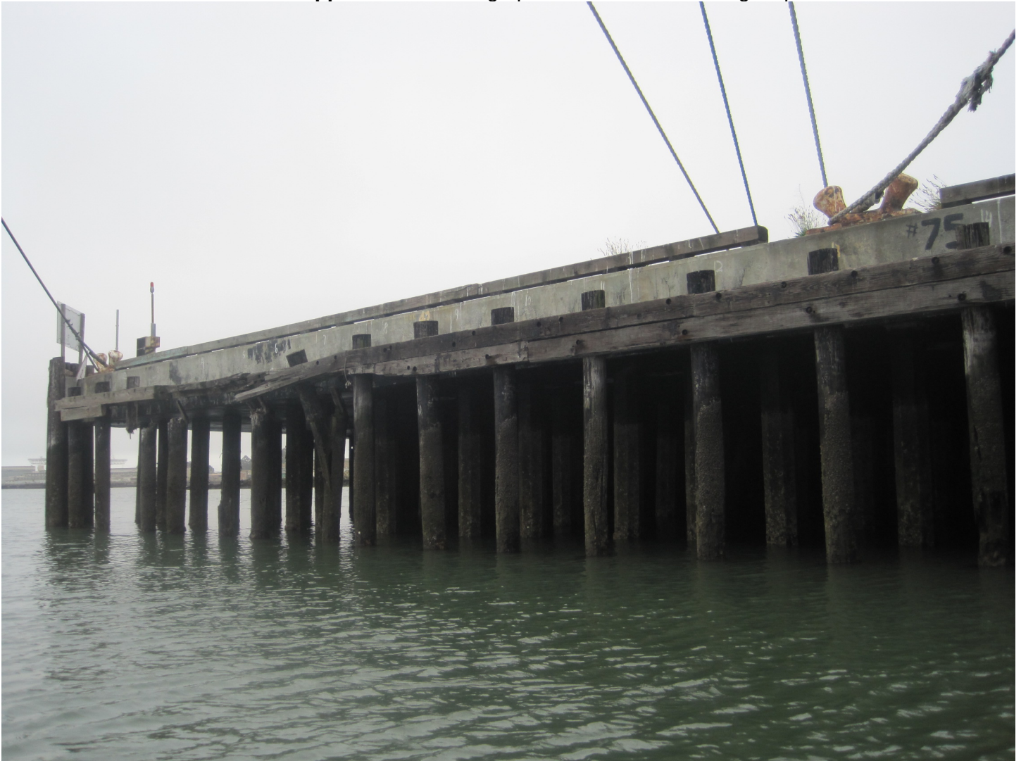
Photo 3. Damaged/deteriorated fendering system
