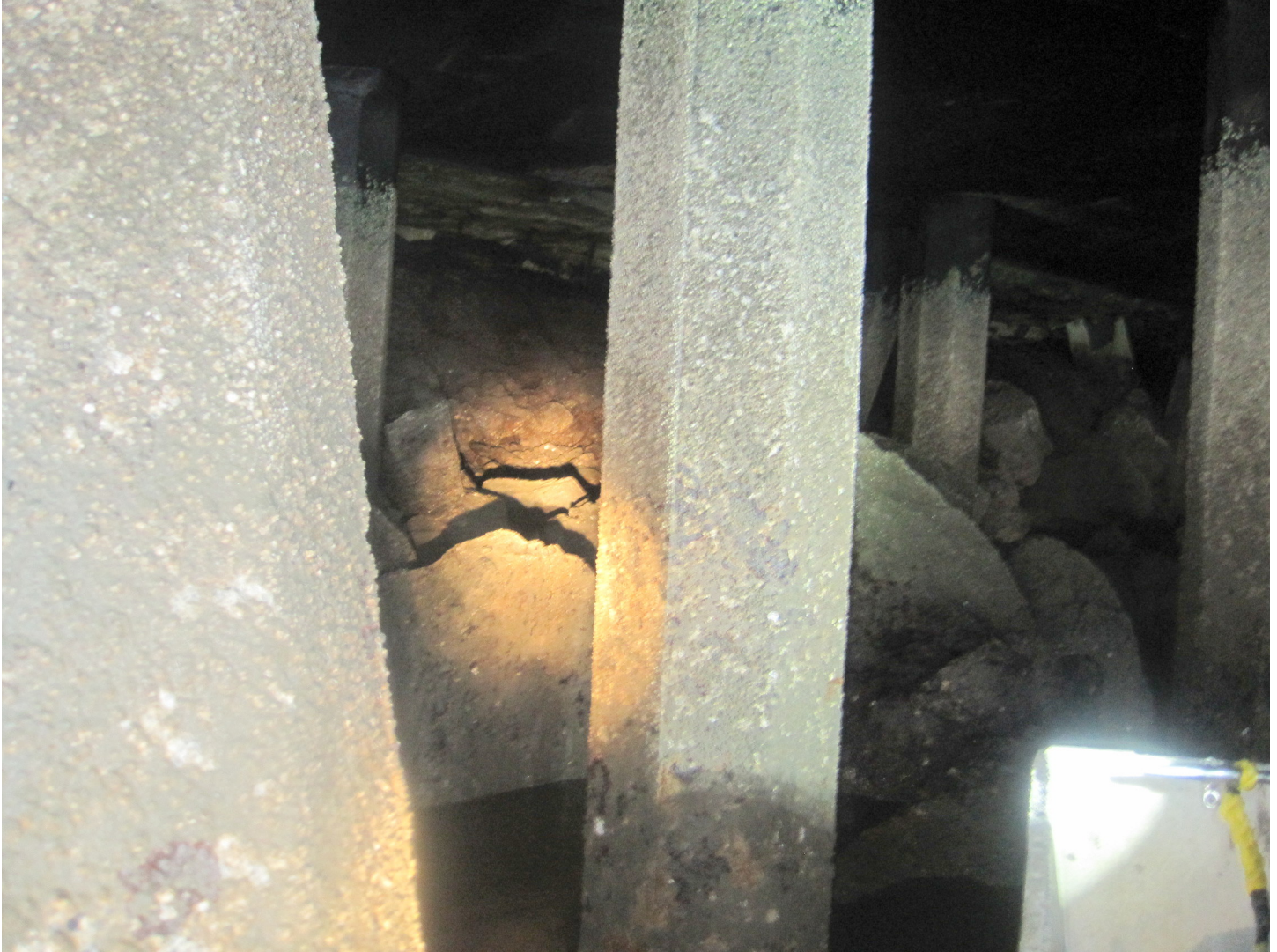
Photo 5. Undermining of seawall
