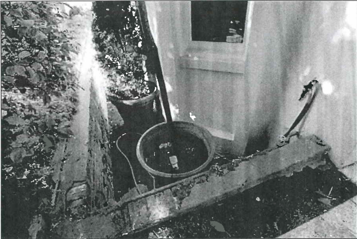
Photo 10. Burr House, 1772 Vallejo Street, 94123. Detail of unreinforced masonry retaining wall adjacent to south facade. Note cracking and mortar deterioration.
