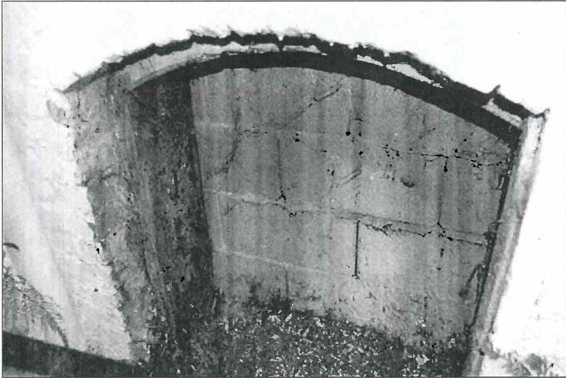
Photo 19. Burr House, 1772 Vallejo Street, 94123. Detail of concrete CMU shear wall at west elevation basement.
