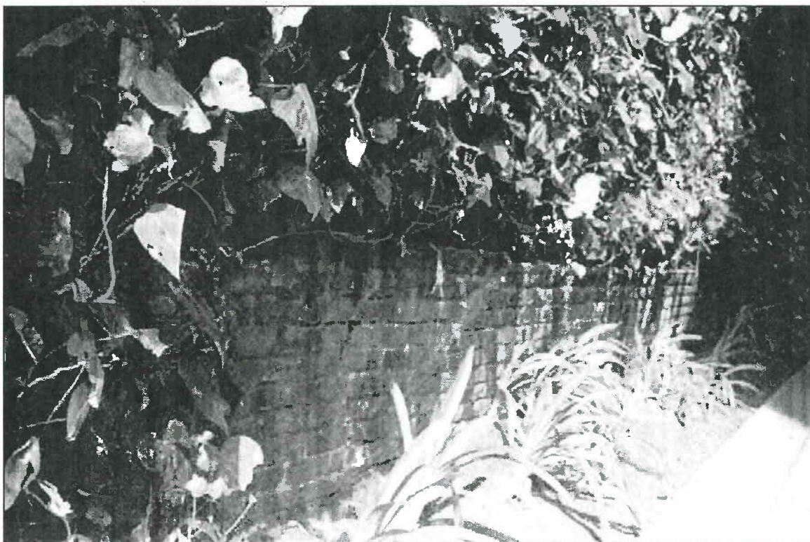
Photo 23. Burr House, 1772 Vallejo Street, 94123. Out of plane URM brick wall west of driveway.
