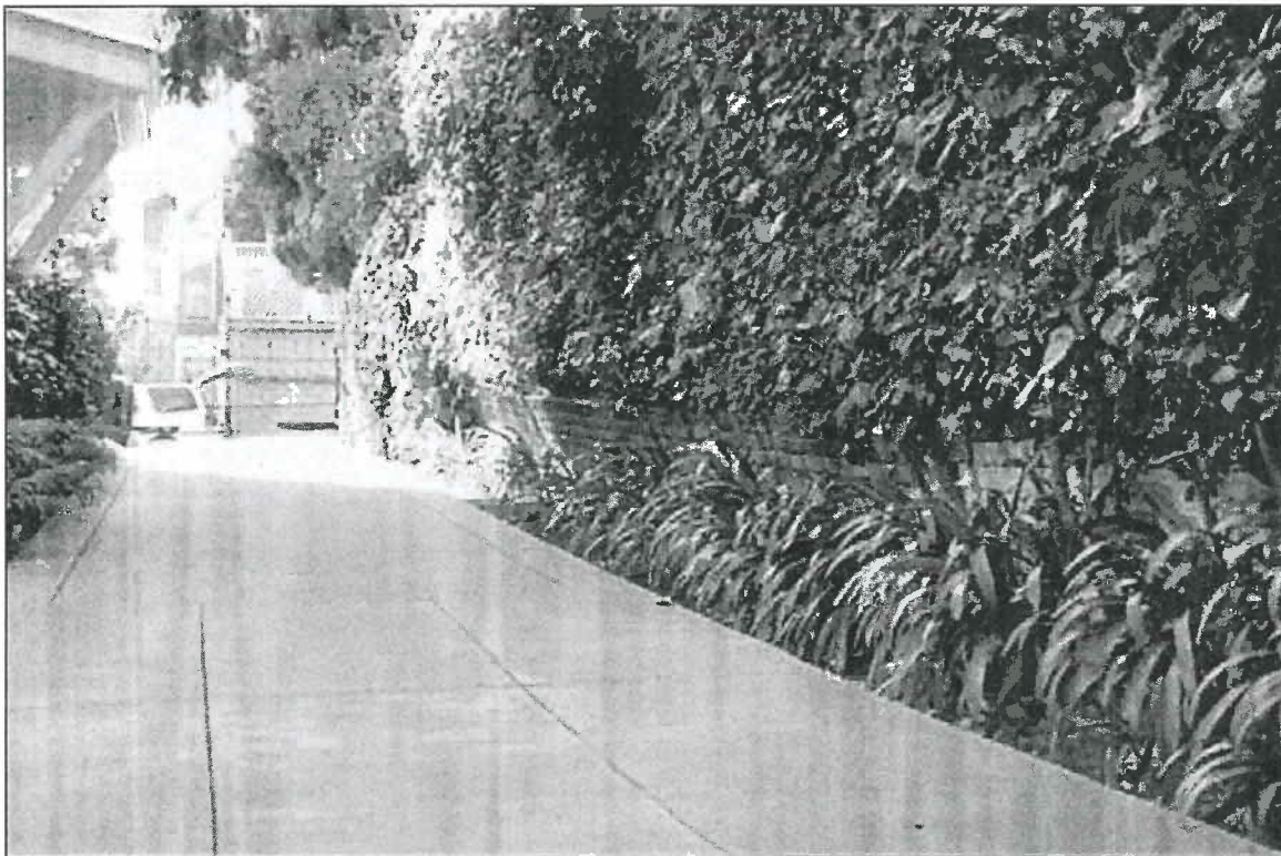
Photo 22. Burr House, 1772 Vallejo Street, 94123. Out of plane URM brick wall west of driveway.
