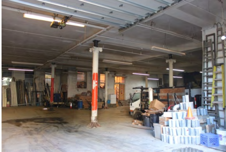
FIGURE 13. CHURCH: BASEMENT SHOWING GUTTED CONDITION, 2015.
