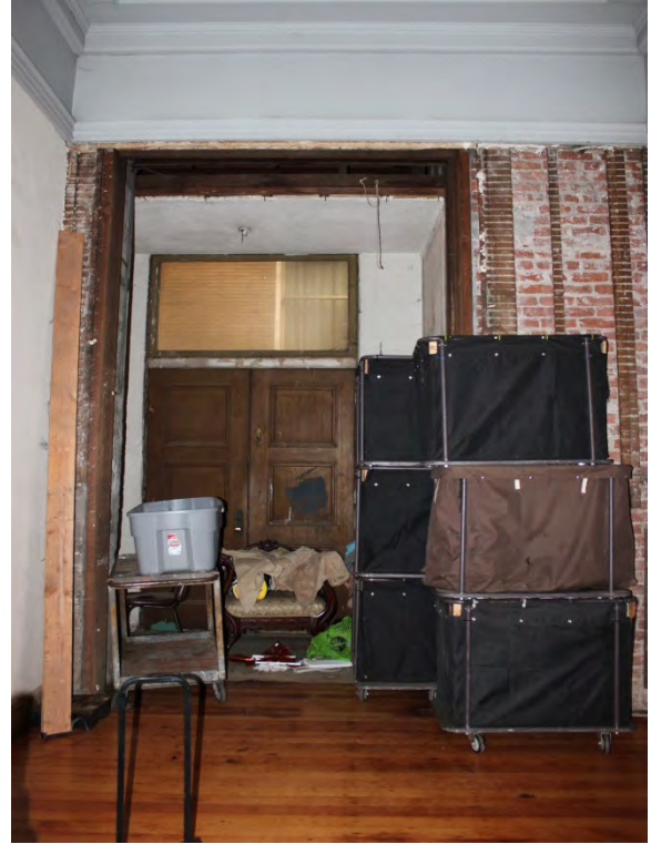
FIGURE 17 (RIGHT). CHURCH: BAPTISTRY SHOWING PARTIAL REMOVAL OF WALLS AND DOOR TO INTERIOR ALLEY, 2016.
