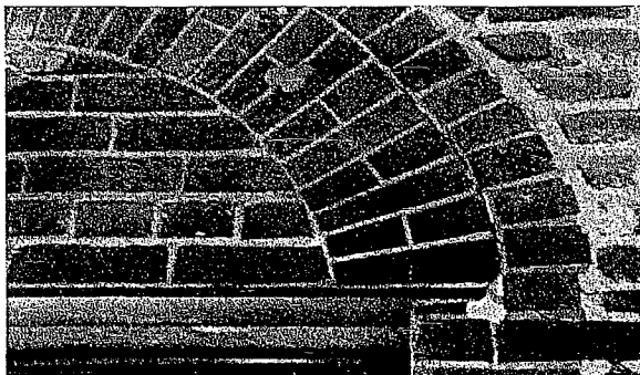
Figure 113 Detail view of cracked mortar and brick around window openings (photograph taken on 04/10/2017).
