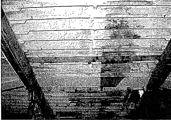
Figure 103 Photograph of ground floor ceiling joists. Note ghosts from old HVAC and water staining (photograph taken on 04/04/2017).
