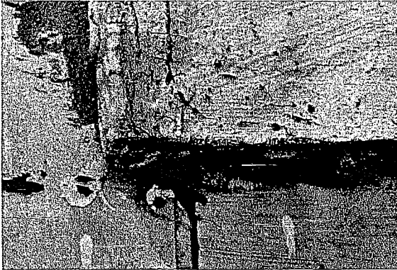
Figure 47 Detail photograph of roof waterproofing construction. Materials include tar, sheet metal, and titanium synthetic underlayment (photography taken on 04/05/2017).
