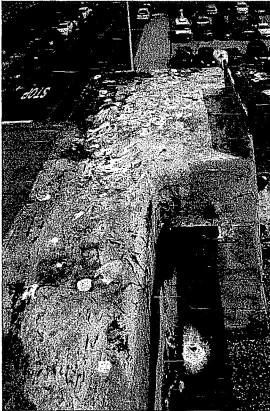
Figure 51 Photograph of the northeast corner and horizontal surface on parapet. Note biological colonization, corrosion, atmospheric pollution, and animal deposits (photography taken on 04/04/2017).
