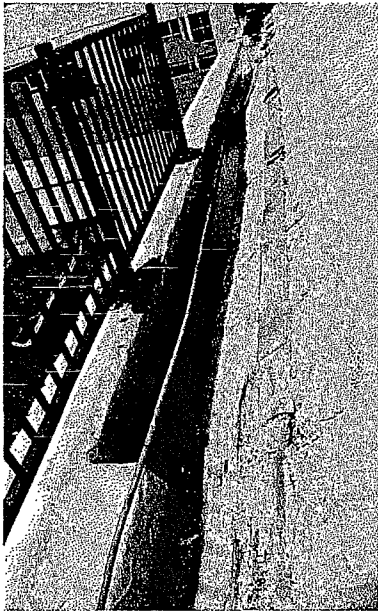
Figure 39 Detail photo of drainage condition along the south parapet. Note standing water (photography taken on 04/05/2017).
