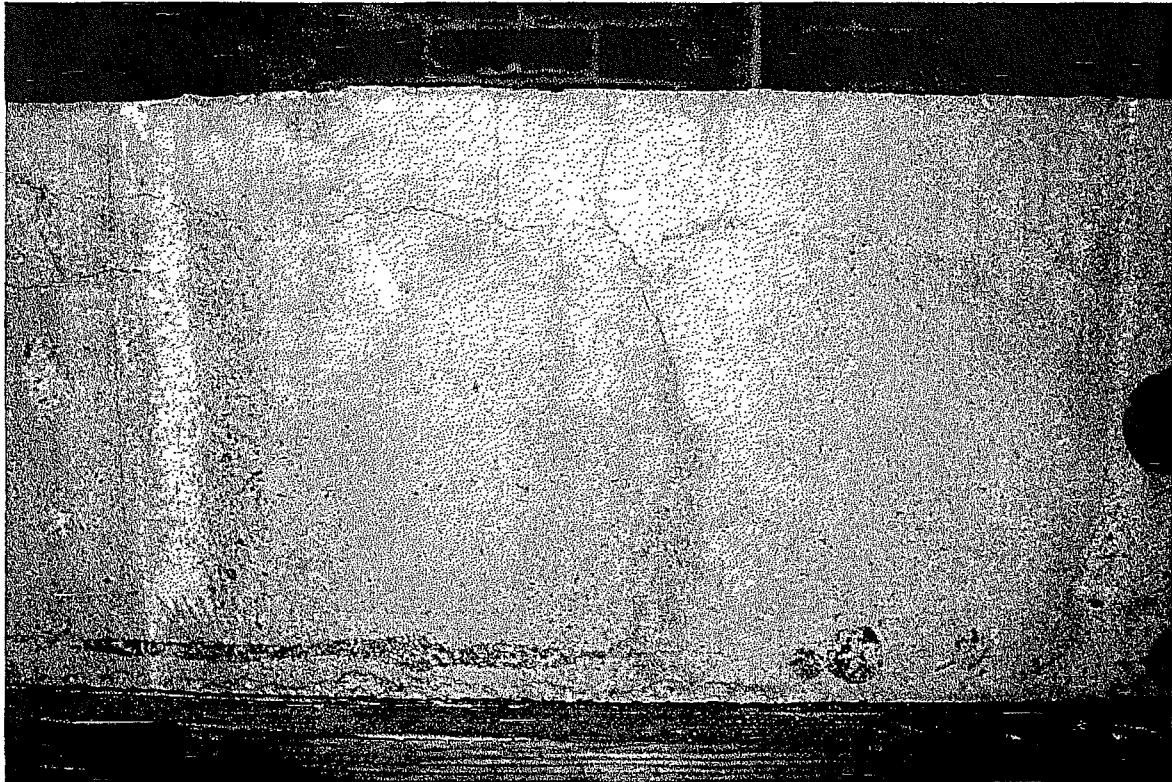
Figure 131 Detail view of cracking pattern found in the reinforced concrete member on the upper story. Note through-cracking: the crack runs the height of the beam and run perpendicular to its width all the way to the exterior brick wall. Stabilization of these structural member has been attempted with thin wooden planks. Also note bolt (right) from steel tie-back, which anchors the exterior walls to the reinforced concrete members (photograph taken on 04/05/2017).
