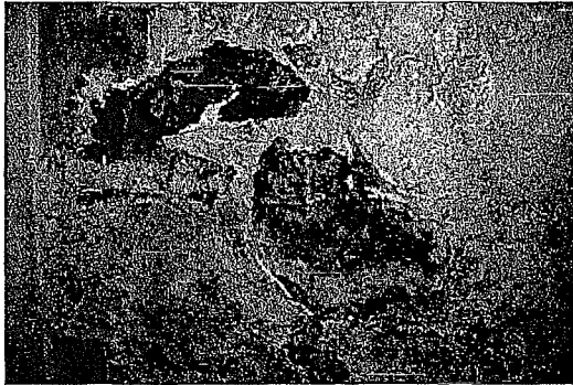
Figure 75 Detail photograph of north foundation condition. Note lost finish, exposed stone, and extensive efflorescence (photography taken on 04/04/2017).
