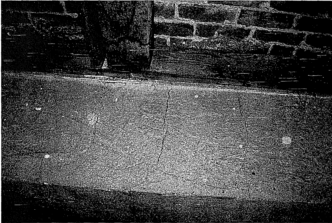
Figure 80 Detail of modern lateral stabilization system (concrete beams). Note severe through-cracking of the cement matrix (photography taken on 04/04/2017).
