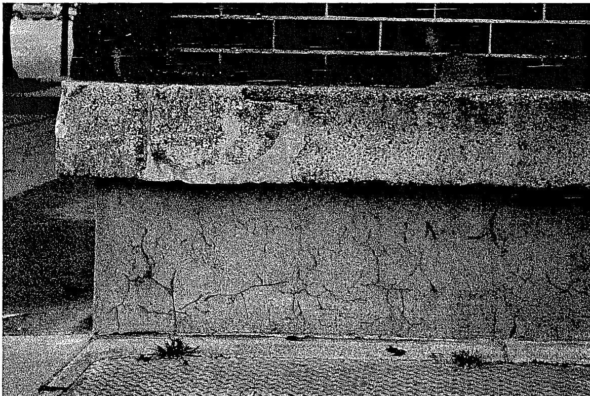
Figure 18 Detail of parging mixture used in the foundation of the Vallejo Street elevation. Note hairline cracking of parging mixture (photography taken on 04/04/2017).
