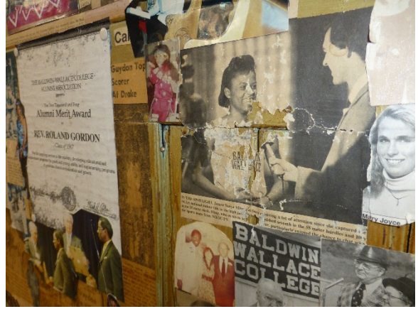
Figure 22: Displacement and movement of wood paneling resulting in attached collage to tear.
