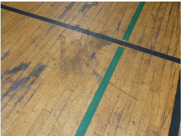
Figure 19: General wear and tear of wood floors from pedestrian traffic.
