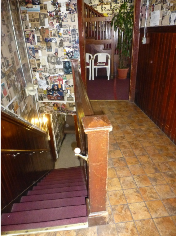
Figure 23: General wear and tear of collage and wood stair railing from pedestrian traffic.
