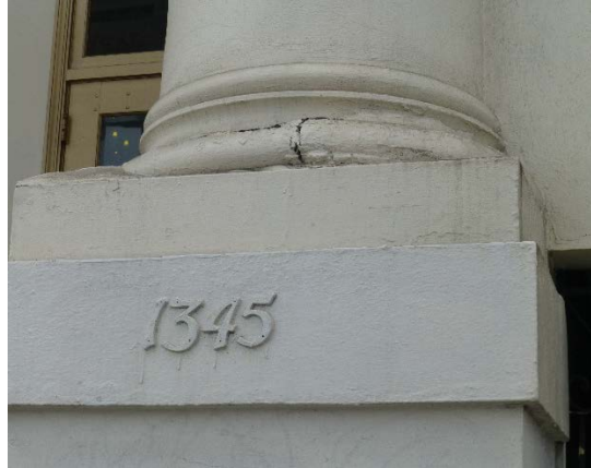
Figure 2: Cracking of concrete column at base.
