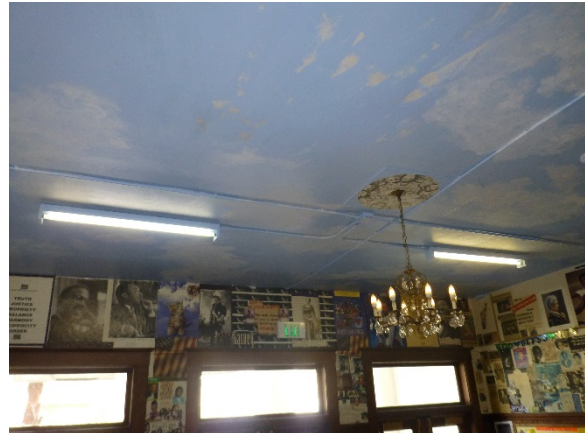
Figure 8: Collages near the front doors experience general wear and tear from pedestrian traffic and UV-light as well as florescent light damage.
