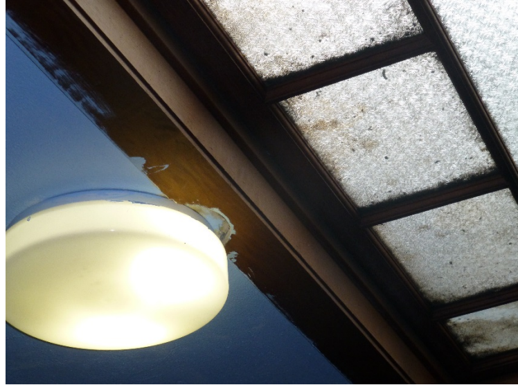
Figure 10: Skylight of textured wire glass has no weatherstripping or putty. Debris has collected on glass. Light fixture cuts into wood frame.
