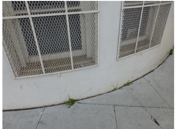
Figure 4: Biogrowth at base indicates possible inadequate drainage.
