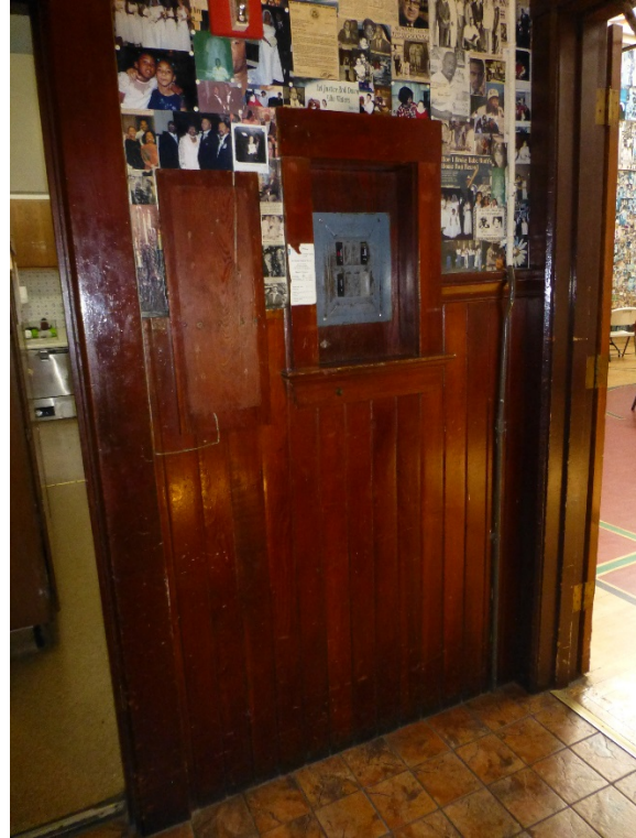
Figure 24: General wear and tear of wood wainscoting from pedestrian traffic.
