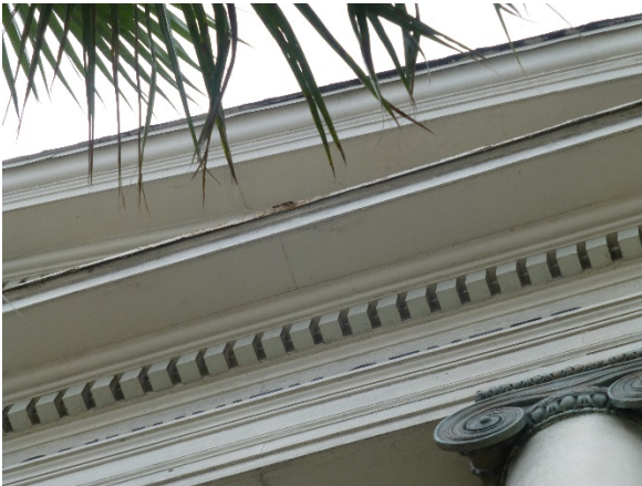
Figure 3: Staining and cracking at roofline suggest roofing issues.
