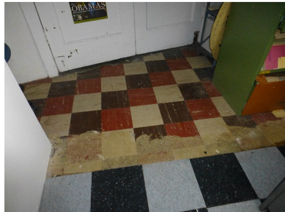
Figure 28: Exposure of multiple layers of flooring.
