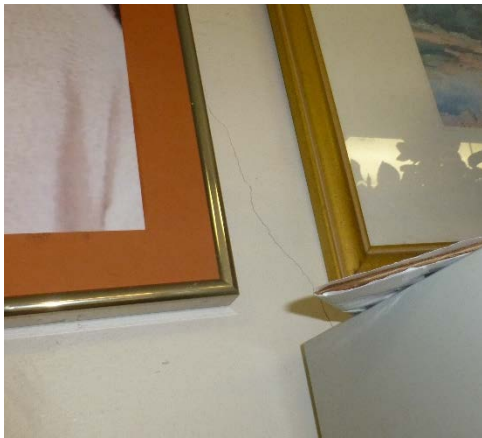
Figure 14: Cracking of plaster wall.
