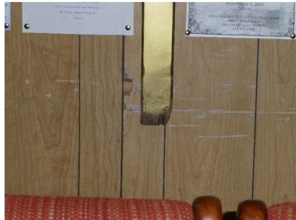
Figure 16: Ends of gold crucifix have missing paint. Wood paneling has abrasion marks from furniture.
