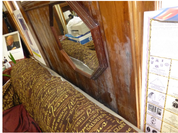
Figure 32: Water damage to wood paneling between windows.
