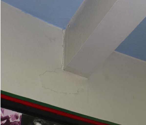
Figure 29: Detail of cracking at ceiling beam.
