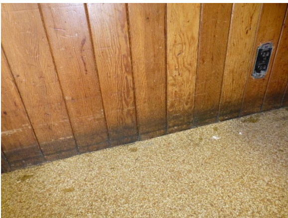
Figure 13: Abrasion marks and soiling at base of wainscoting from pedestrian traffic.
