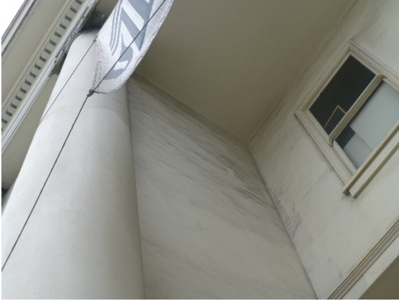
Figure 1: Portico ceiling and walls have general soiling and staining.
