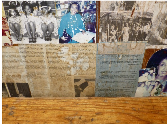
Figure 18: Detail of water damage on collage behind wood bench.
