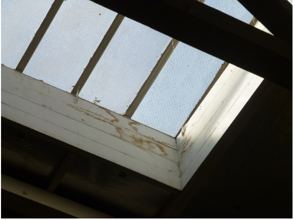
Figure 21: Water damage to wood paneling near skylight.
