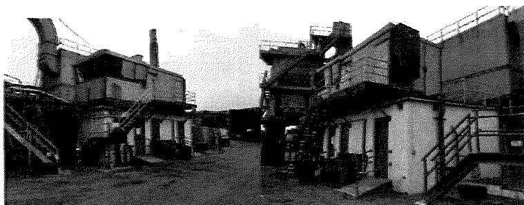
Electrical Power Room (bottom) and Control Room (top), northwest facing elevations (left) and southwest facing elevations (right)
