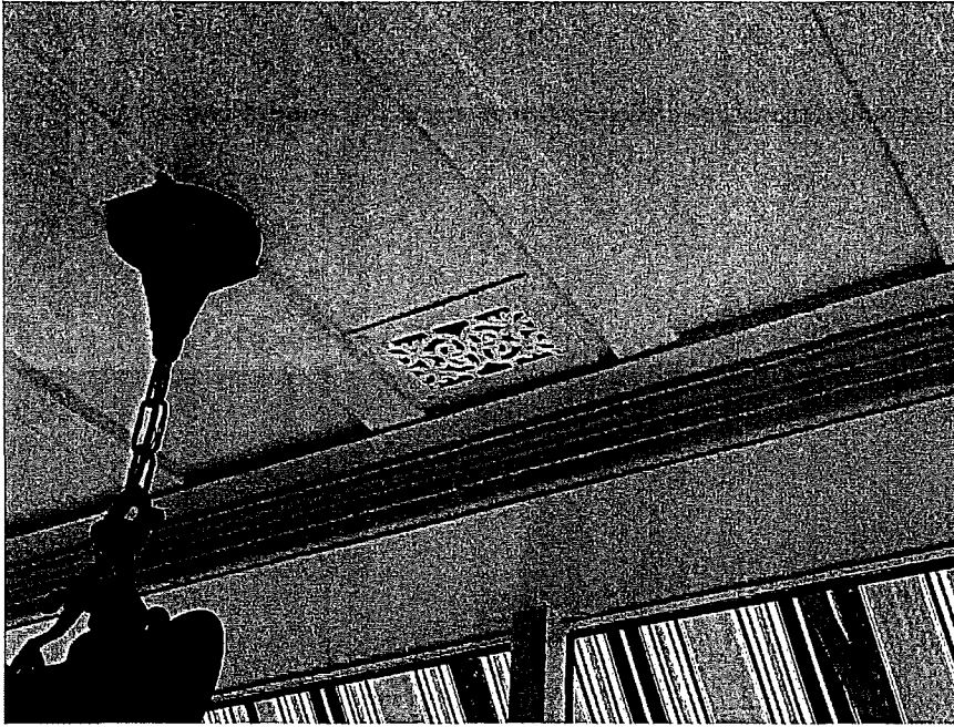
Figure 40 A detail of the wood ceiling moldings and a vent in the front window of 198 Gough Street.
