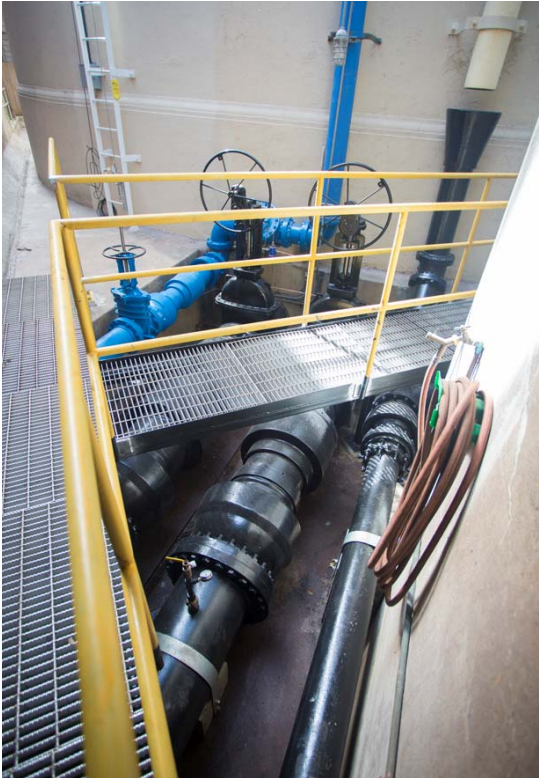
Jones Street Tank, new piping and walkway
