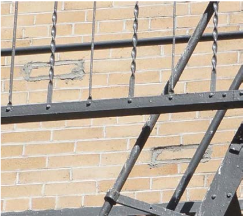
17-29 Third Street - Limited locations of mismatched mortar
