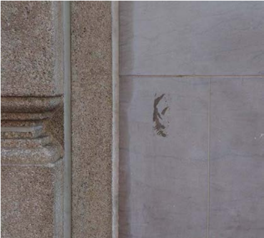
Hearst Building – Minor residue at marble podium
