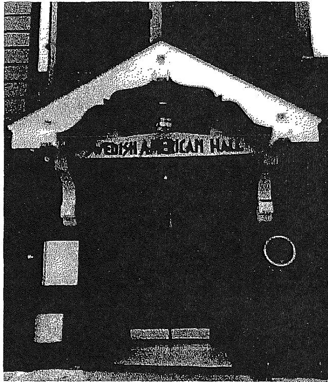
Main entry showing doors to be replaced.
